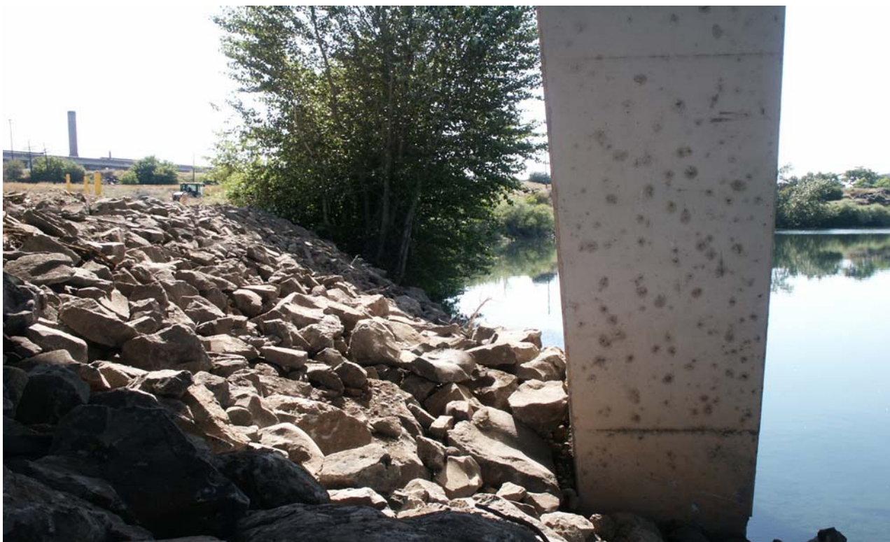
View of new riprap on stabilized river bank (looking west under bridge).
