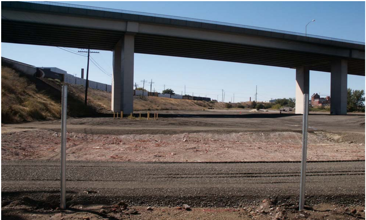
View of southeast detention basin and top course (looking west from Erie Street).
