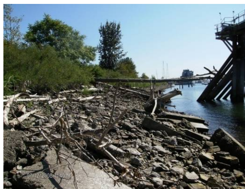
Photograph 32: Concrete and woody debris
