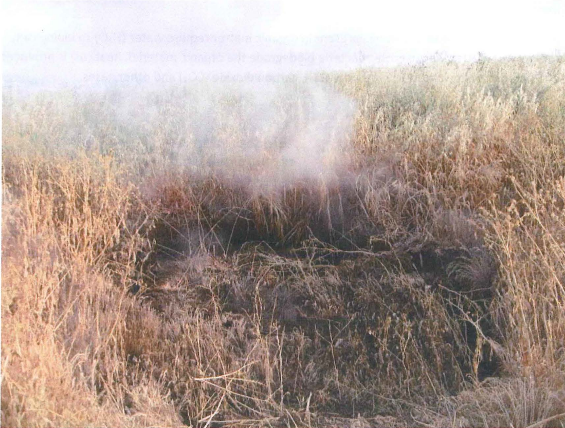
Photo 2. Typical sinkhole at a solid waste landfill caused by a subsurface smoldering event (Source: Todd Thalhamer)
