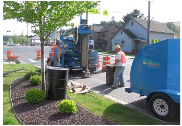
Photograph 2. View looking southwest toward boring B26, completed as monitoring well MW26, located in the right-of-way along the east side of North Main Street adjacent to the Time Oil property.
