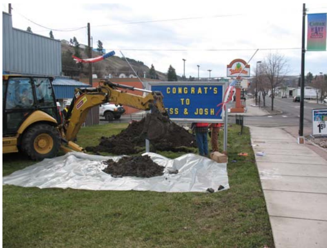
Photograph 11. View of the excavation of TP01 looking south along the west side of the Colfax Grange Supply Company building along North Main Street.
