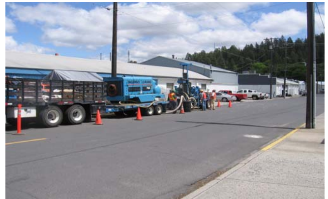
Photograph 10. View of the installation of MW32 looking northeast toward the Colfax Grange Supply Company building along East Harrison Street.
