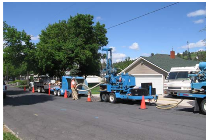
Photograph 12. View of the installation of MW31 (an off-site well) looking northeast along North Morton Street.
