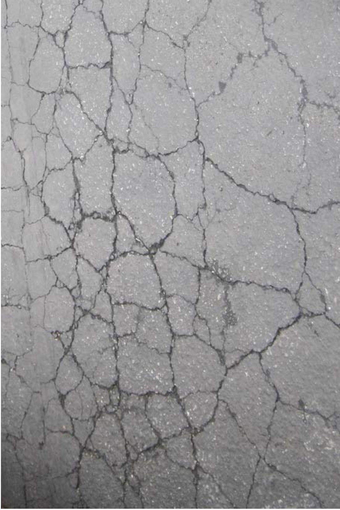
Photograph 7. Example of pavement “spider” or “alligator” cracks that would warrant additional inspection and repair under the proposed OMMP.
