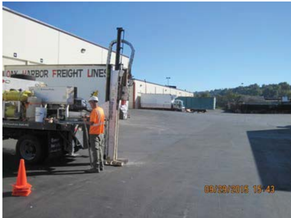
Photograph 2. North central portion of the KIP parcel facing south, during installation of temporary gas probes.
