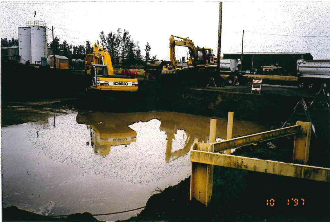
18. Track-hoes continue trying to excavate to 6 feet below ground surface, but standing water complicates the project.
