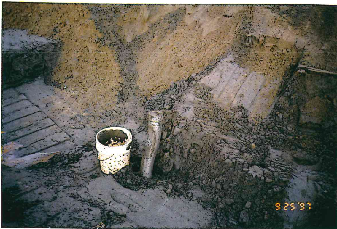
13. Bucket drainage system or dry well discovered near MC-R during excavation procedures.
