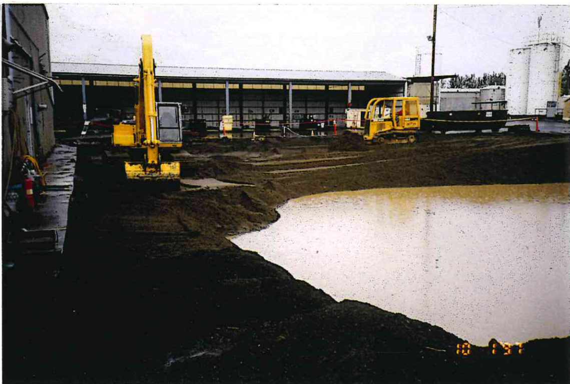
20. Decide not to excavate beyond 6 feet below ground surface to protect the silt confining layer. Fill in excavation with pre-load.
