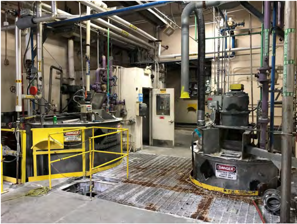
Photograph 5: Subgrade tanks/vault in Make Tank Room
