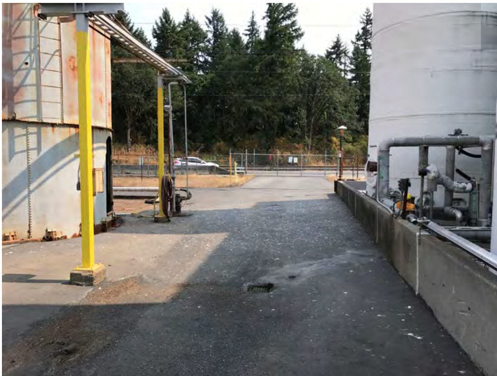
Photograph 4: Drain in tanker loading driveway (SB19 location)
