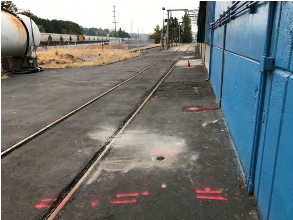
Photograph 1: Rail spur along east side of manufacturing plant building (SB8 in foreground)
