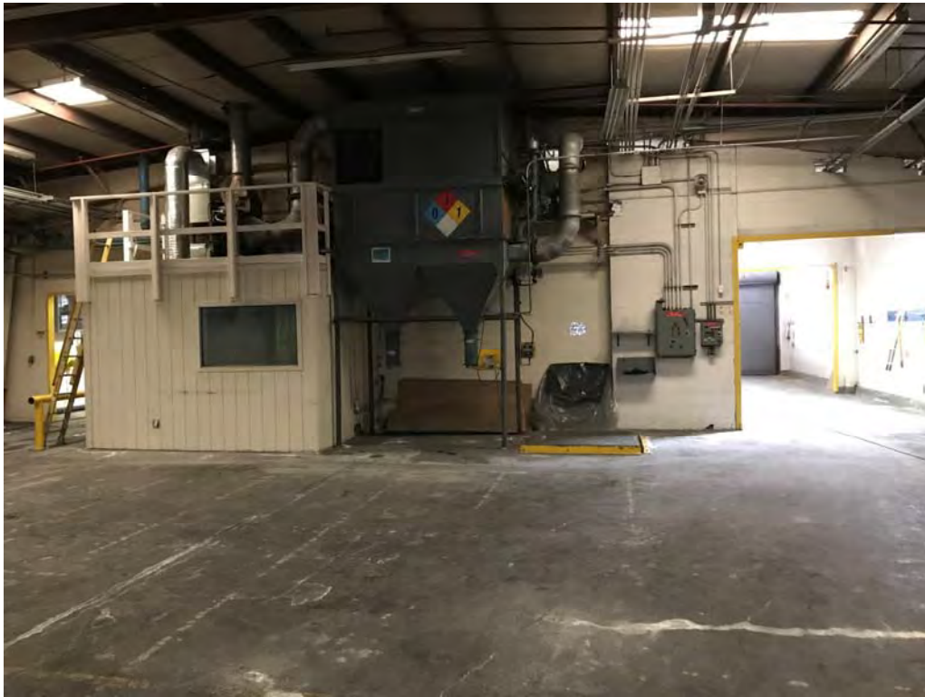
Photograph 3: Baghouse inside manufacturing plant warehouse (SB9 location)
