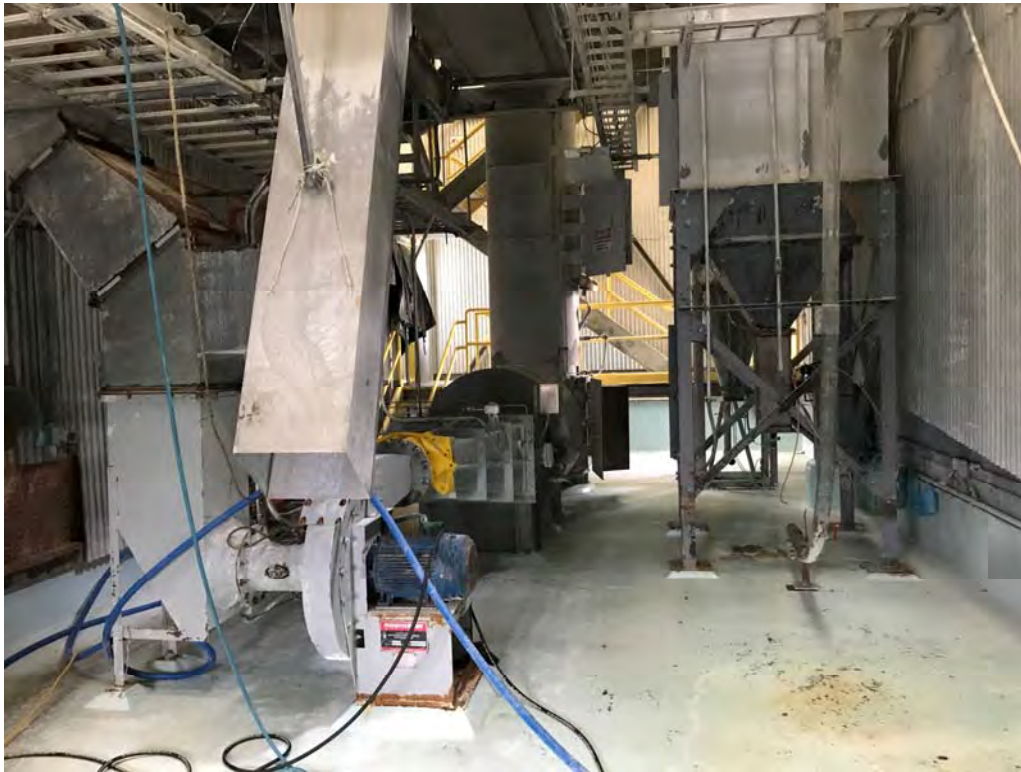
Photograph 9: Zinc Oxide Dryer Room
