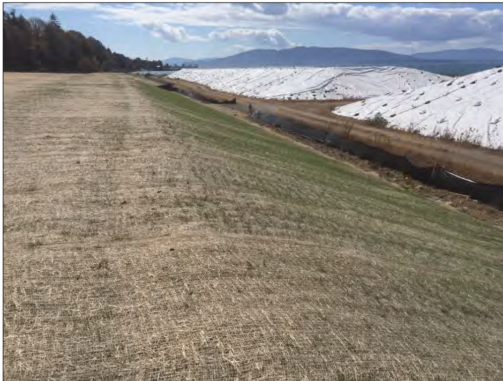
4. Top of pile showing western slope, silt fence visible, grass visible. Loose soil along upstream side of silt fence needs to be graded out and stabilized with grass or some other means.
