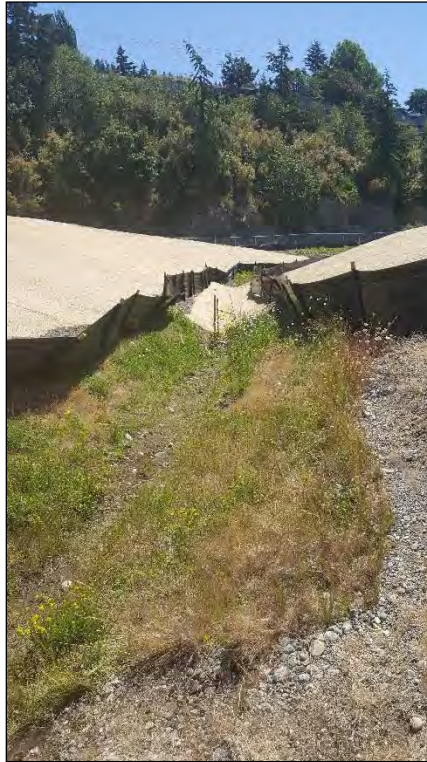
31. Temporary culvert has been removed and area has been covered with erosion control.
