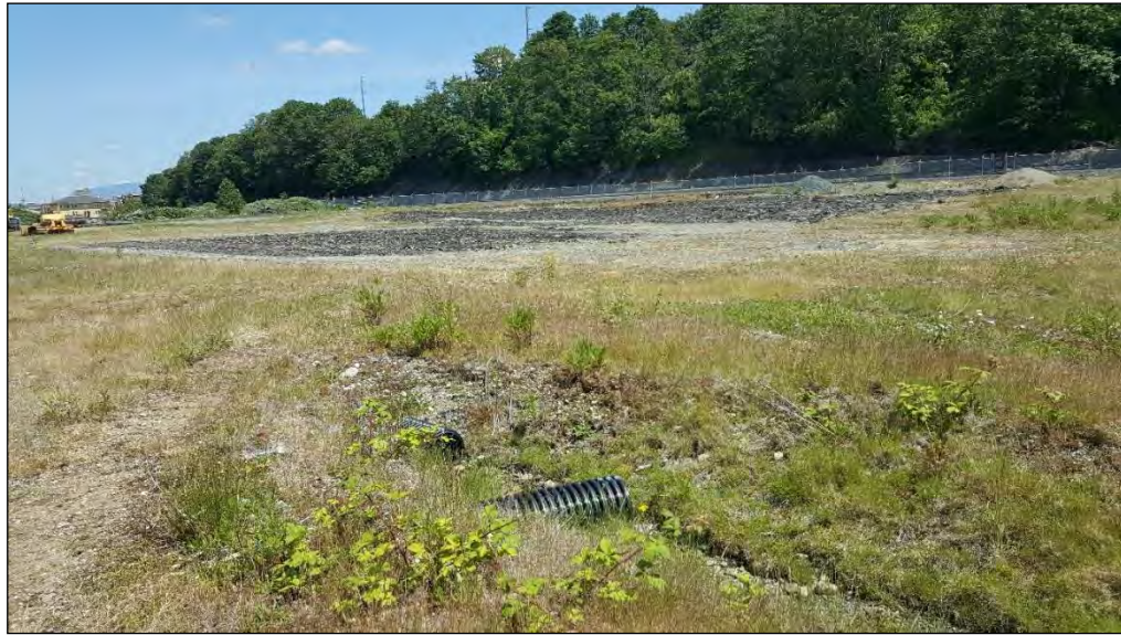
3. Looking north from southwest end of site. Asphalt has been ripped and vegetation has been mulched and left in place.
