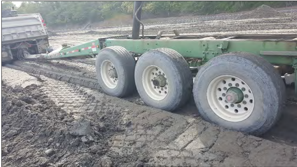
18. Trucks getting stuck in compacted fill material.
