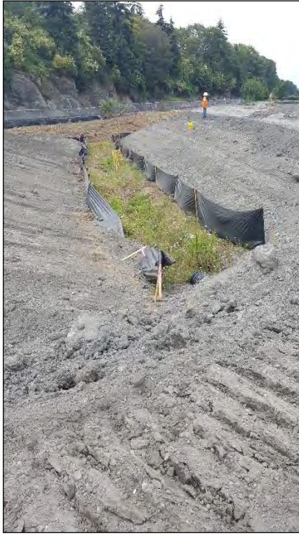
17. Silt fence has fallen down. MTC technician in background.
