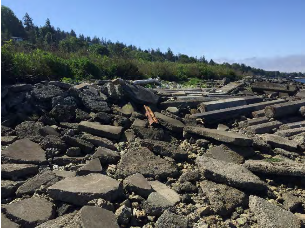
Photograph 9. Extensive coverage of angular concrete below the MHHW within the middle of the Site.
