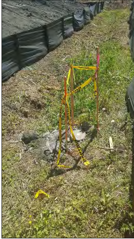
14. Destroyed settlement survey monument SSM-5 has been replaced.
