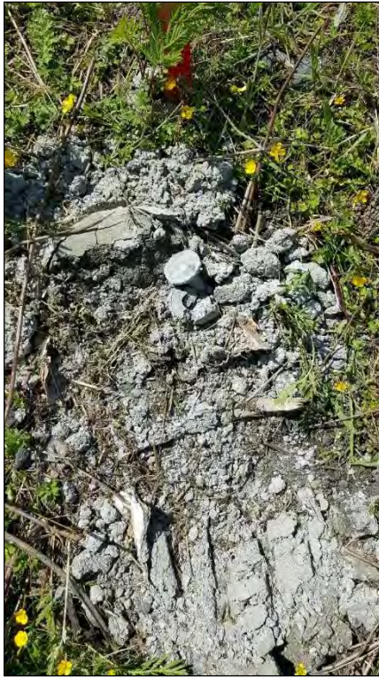
1. Destroyed settlement survey monument SSM-5.
