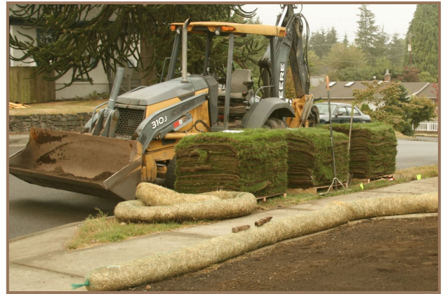
Stacked sod is staged and ready for placement in a front yard in Tacoma.
