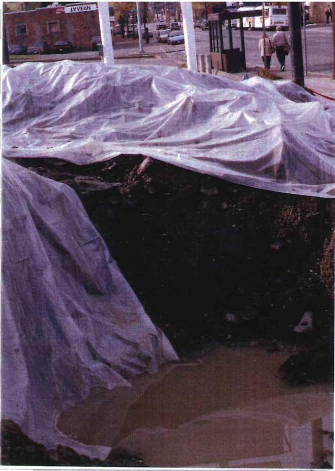
5. Water in excavation pit and stockpiled soils. 6. Excavation along Rainier Avenue South.
