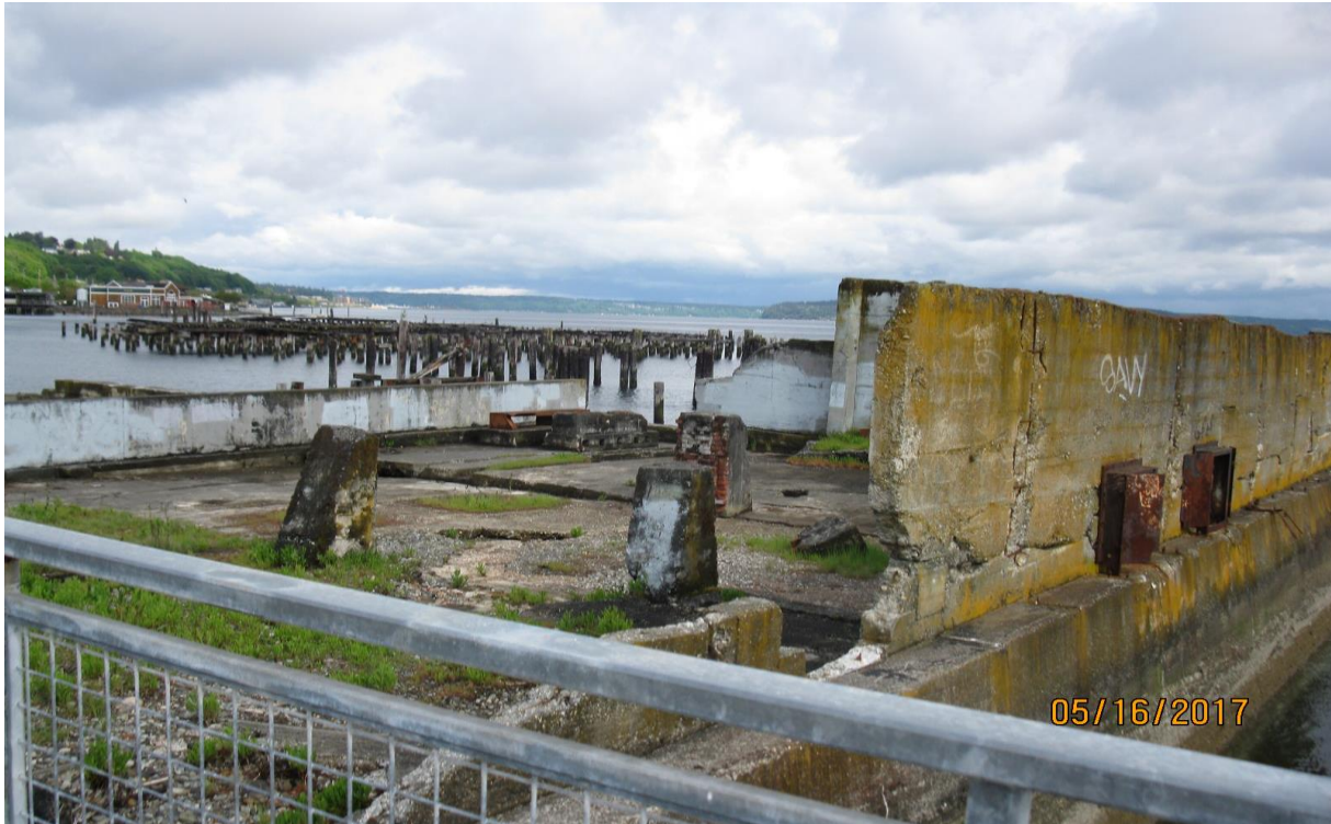
Photo 7: Remaining Mill Building/Foundation and Pilings in the Commencement Bay – from the Southeast
