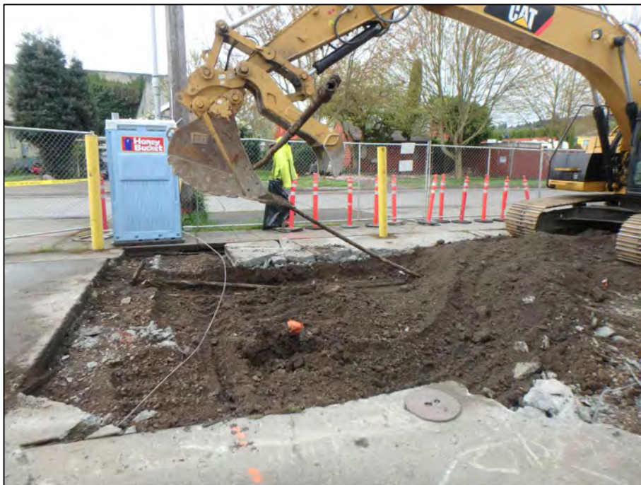
Photograph 6: Uncovering and removal of three former product lines between the USTs and the former pump island in the South Yard.
