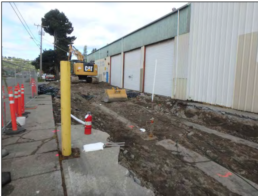
Photograph 10: Photograph showing the interting of UST1 in the South Yard with carbon dioxide. CO 2 tanks were located east of the excavation.
