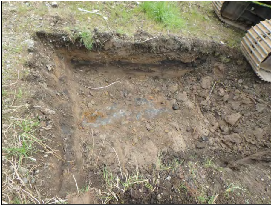
Photograph 5: Top of the residential heating oil tank located on the eastern portion of the Site. The top of the tank was approximately 2 feet below ground surface.
