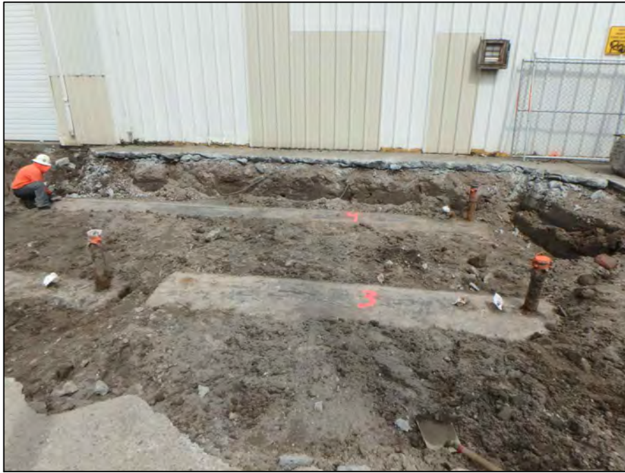
Photograph 7: View of UST3 and UST4's fill ports which were covered by concrete and uncovered during excavation. UST4 is north of UST3 and south of the current warehouse building.
