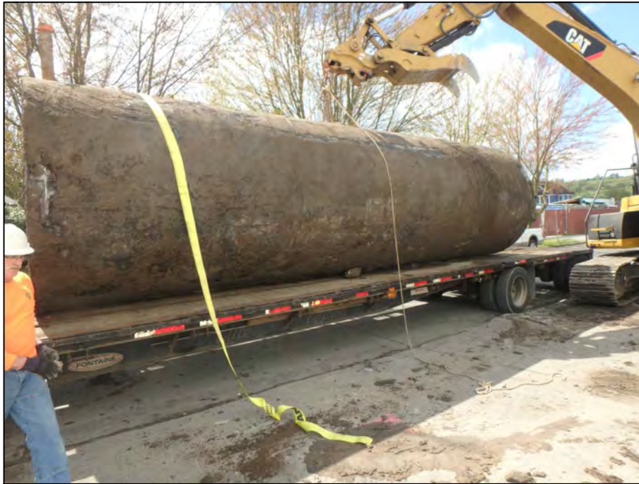
Photograph 15: Side view of UST2 on the truck prior to being transported off-Property. No obvious signs of holes or other evidence of release from UST2 was observed.
