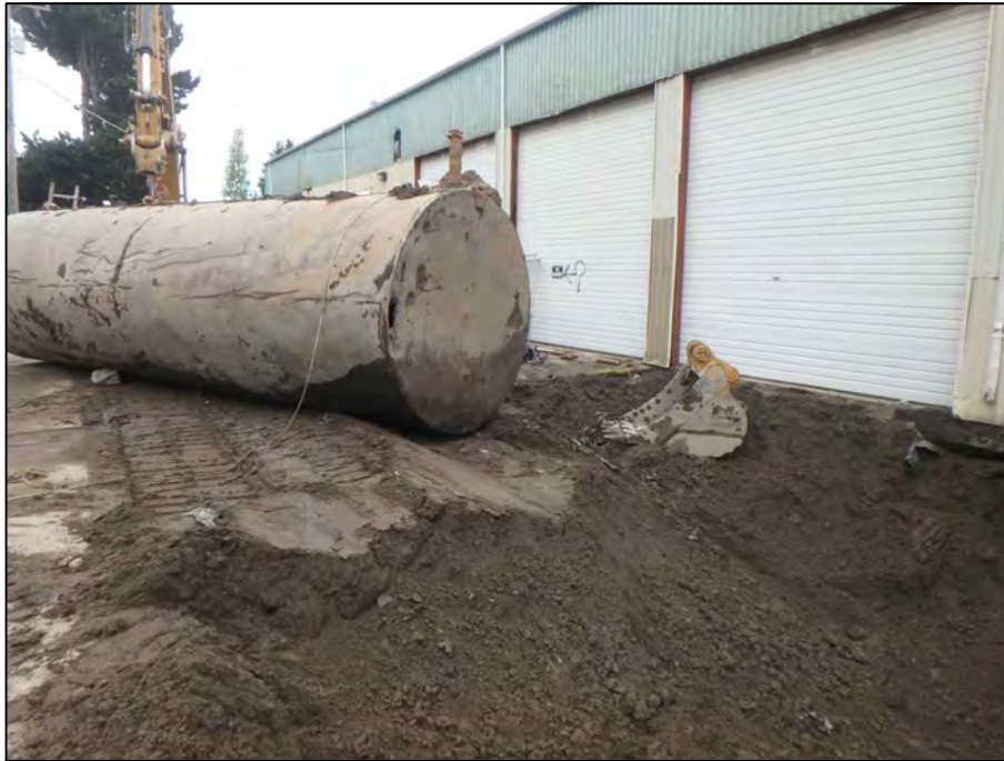
Photograph 11: View of a hole observed in the eastern sidewall of UST4 caused by the excavator during removal. No release of fluids was observed.
