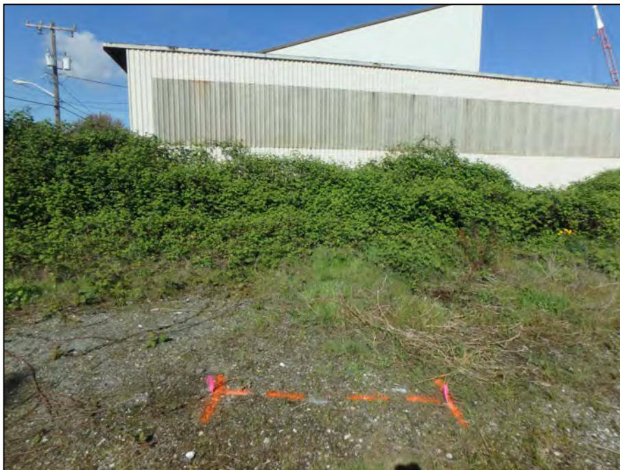
Photograph 2: View looking west at the residential heating oil tank (RT) excavation, which was situated approximately 35 feet from the eastern edge of the warehouse.
