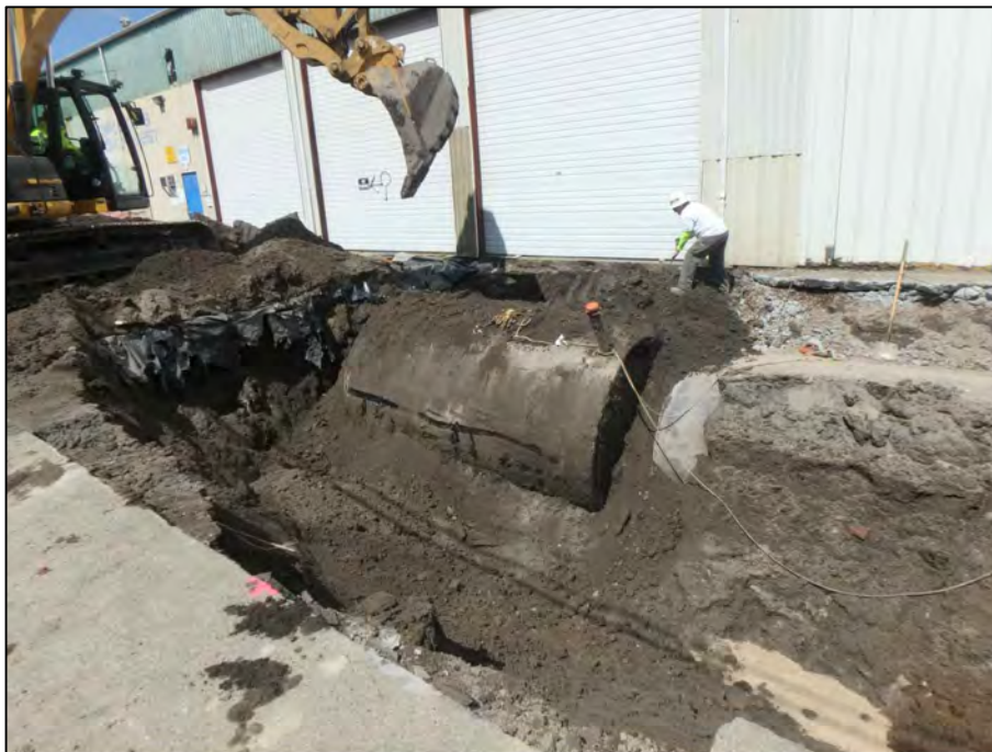
Photograph 12: Location of UST1 in the fuel tank nest located in the South Yard on the Property.
