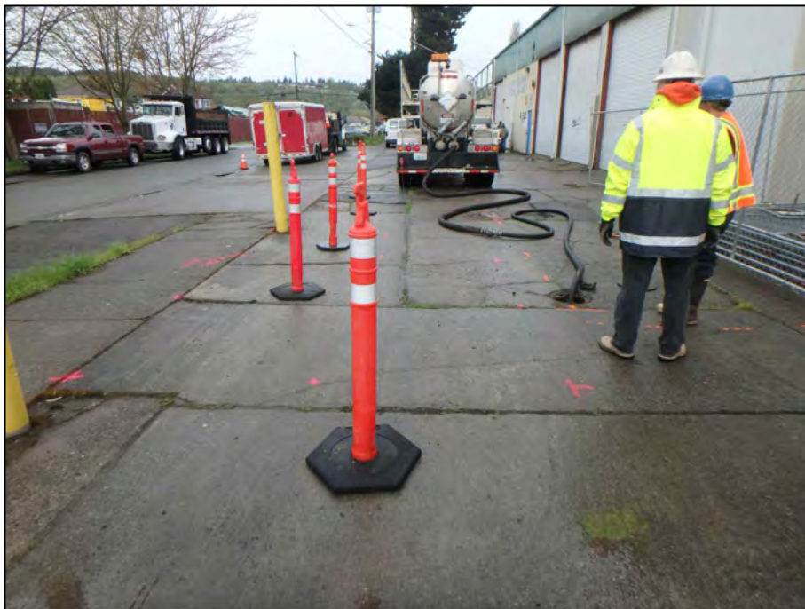
Photograph 4: View looking west at the South Yard excavation location while the USTs were being pumped of fluid in preparation for their removal.
