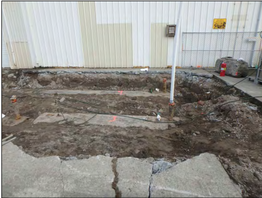
Photograph 9: Photograph of the interting of UST3 in the South Yard with carbon dioxide. CO 2 tanks were located east of the excavation.
