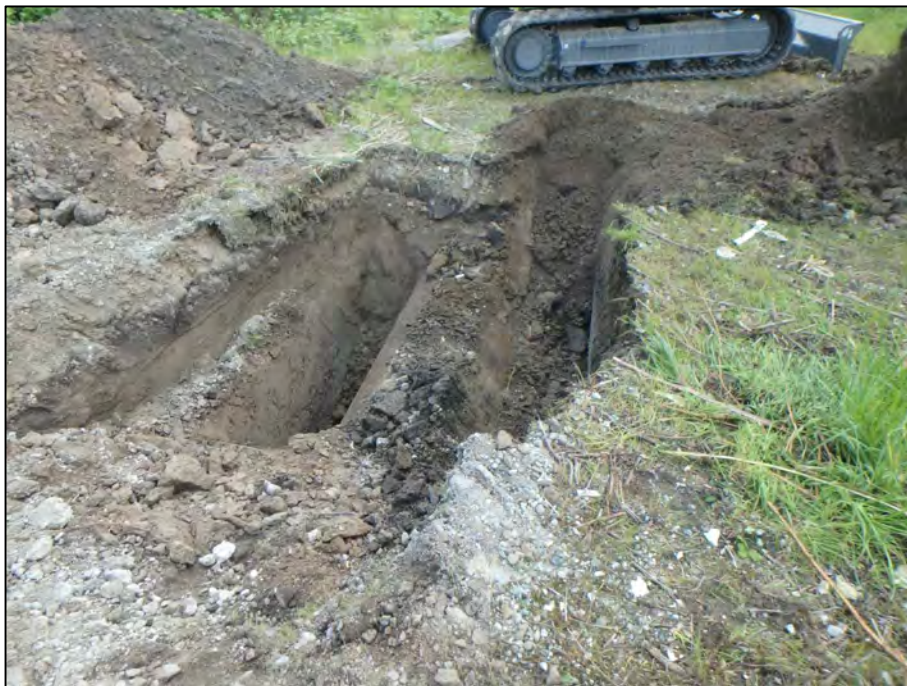
Photograph 18: View of the surface above UST5 (residential heating oil tank) during the excavation.
