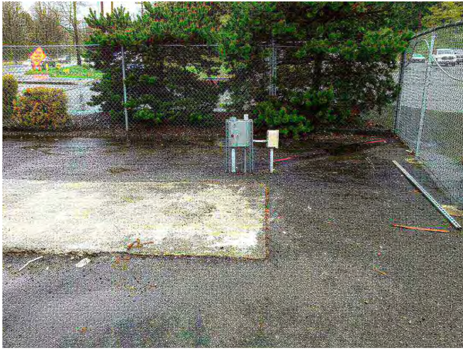
Electrical lines along perimeter fence
