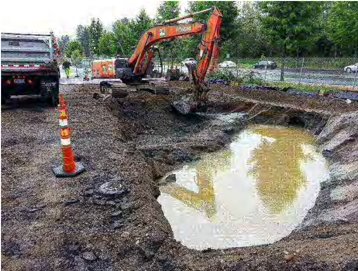
Photo #5. The leaking storm water pipe flooded the remedial excavation.
