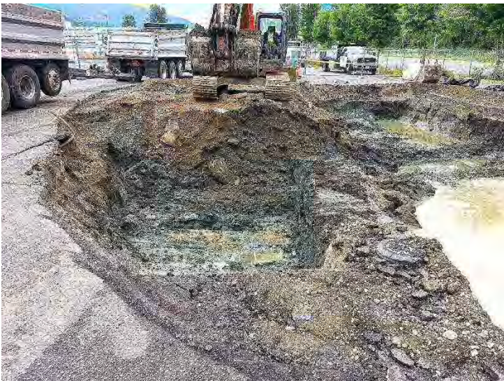
Photo #6. Impacted soil continued to be removed using temporary soil berms to retain the storm water pipe water.
