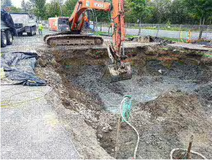
Photo #7. A sump was installed in the remedial excavation to extract water for treatment and subsequent permitted disposal to the King County sanitary sewer system.
