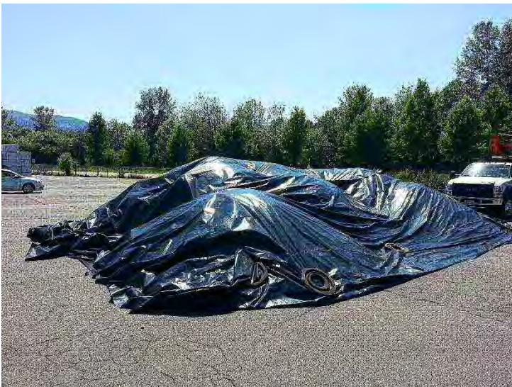
Photo #3. The stockpiled clean overburden soil was returned to the excavation following the remedial action.
