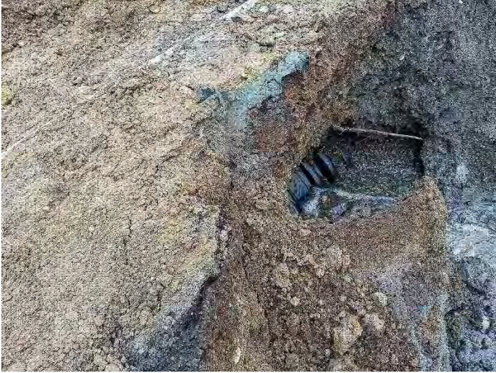
Photo #4. A 24-inch PVC storm water pipe was encountered along the west side of the remedial excavation. The pipe was not damaged by the excavator, instead water appeared to be leaking from a faulty pipe joint.
