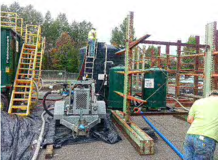
Photo #9. Dewatering effluent was treated with a sand filter and activated carbon, sampled and analyzed for TPH and BTEX, and discharged to the sanitary sewer under a King County permit.
