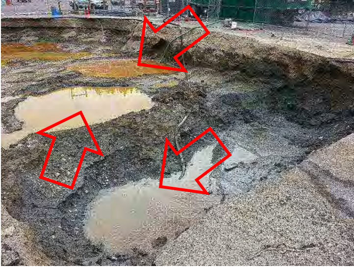
Photo #10. Rectangular-shaped areas that had been backfilled with pea gravel are assumed to be the former location of the three USTs removed in 1989.
