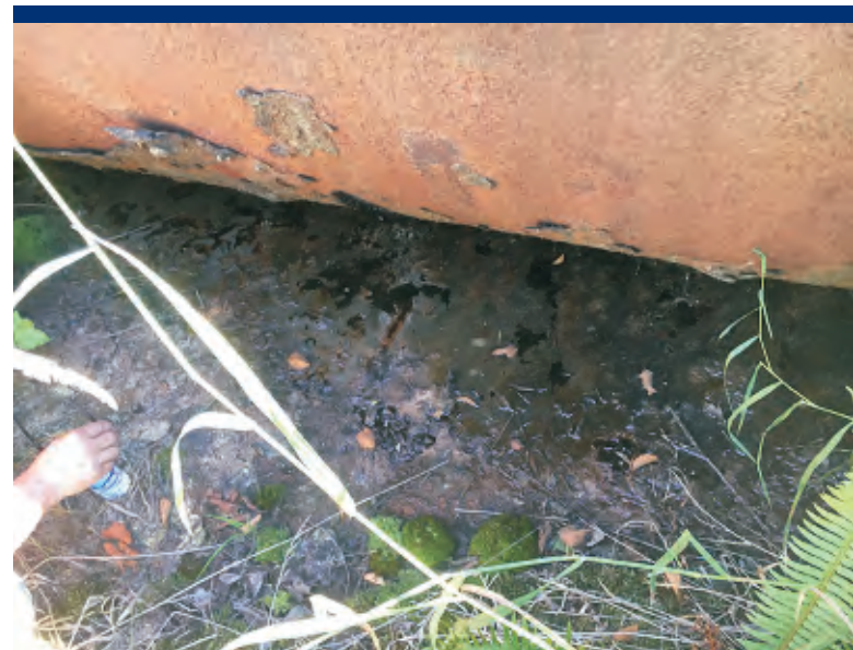
Photo 48 Visible oil pool under Tank 50.
