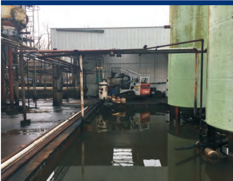
Photo 24 Water in Secondary Containment B that requires removal prior to pumping crude glycerine from tanks.
