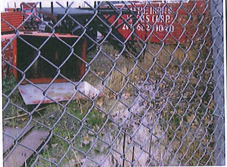
#2. DESCRIPTION: There are no catch basins or storm drain systems on the site. Stormwater run-off sheet flows to a low point and then through the chain link fence and onto the unpaved shoulder of S. Myrtle Street.
