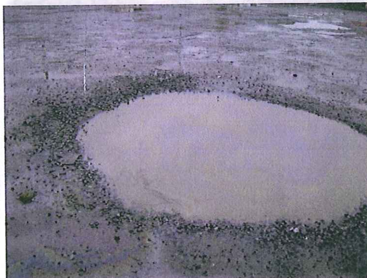
#12. DESCRIPTION: The petroleum leak or spill (lower left of photo) was enough to cause a black layer on the nearby puddle. The permit requires leaks and/or spills to be cleaned up immediately.
