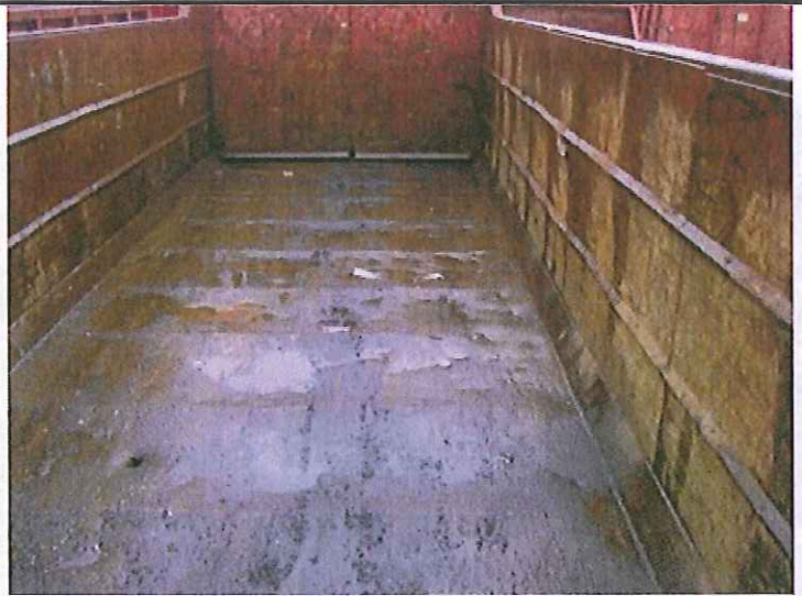
#14. DESCRIPTION: This scrap metal dumpster (drop box) is "empty" but unless it is clean, it must be stored under cover or be fitted with a lid that remains closed when not in use. Stormwater falling into this bin will flush pollutants out of the holes and unsealed ends and onto the ground.
