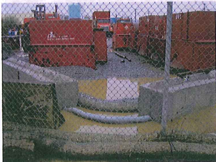
#9. DESCRIPTION: After a brief discussion between Ecology and SIM on January 26, SIM officials installed the ecology blocks to enhance their ability to collect stormwater run-off samples. The sausage booms and straw wattles were not providing adequate treatment of the oily turbid stormwater run-off.
