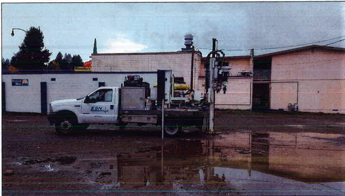
Photo 16. Borehole GP-4 location in progress. Existing site building to left. Looking West.
