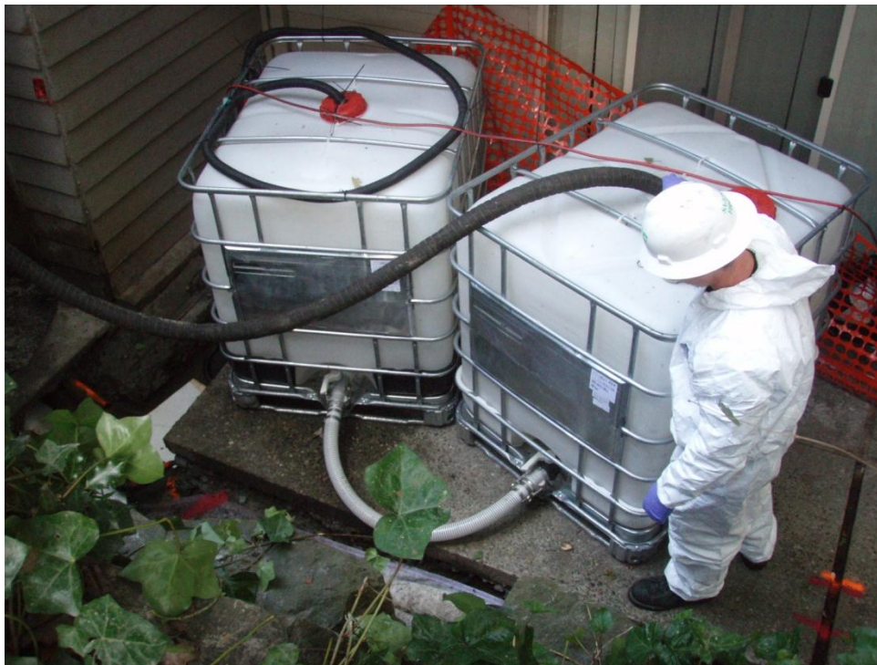
Temporary water storage in poly totes. Totes were emptied using a vacuum truck every two days and the fluids transferred off-site for permitted treatment and disposal between September 1 and 18, 2010.
