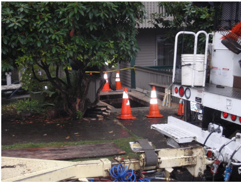
Cones mark access hole cut in top of pedestrian bridge to remove damaged transformer on August 31, 2010.
