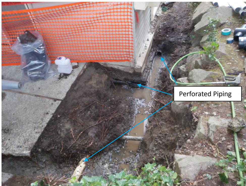
Northwest corner of the building exposing subsurface perforated piping on September 1, 2010.
