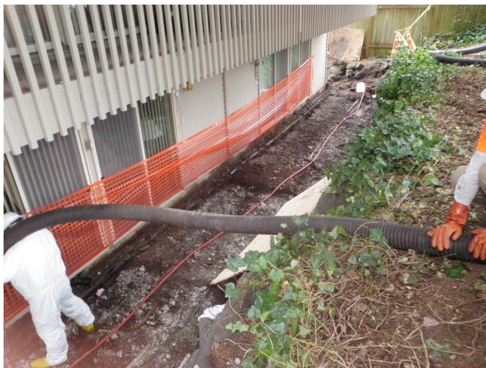
Soil removal using vac-trucks on September 16, 2010 at perforated pipes beneath concrete patio decks.
