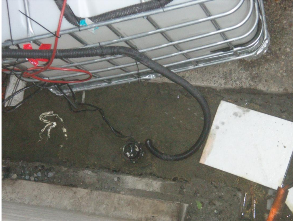
Containment of potentially impacted surface water by pumping to poly totes between September 1 and 18, 2010.
