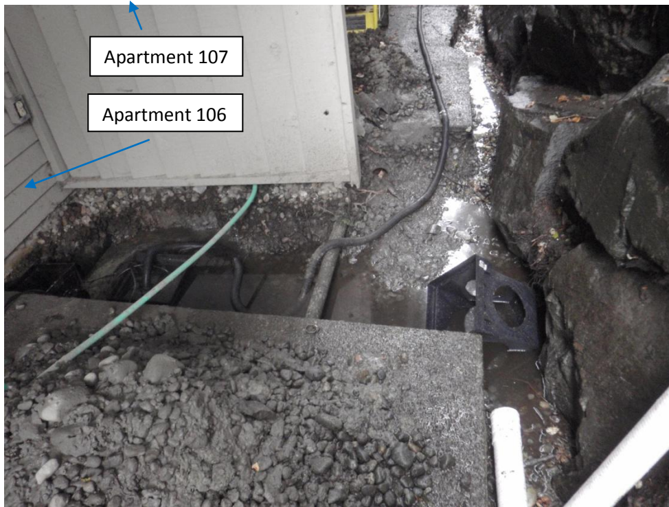
Sump pump used on north side of building for construction dewatering prior to initial spill response activities on August 31, 2010.
