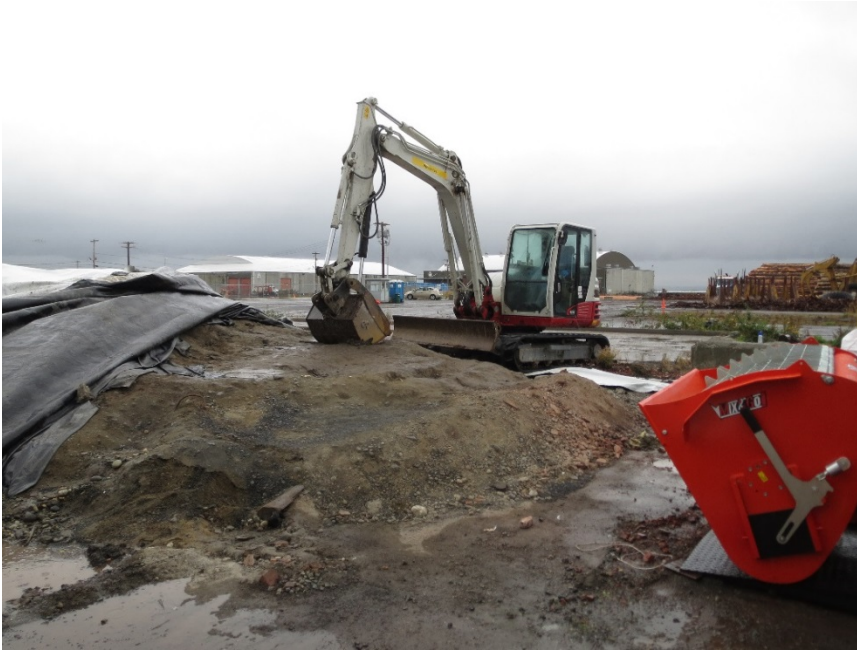
Photo 3. Eastern end of soil/debris pile uncovered, ready to begin loading to mixer.
