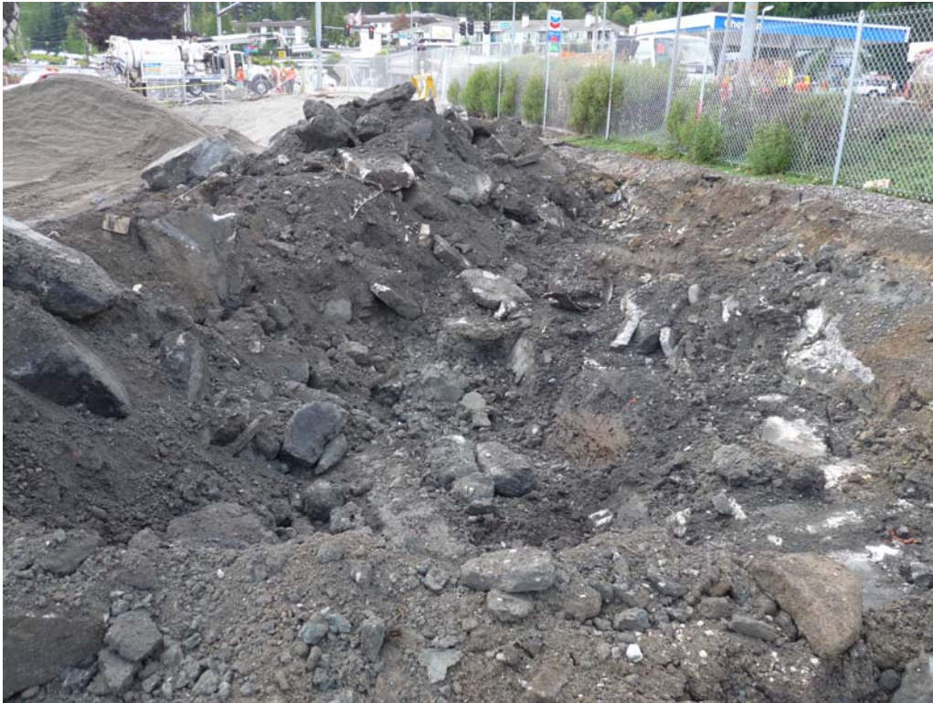
Photo 3 – Concrete and wood debris in north end of excavation (looking to northwest)
