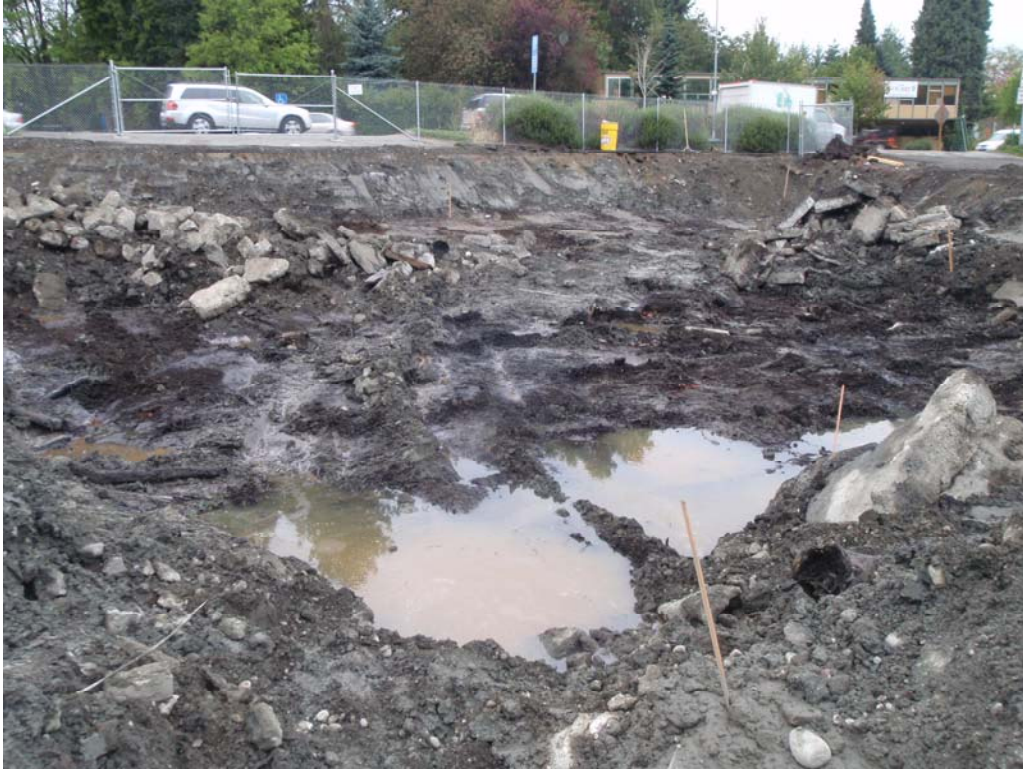
Photo 5 – Peat layer and water table exposed in northern excavation (looking north towards SR 522).
