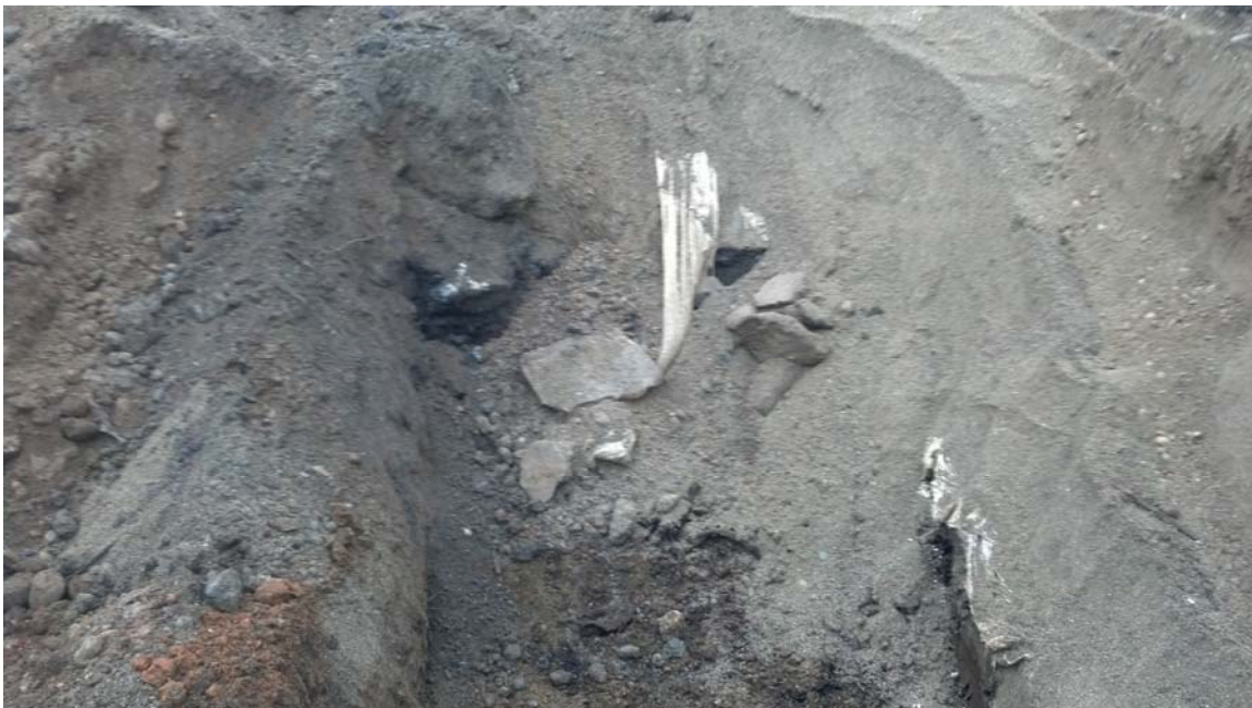
Photo 8 – Exposing liner and ORC from 2010 Interim Action along former SR 522 during October, 2013 remedial excavation.
