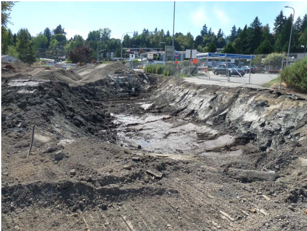
Photo 2 – Looking to northwest. Extent of excavation was limited to maintain the structural integrity of SR 522 and related sidewalk and utilities.
