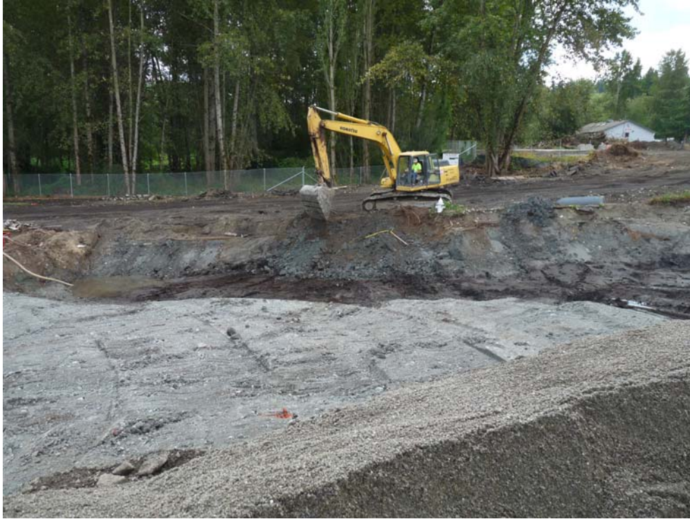
Photo 1 – Excavation limit looking southwest. Note peat layer on excavation floor. Select Borrow fill is being placed into excavation
