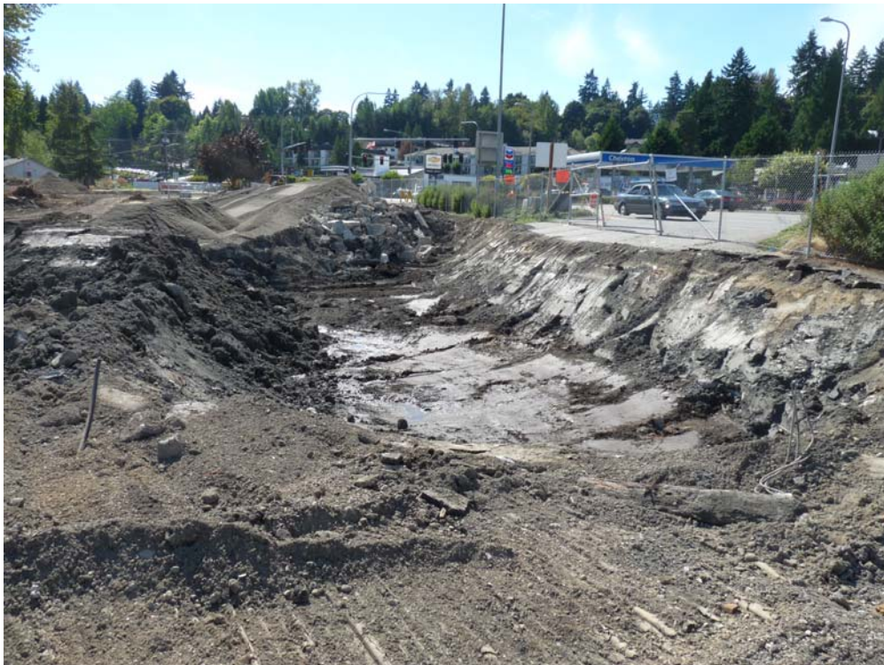
Photo 2 – Looking to northwest. Extent of excavation was limited to maintain the structural integrity of SR 522 and related sidewalk and utilities.
