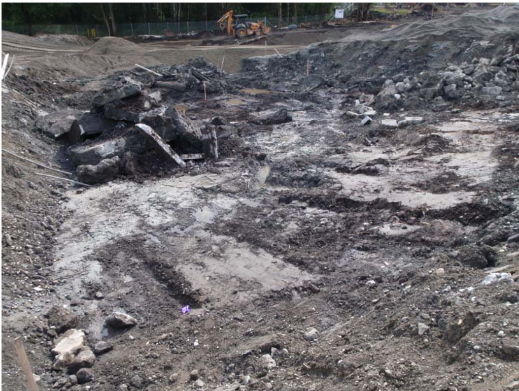
Photo 4 – Concrete and wood debris in north end of excavation (looking to south).
