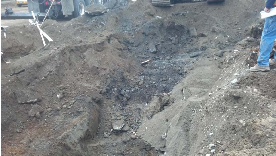
Photo 9 – Debris and fill encountered along former SR 522 during October, 2013 remedial excavation.
