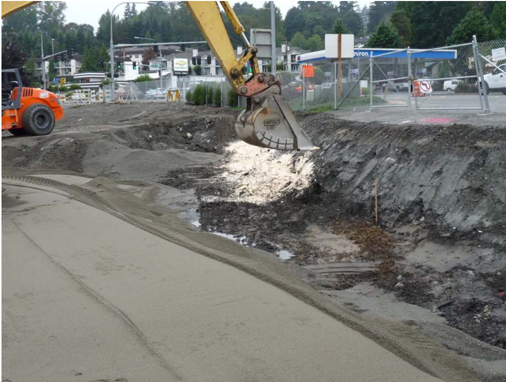
Photo 7 – Placing ORC on northern sidewall along SR 522 before backfilling excavation with Select Borrow seen in foreground.
