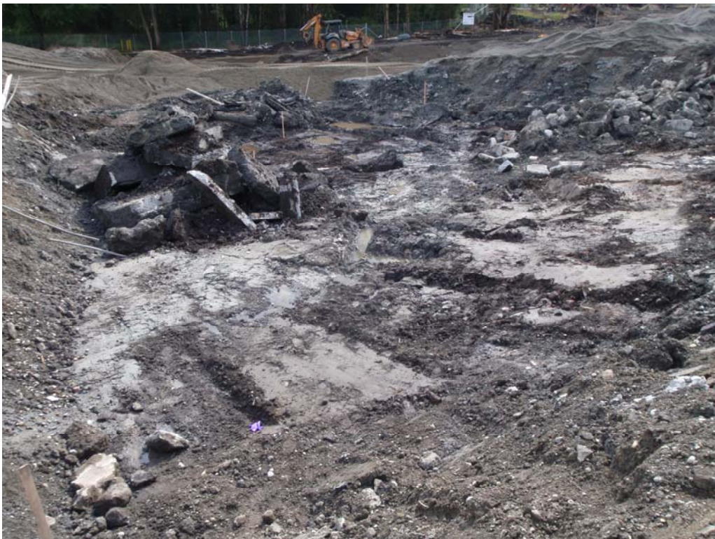
Photo 4 – Concrete and wood debris in north end of excavation (looking to south).
