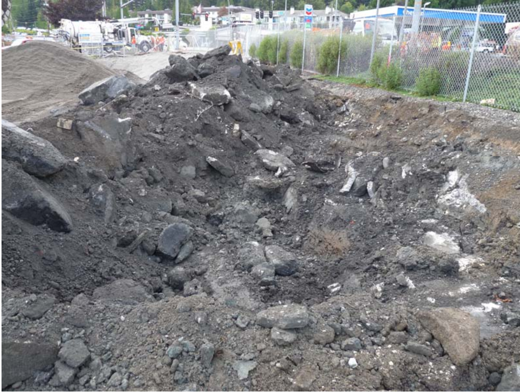
Photo 3 – Concrete and wood debris in north end of excavation (looking to northwest)
