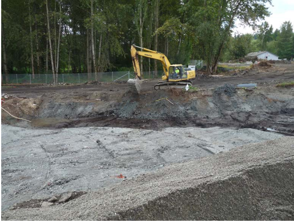
Photo 1 – Excavation limit looking southwest. Note peat layer on excavation floor. Select Borrow fill is being placed into excavation
