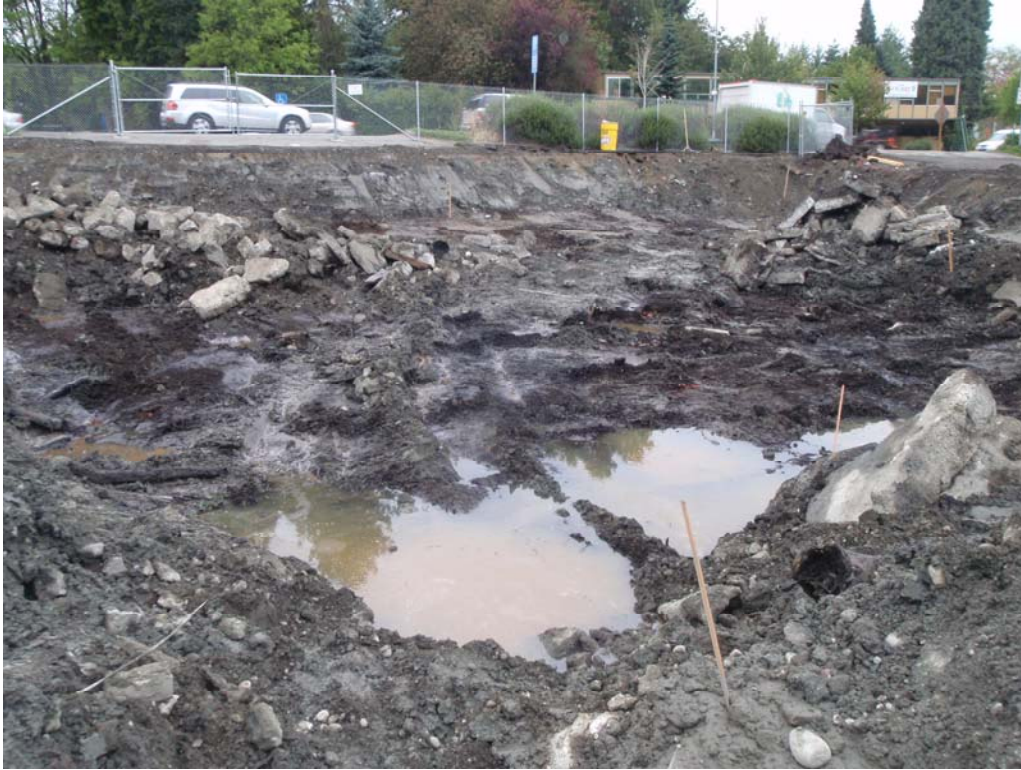
Photo 5 – Peat layer and water table exposed in northern excavation (looking north towards SR 522).
