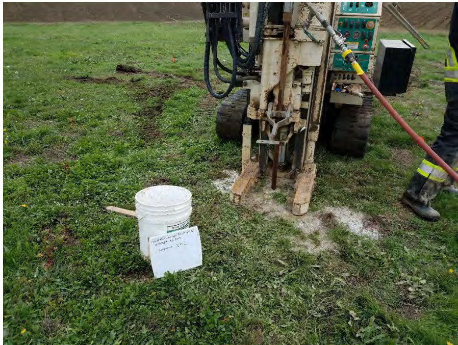
Photo 1 (top): Orientation - South Injection rig on secondary containment and product (RegenOX and ORC) on the lift gate. A water truck (filled at an onsite fire hydrant) was used to supply water to the injection rig.
