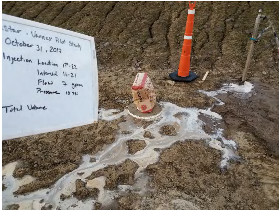
Photo 1 (top): Orientation – NA Injectant flowing from the borehole around the drilling rods at injection point IP-8.
