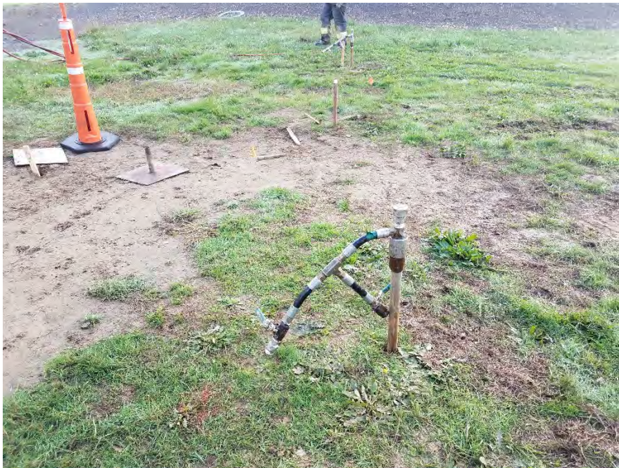
Photo 1 (top): Orientation - North Monitoring wells MW-5D (left) and MW-5 (right) are present in the foreground. The injection rig containing the mixing tanks and pumps is present in the background.
