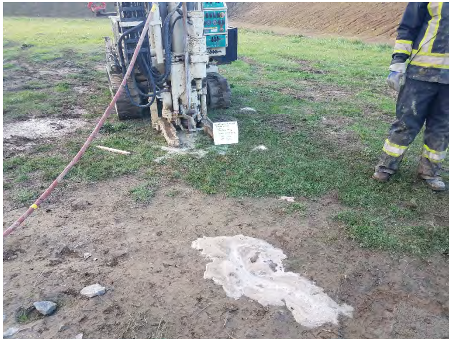
Photo 1 (top): Orientation - Northeast Pilot study injection area. The injection locations were hand augered to 8 feet bgs prior to advancing the injection rod. Cleared locations were covered with a steel plate cover or a large traffic cone.
