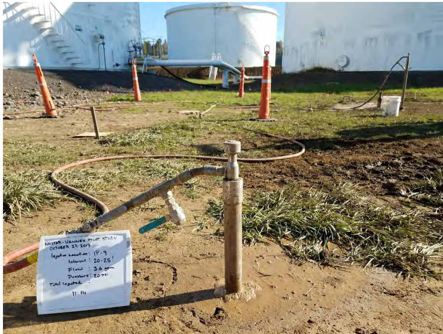
Photo 1 (top): Orientation – Northwest Injection at location IP-6 using a 5-foot injection point screened between 20 and 25 feet bgs.
