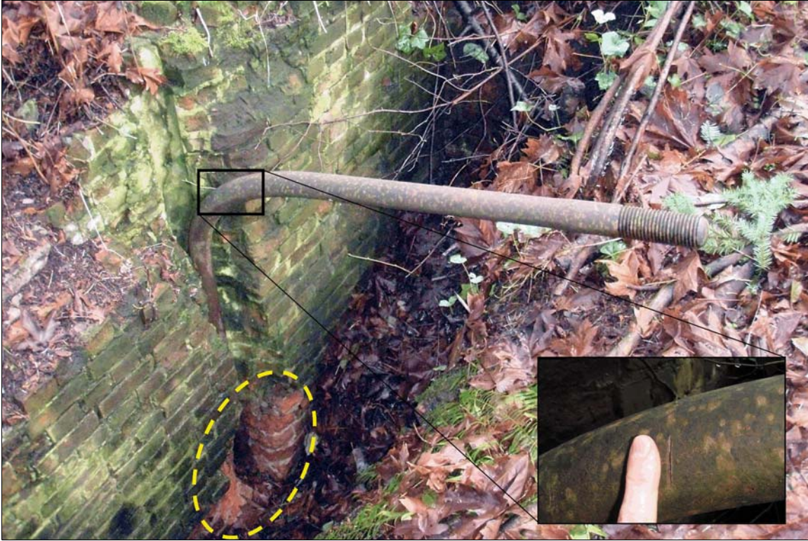
Figure 9. Overview of the Blower Engine base, view to the east. Note the recently broken bricks at the base of the masonry wall. Inset shows a partial saw cut mark near the center of the bolt.
