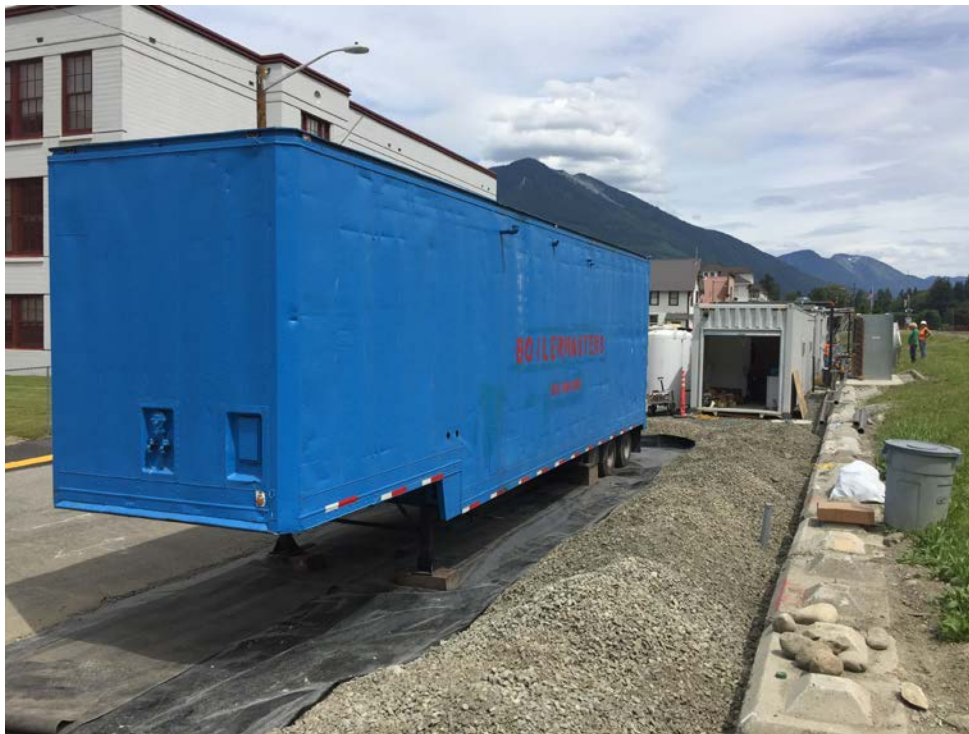
Photograph 12: Boiler staged at the HWF treatment compound, looking east.
