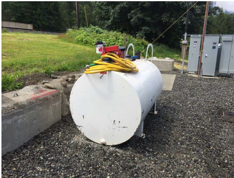
Photograph 14: Temporary fuel storage tank for the HWF system.
