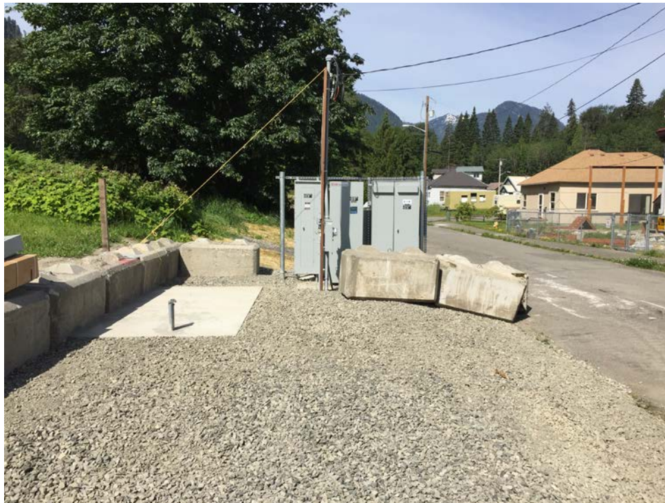
Photograph 8: Electrical panel and concrete pad for generator at the HWF treatment compound, looking west.
