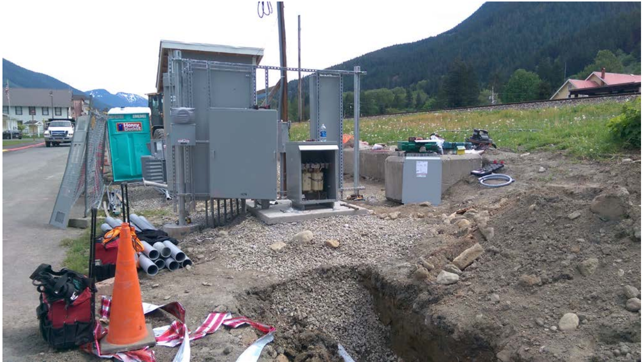
Photograph 13: HWF electrical panel and transformer, looking east.
