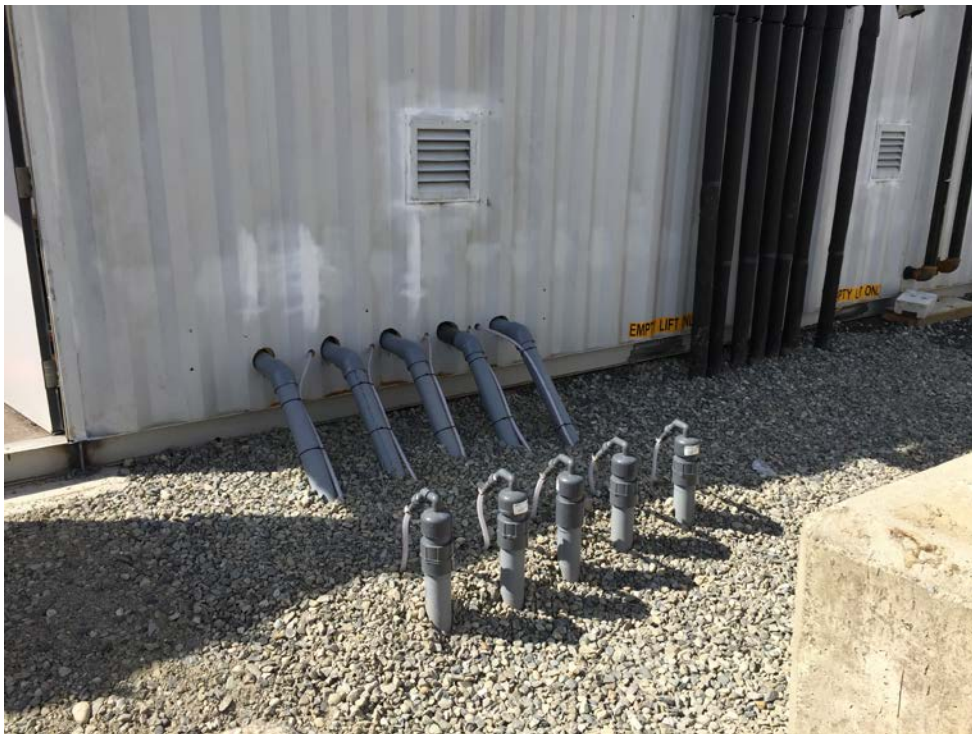
Photograph 10: Piping connecting the SVE condensation sumps to the SVE container.
