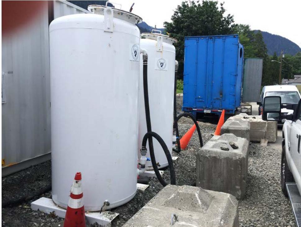
Photograph 15: Liquid-phase granular activated carbon treatment vessels at the HWF treatment compound.
