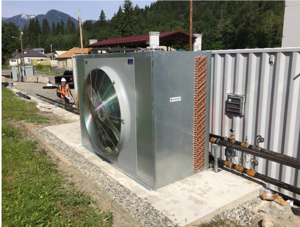
Photograph 11: Air-to-water heat exchanger installed adjacent to the HWF treatment compound.
