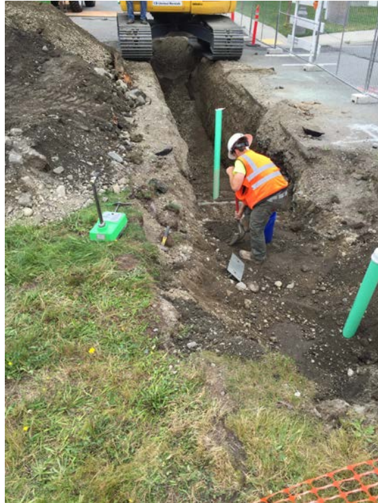
Photograph 23: New wye of teacheage side sewer adjacent to existing capped side sewer.
