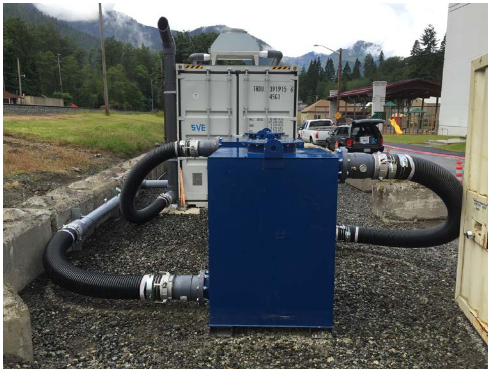
Photograph 16: Vapor-phase granular activated carbon treatment vessels at the HWF treatment compound.
