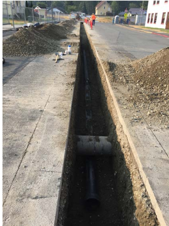
Photograph 3: Installed new water main below storm sewer line, looking south on Sixth Street.
