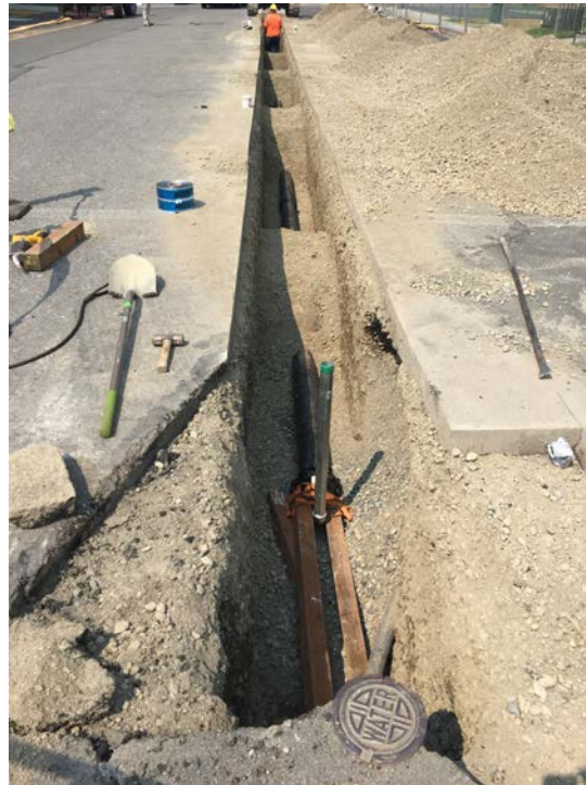
Photograph 2: Installation of new 6-inch ductile iron water main, looking north on Sixth Street.
