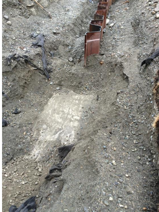
Photograph 13: End of sheet pile installation on northern side of school, facing east. Sheet piles are tied into ecology blocks.
