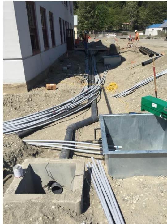
Photograph 19: Glacier Environmental installing hot water flushing piping on eastern side of school, facing north.
