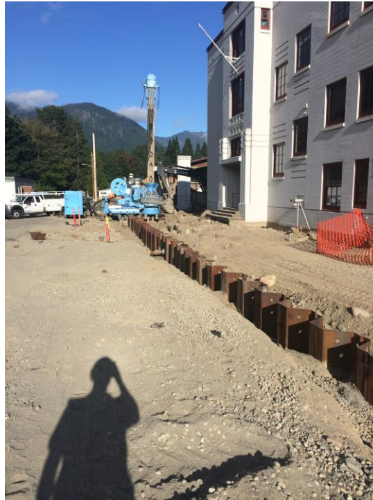
Photograph 11: Blue Iron installing sheet piles on southern side of school, facing west.
