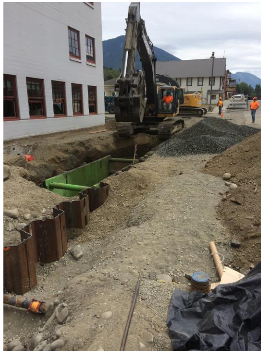
Photograph 16: Glacier Environmental excavating recovery trench on southern side of school, facing east.
