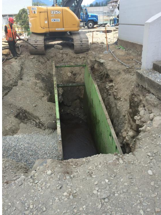
Photograph 17: Northern side of school showing trench box used for recovery well trenching, facing east.
