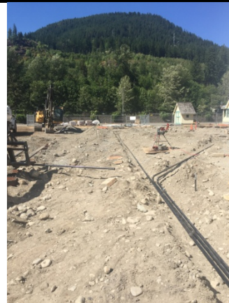
Description: Glacier installs HWF injection piping along west side of the school.
