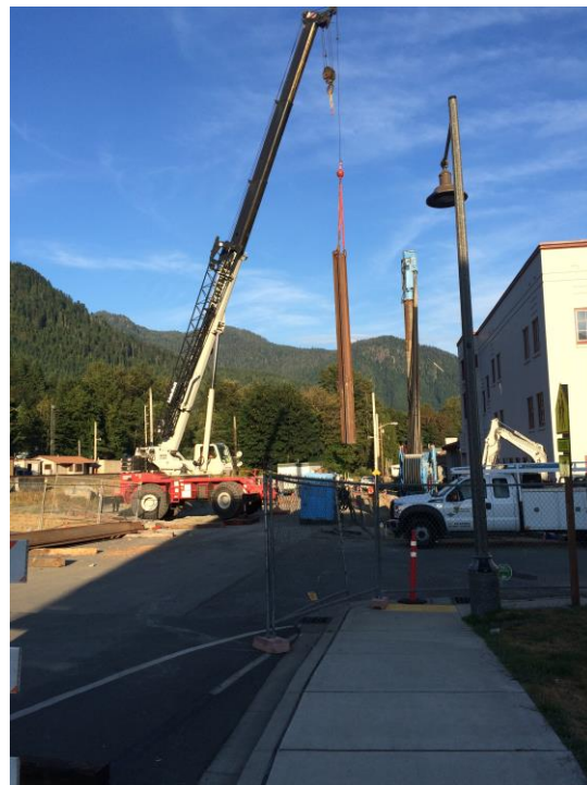
Photograph 6: Blue Iron installing sheet piles on southern side of school, facing west.
