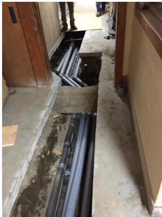
Photograph 8: School interior showing interior hot water flushing system piping, facing east.
