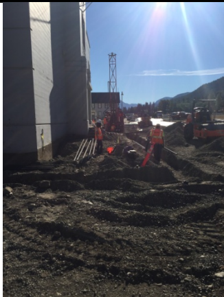
Description: Glacier installs HWF injection piping along south side of the school.
