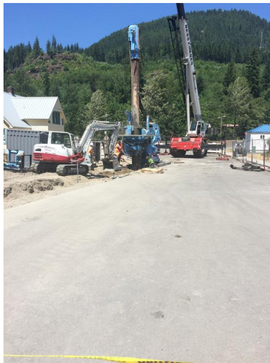
Photograph 4: Blue Iron installing sheet piles on eastern side of school, facing north.
