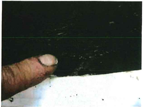
Photograph 8. Corrosion Hole in UST #2
