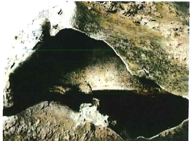
Photograph 14. Corrosion Hole in UST #3
