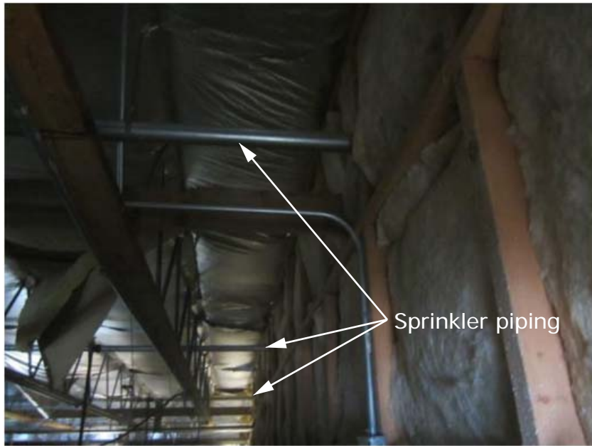
Photo 1. Showing sprinkler piping inside the former Hallmark Suite penetrating the wall into Amy's on the right.
