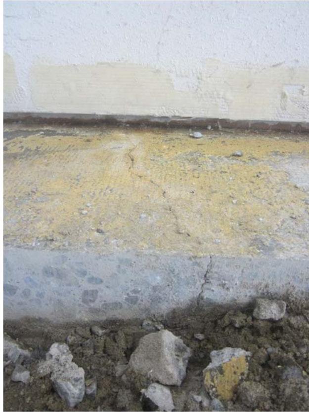
Photo 1. Fully penetrating crack through the slab in the former Hallmark Suite floor. Crack extends below the demising wall between this suite and Amy's Dry Cleaners.
