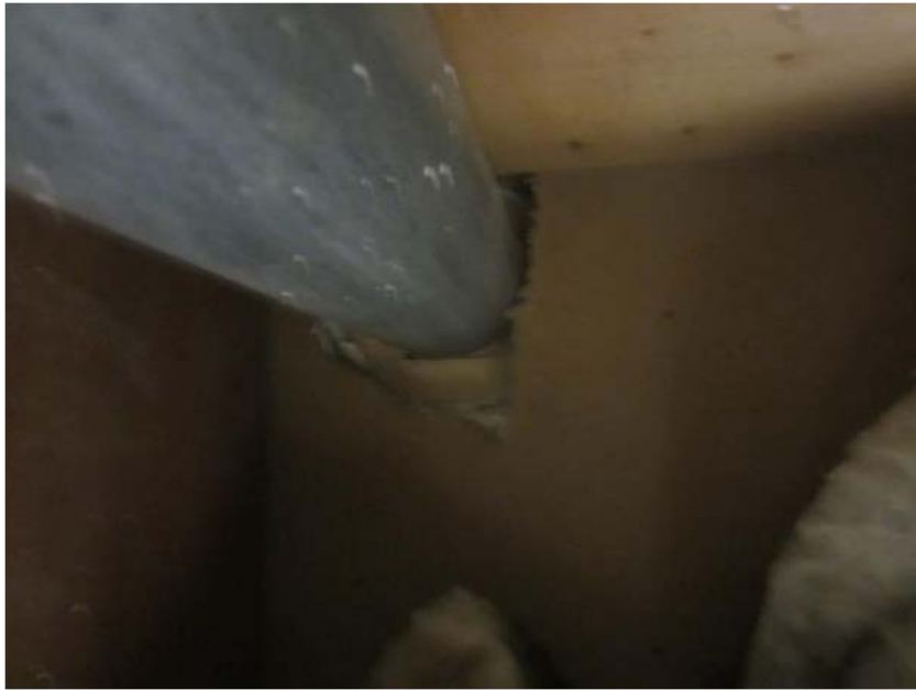
Photo 2. Pipe in southwest corner of Hallmark suite above drop ceiling penetrating the drywall separating Amy's and Hallmark.
