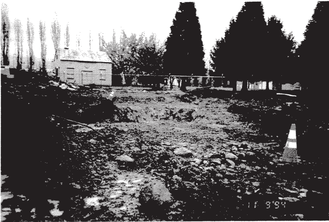
Photograph #6: Shallow excavation. Cones mark MW-5 (foreground) and MW-1 (background). Photograph taken looking southeast.
