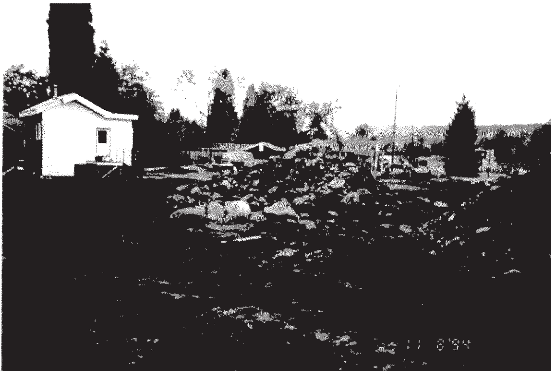
Photograph #7: Stockpile of screened rock (in center) after one day of screening. Compactor used for compacting backfill in background. Photograph taken looking west.
