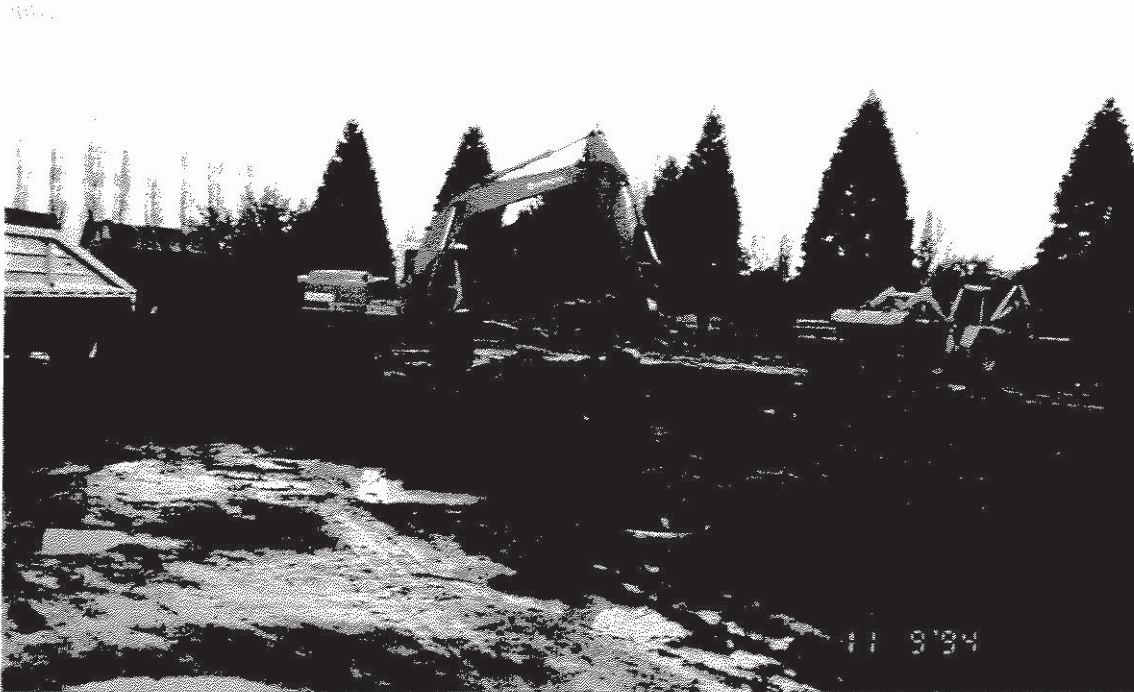
Photograph #8: Placing screened rocks into former AST's excavation. Imported sand to be mixed in with rocks is to left. Hoepack at right. Photograph taken looking east.
