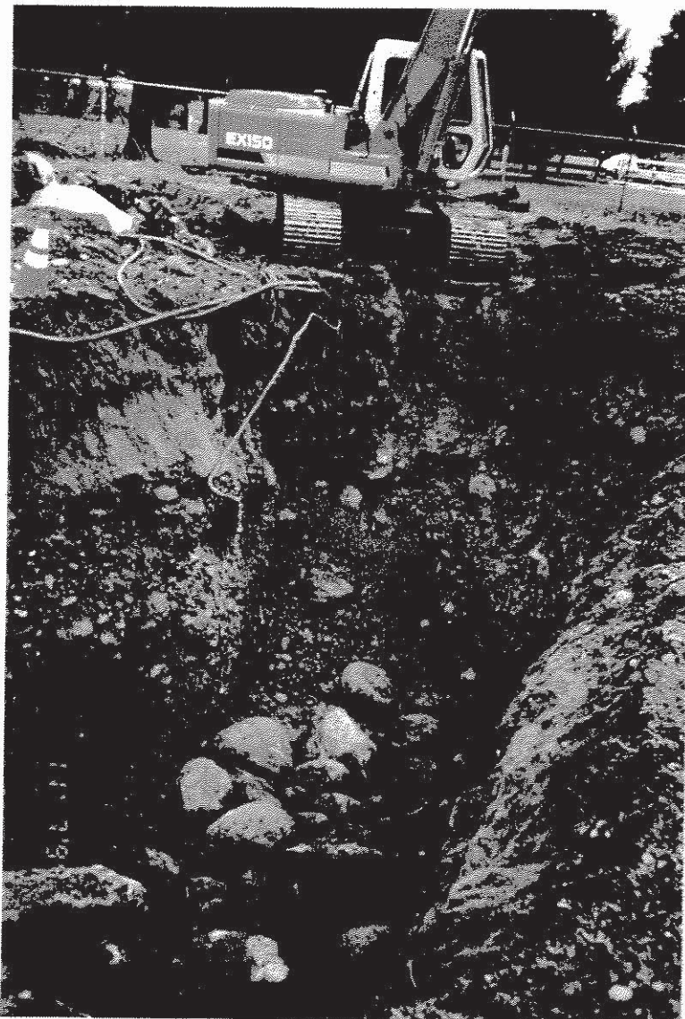
Photograph #3: Former ASTs excavation. Note boulders at bottom. Photograph taken looking south (MW-1 marked by cone).
