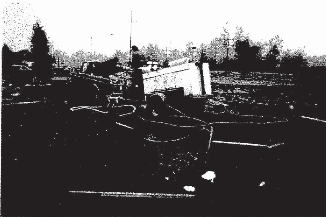
Photograph #11: Abandoning MW-1 by grouting. Note crushed rock for grade. Photograph taken looking northwest.
