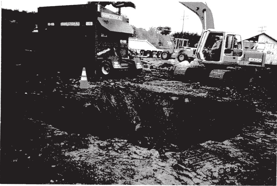
Photograph #1: Excavation of former loading rack area and screening. Loading in background. Photograph taken looking east.
