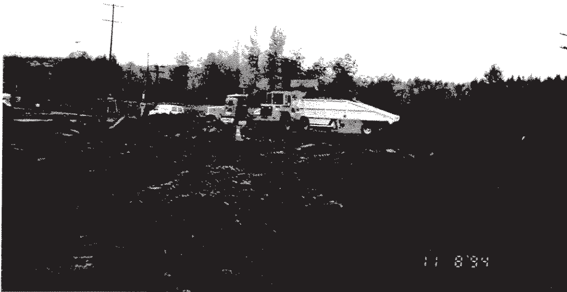
Photograph #4: Loading screened soil into belly dump from stockpile at right. Photograph taken looking northwest.
