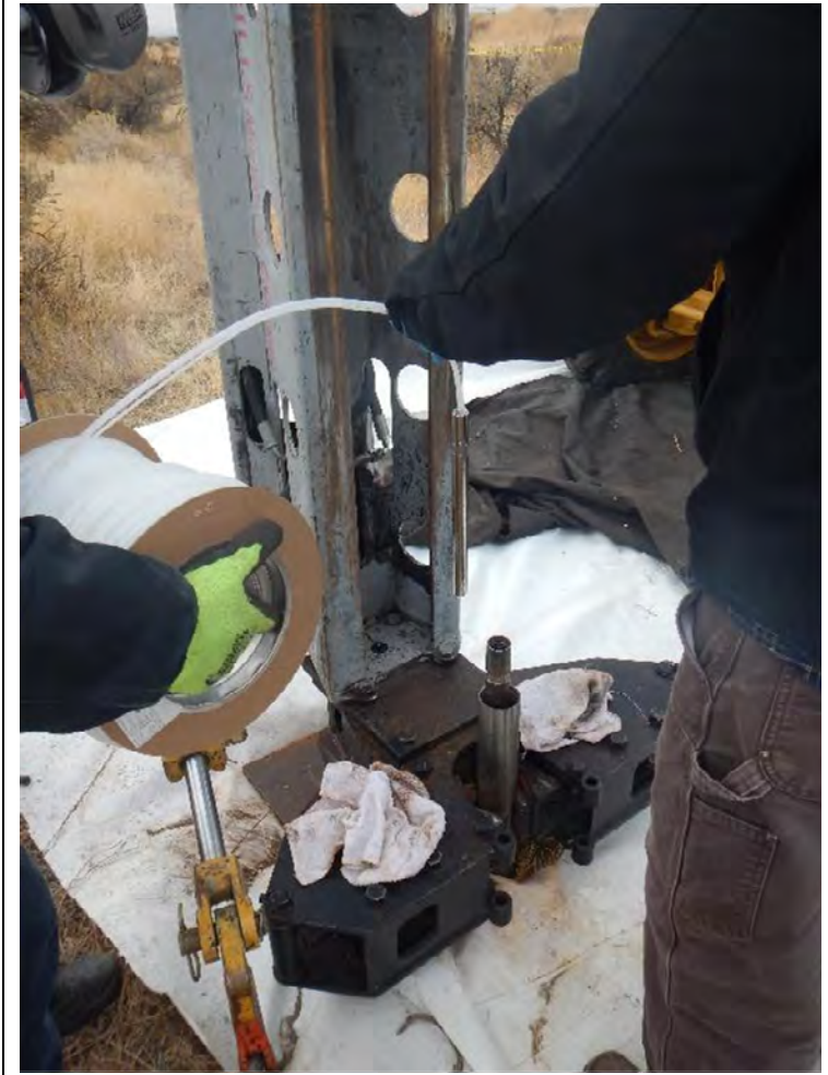
Groundwater sampling pump and tubing at PP-2
