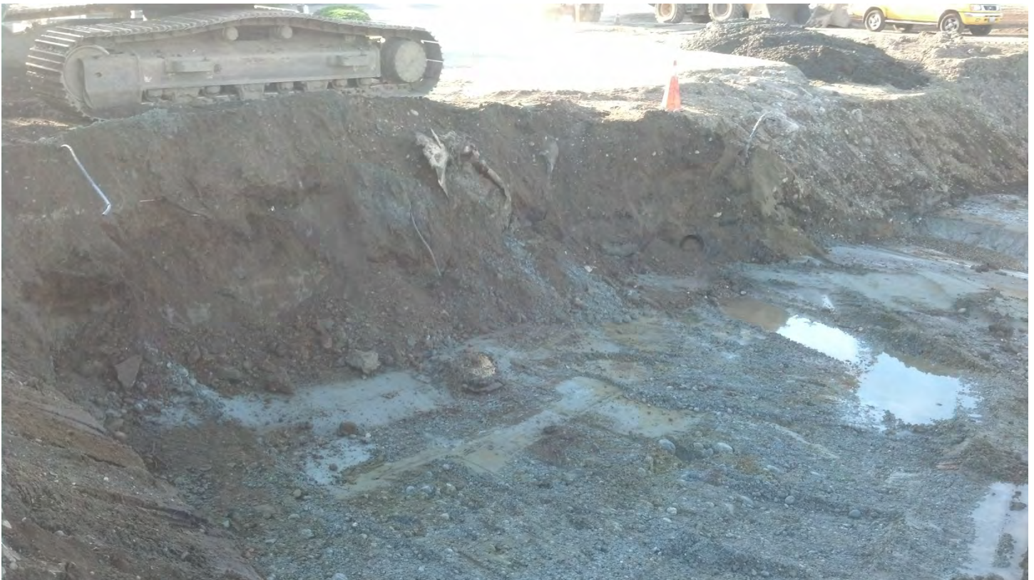
Photo 21 – UST exposed during remedial soil excavation. Tank end is visible in sidewall below excavator track.
