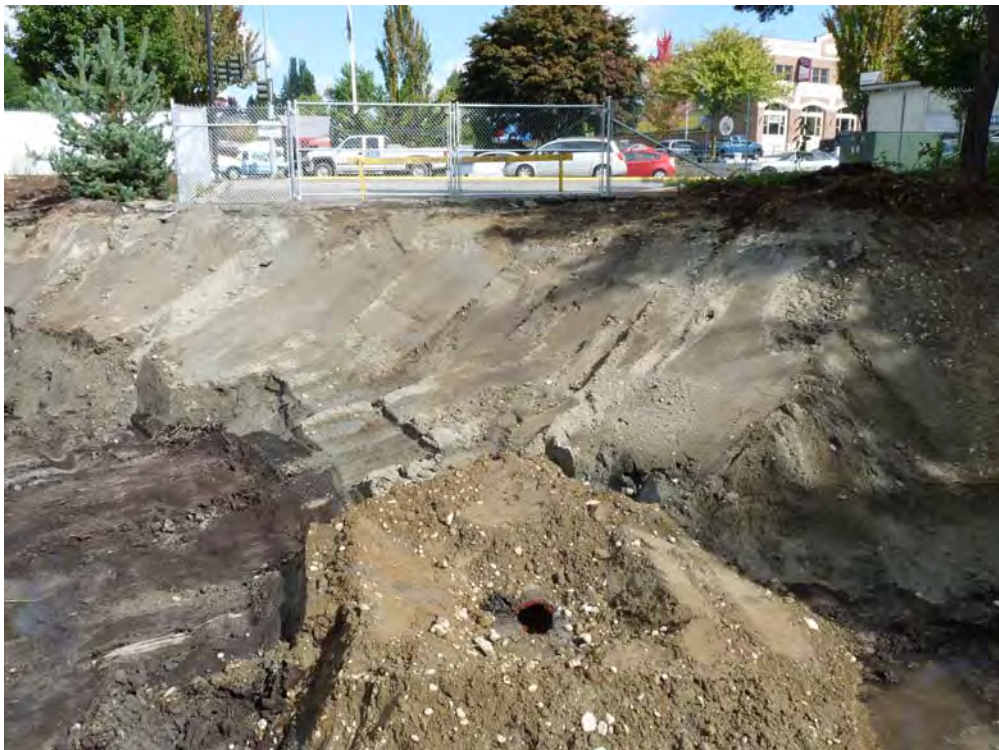
Photo 2 – Uncovered abandoned storm drain pipe in northeast corner of excavation
