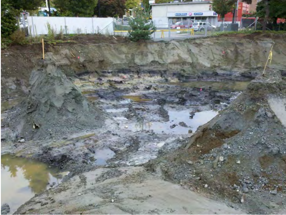
Photo 9 – Monitoring wells MW-3 (left) and MW-4 (right) prior to decommissioning by excavation (looking to northeast)
