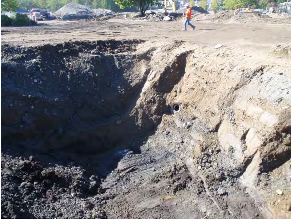
Photo 5 – Exposed abandoned storm drain side connection to Horse Creek Culvert in western extent of excavation (looking southwest)
