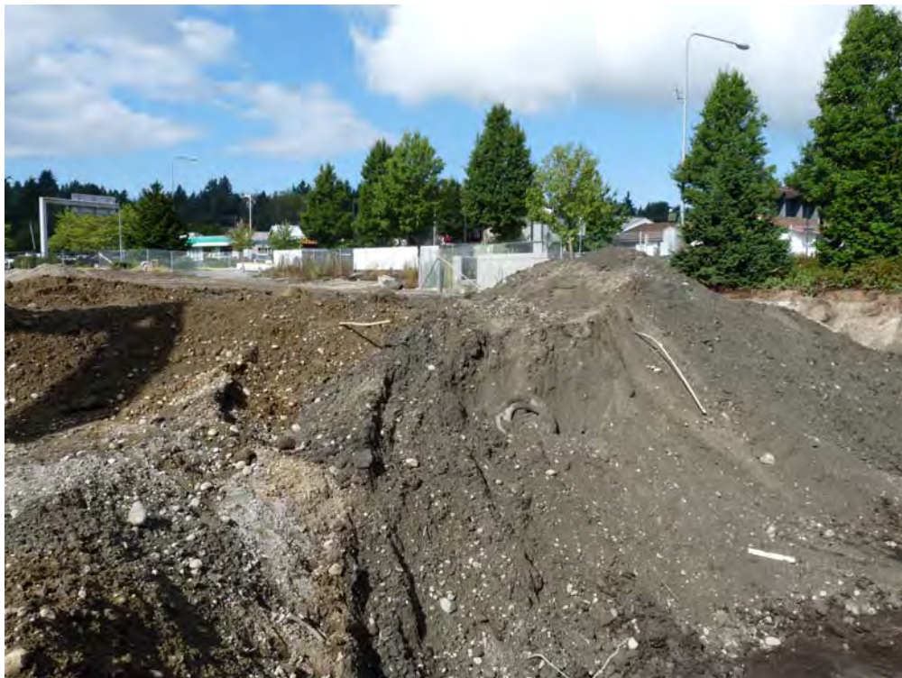
Photo 4 – Buried debris in west end of excavation below Rotunda Park (looking to northwest)
