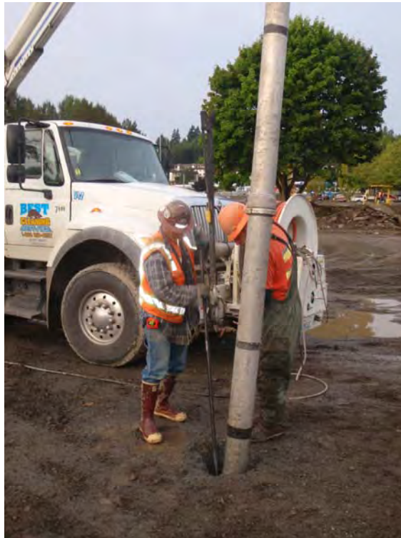
Photo 6 – Using a vactor truck to excavate an exploration borehole adjacent to Horse Creek culvert
