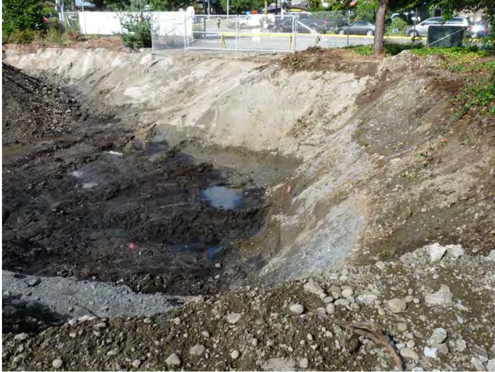
Photo 1 – Excavation limit looking north to SR 522. Note peat layer on excavation floor. Extent of excavation was limited to maintain the structural integrity of SR 522 and related sidewalk and utilities
