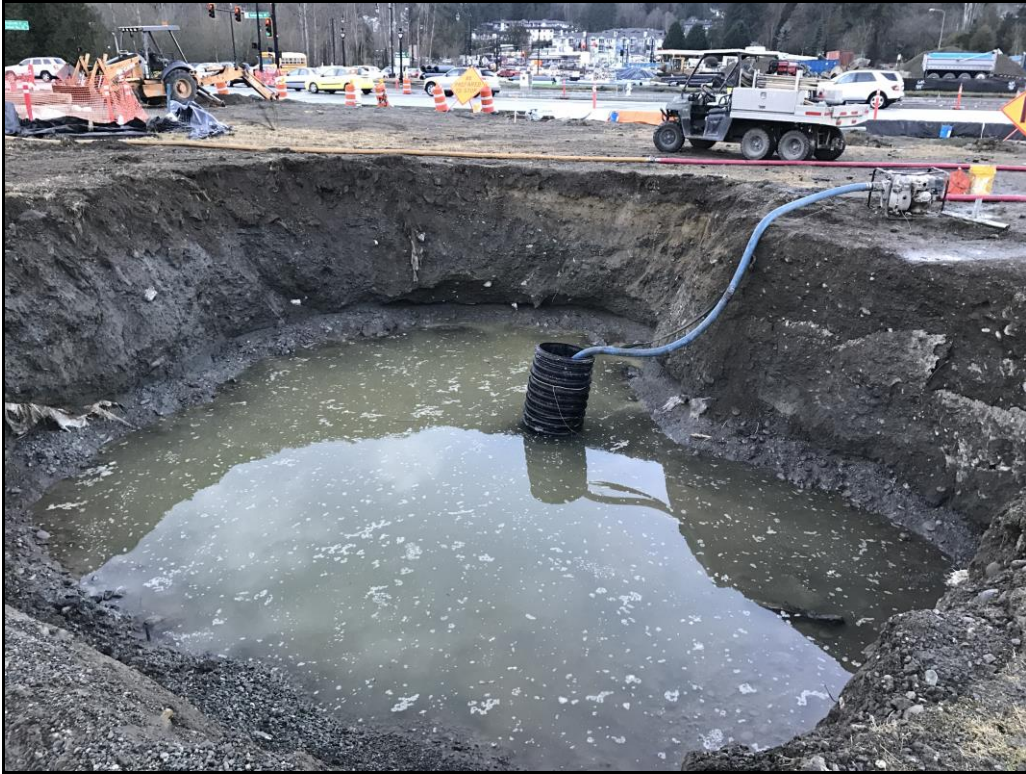
Photograph 1: View facing west toward the final boundaries of the 2017 Bothell Landing remedial excavation. Photograph taken prior to pumping water that had accumulated in the excavation.
