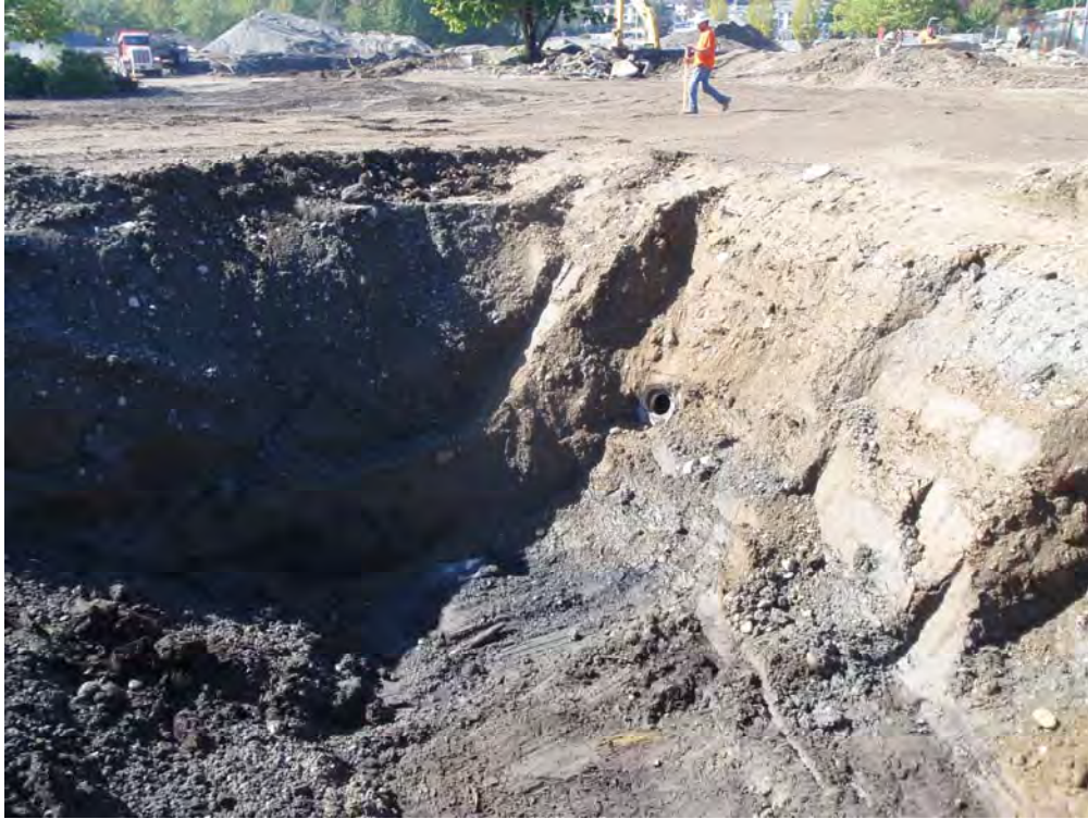
Photo 5 – Exposed abandoned storm drain side connection to Horse Creek Culvert in western extent of excavation (looking southwest)
