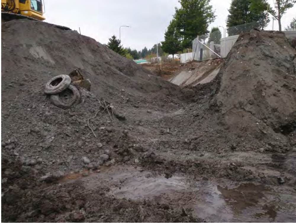
Photo 3 – Buried debris in west end of excavation below Rotunda Park (looking to northwest)
