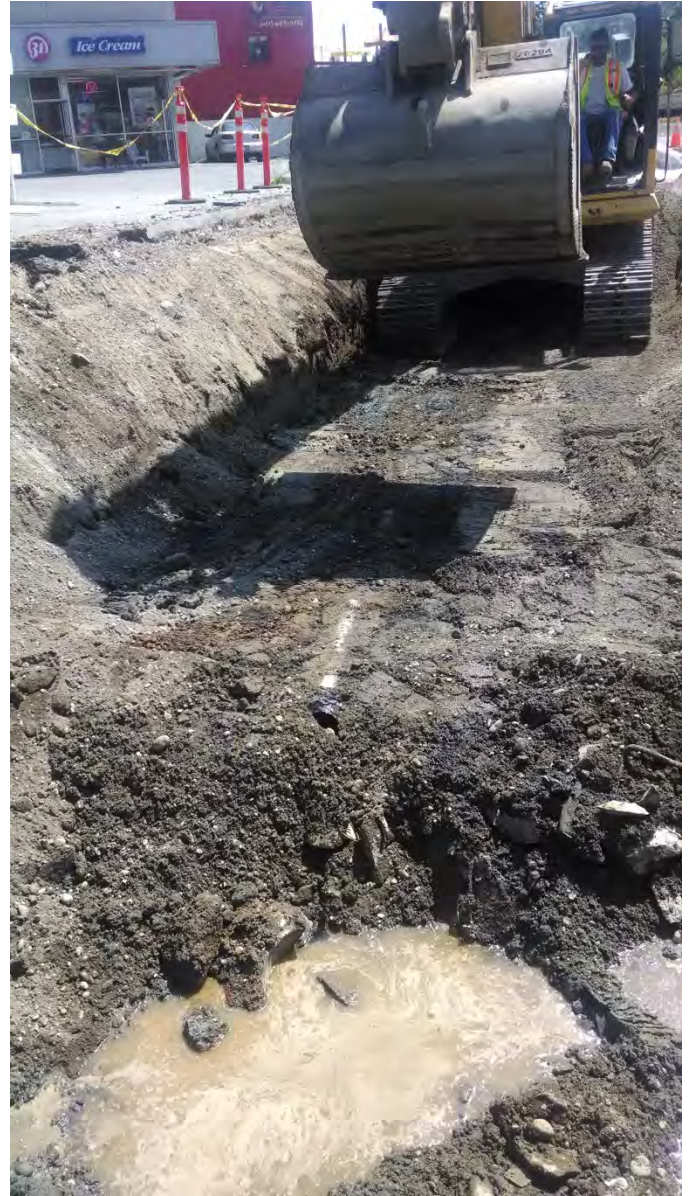
Photo 27 – Excavation of soils along project limit, north edge of former SR-522, view east
