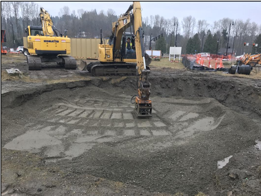
Photograph 2: View facing south toward the 2017 Bothell Landing remedial excavation during backfilling activities. Brown Baker tank utilized for storing water pumped from the excavation visible in the background.
