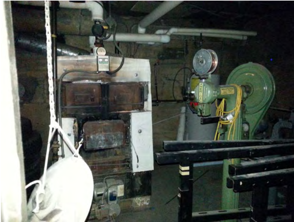
13.) View of the furnace in the basement of the 104 12 th Avenue building.
