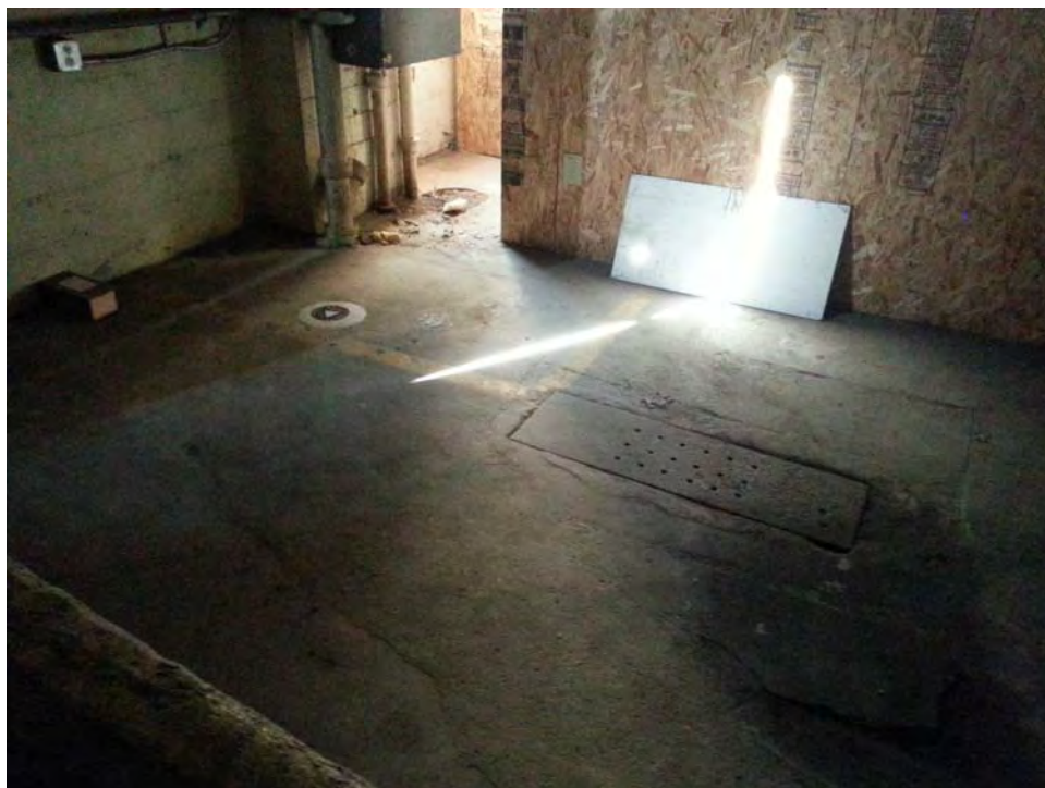
12.) View of the oil/water separator in the southwestern corner of the 104 12 th Avenue building. Adjacent monitoring well installed in 2016 site investigation.
