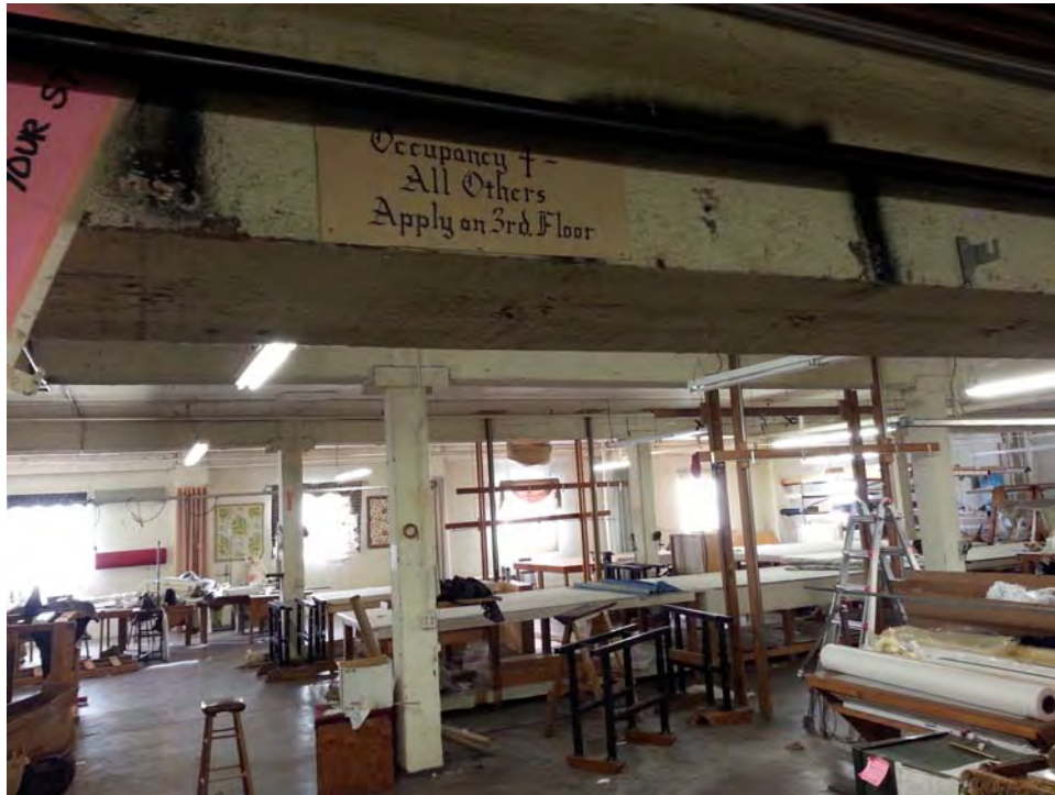
11.) View of the basement storage and work areas of the 104 12 th Avenue building.
