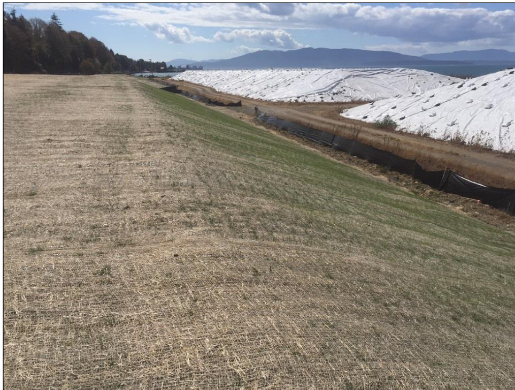
4. Top of pile showing western slope, silt fence visible, grass visible. Loose soil along upstream side of silt fence needs to be graded out and stabilized with grass or some other means.
