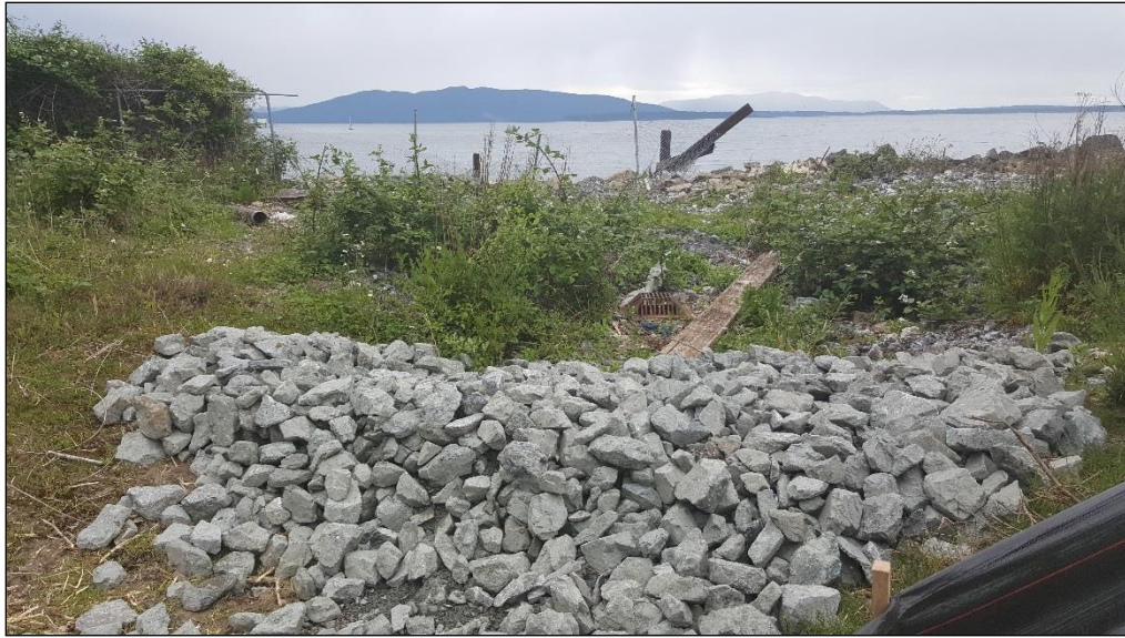
8. Quarry spall check dam installed instead of silt fence.
