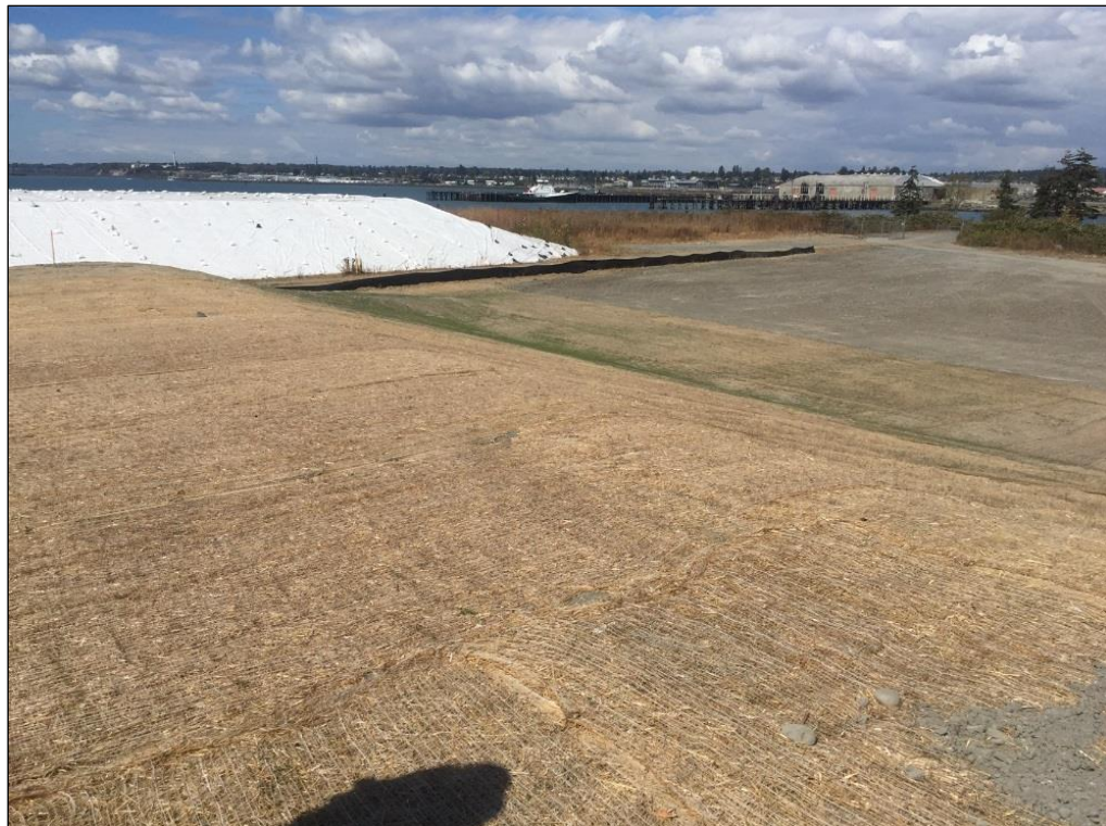
6. Top of pile looking northwest, silt fence visible, some grass visible on northern slope. Per survey, fill needs to be added to areas north of pile to facilitate drainage.
