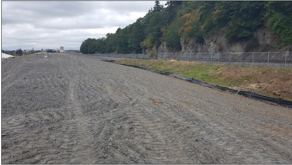
25. Looking north toward northern stockpile from middle of south stockpile. Erosion control matting being placed.
