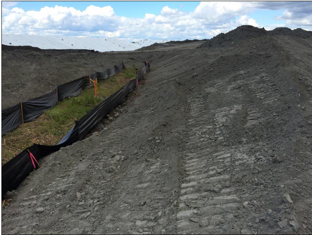
22. Looking west between the two stockpiles. Note silt fence has been repaired.
