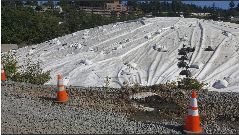
12. Area where cap material was damaged by truck traffic.
