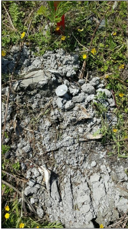
1. Destroyed settlement survey monument SSM-5.
