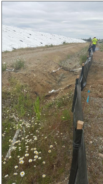
7. Ditches have been connected for stormwater flow. A culvert was installed here after this photo was taken.
