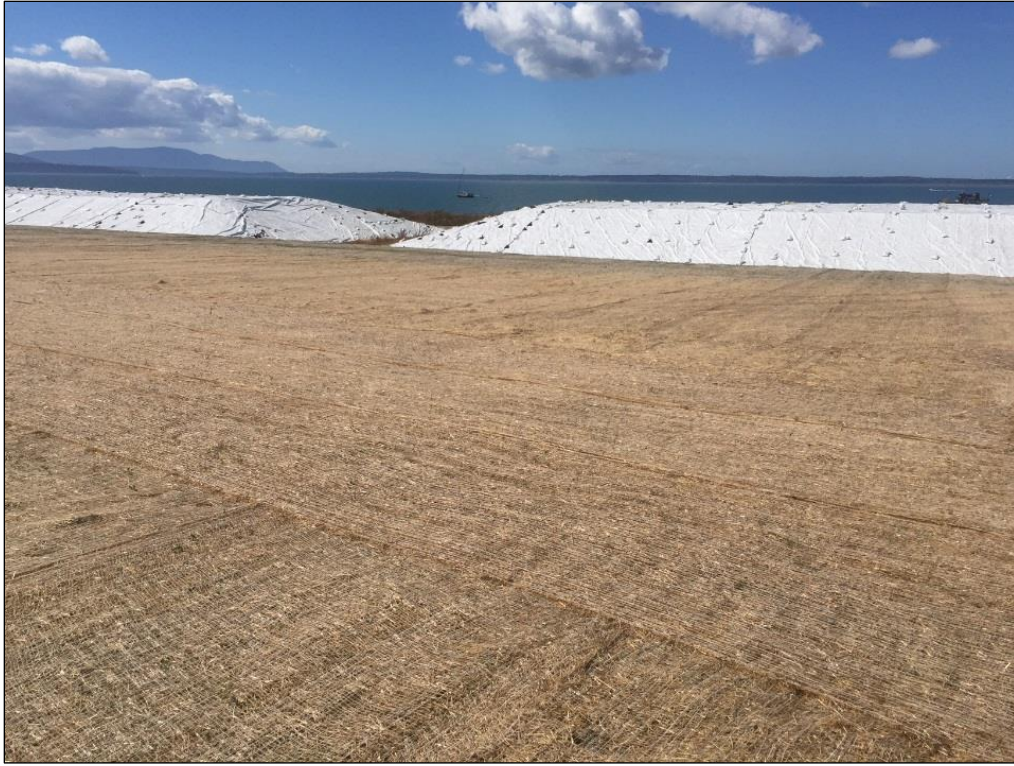
1. Top of pile, looking west toward IPAs. Jute matting and grass coverage is typical of 90% of the pile.
