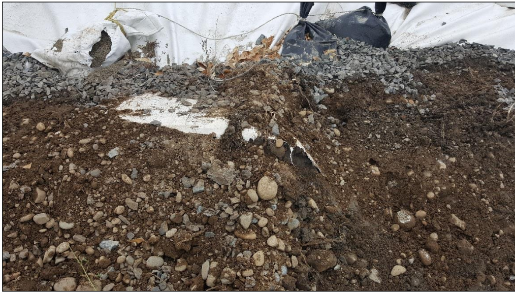
26. Repairs made to damaged stockpile cover.
