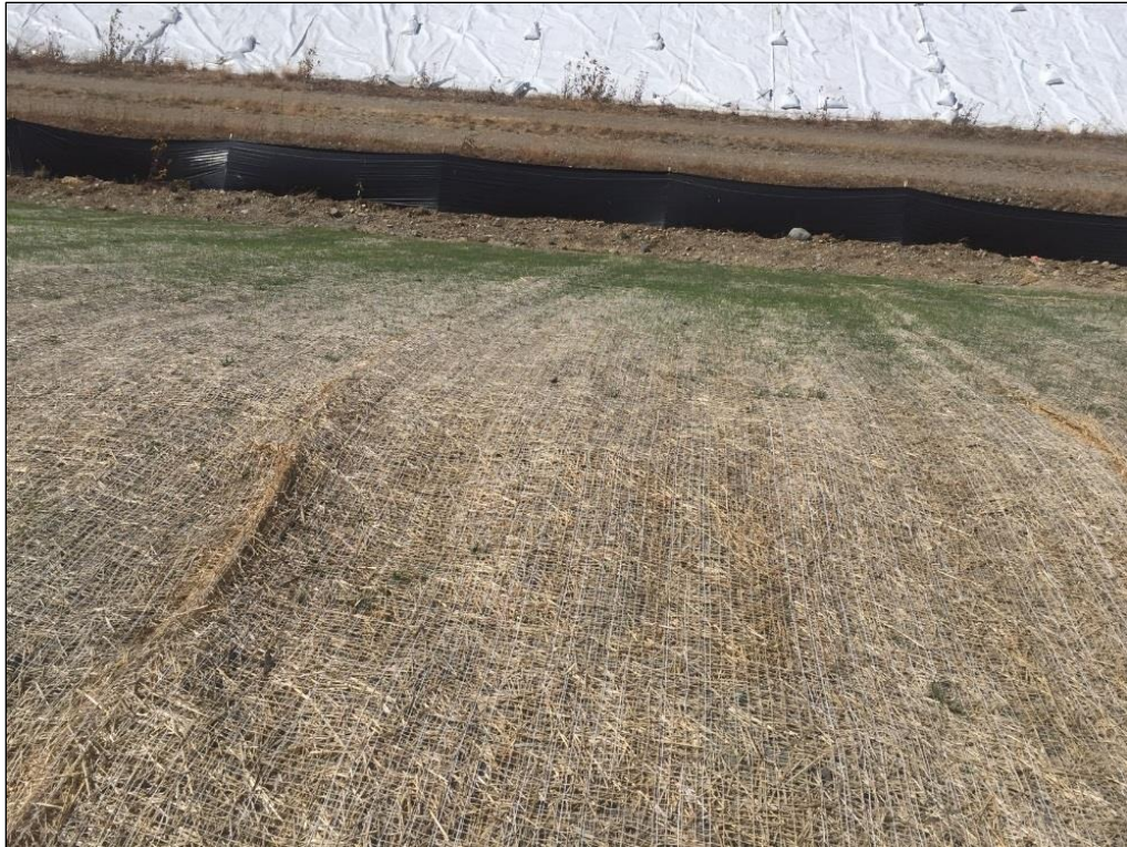
5. Top of pile looking west, down the western slope, silt fence visible, grass visible.
