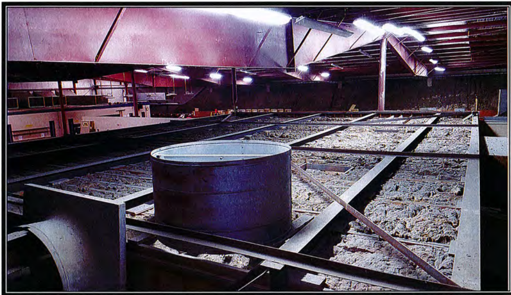
Photo #4 – Settled dust on fiberglass insulation
