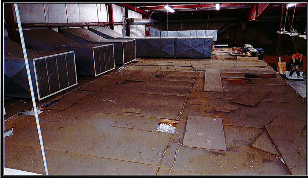
Photo #3 – Settled dust above training room
