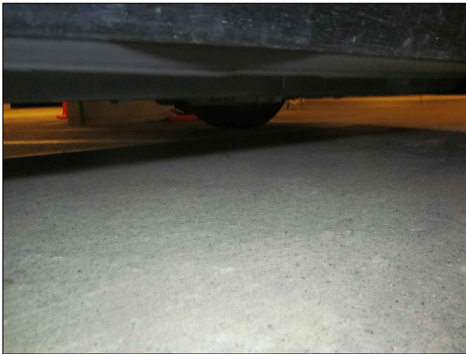
Photograph 4: View looking northwest representing the condition of the garage floor slab at the eastern portion of Area 2.
