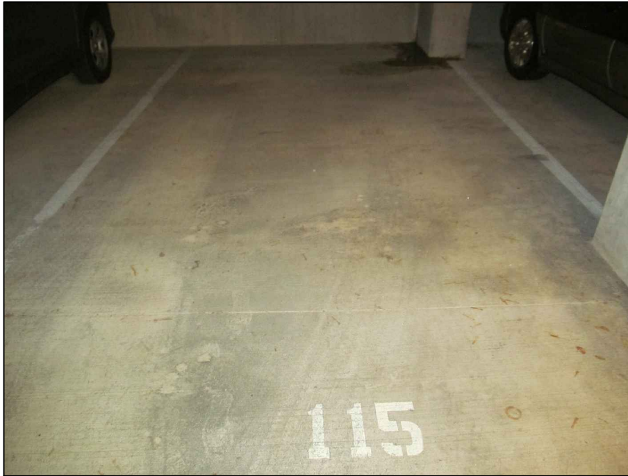
Photograph 1: View looking west representing the condition of the garage floor slab at the northern portion of Area 1,
