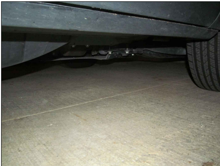
Photograph 2: View looking southwest representing the condition of the garage floor slab at the southern portion of Area 1.
