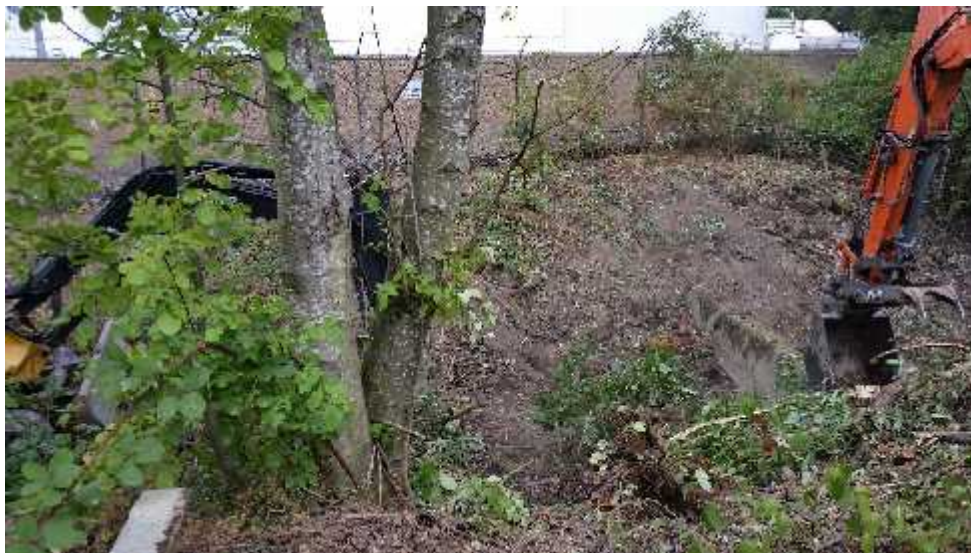
Photo 2 - Alternate view of active vegetation clearing activities within the excavation area, from the Southwest 27 th Street right-of-way, facing north.
