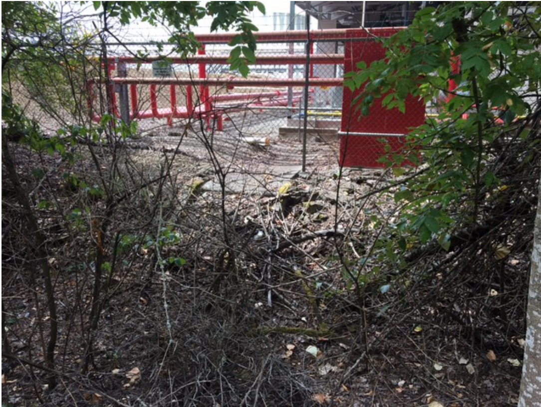
Photo 1 - Edge of detention pond showing abandoned inlet to pond.
