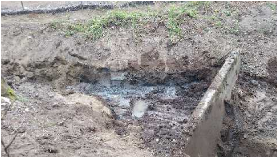
Photo 3 - View of the completed western portion of the remedial excavation area, from the Southwest 27 th Street right-of-way, facing north-northwest.
