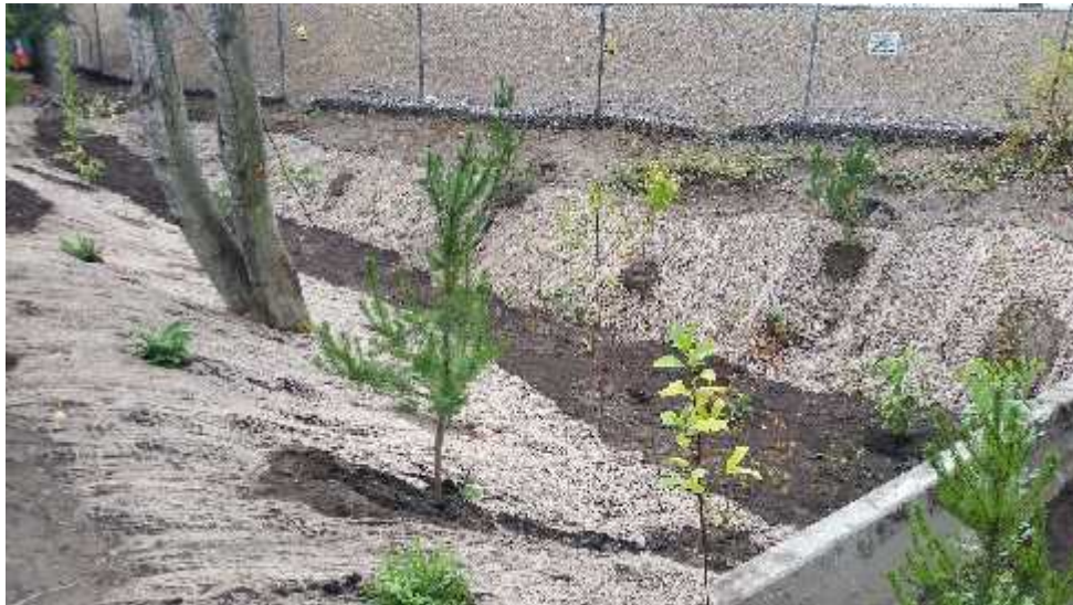
Photo 6 - View of the western portion of the remedial excavation post revegetation, from the Southwest 27 th Street right-of-way, facing northwest.
