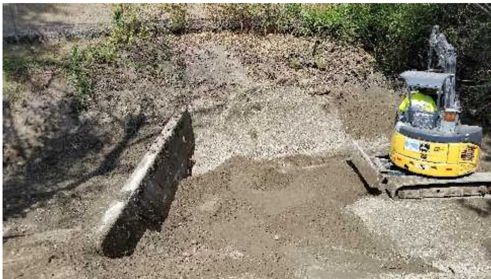
Photo 4 - View of backfilling activities within the eastern portion of the remedial excavation area, from the Southwest 27 th Street right-of-way, facing northwest.
