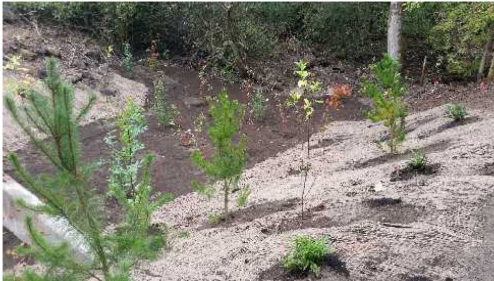
Photo 7 - View of the eastern portion of the remedial excavation post revegetation, from the Southwest 27 th Street right-of-way, facing northeast.
