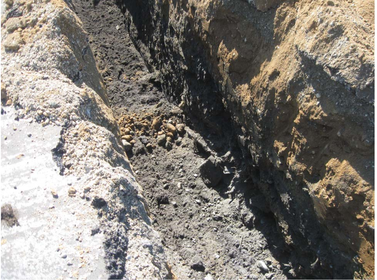
Exploratory trench opened to about 7 feet in depth showing some of the random debris being found in the fill materials.
