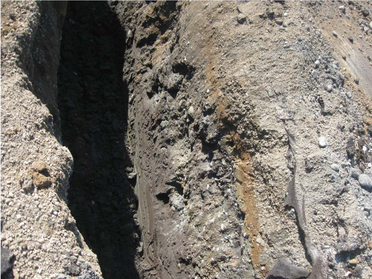
Exploratory trench at station 12+30 with grey sandy silt original ground exposed on trench bottom.
