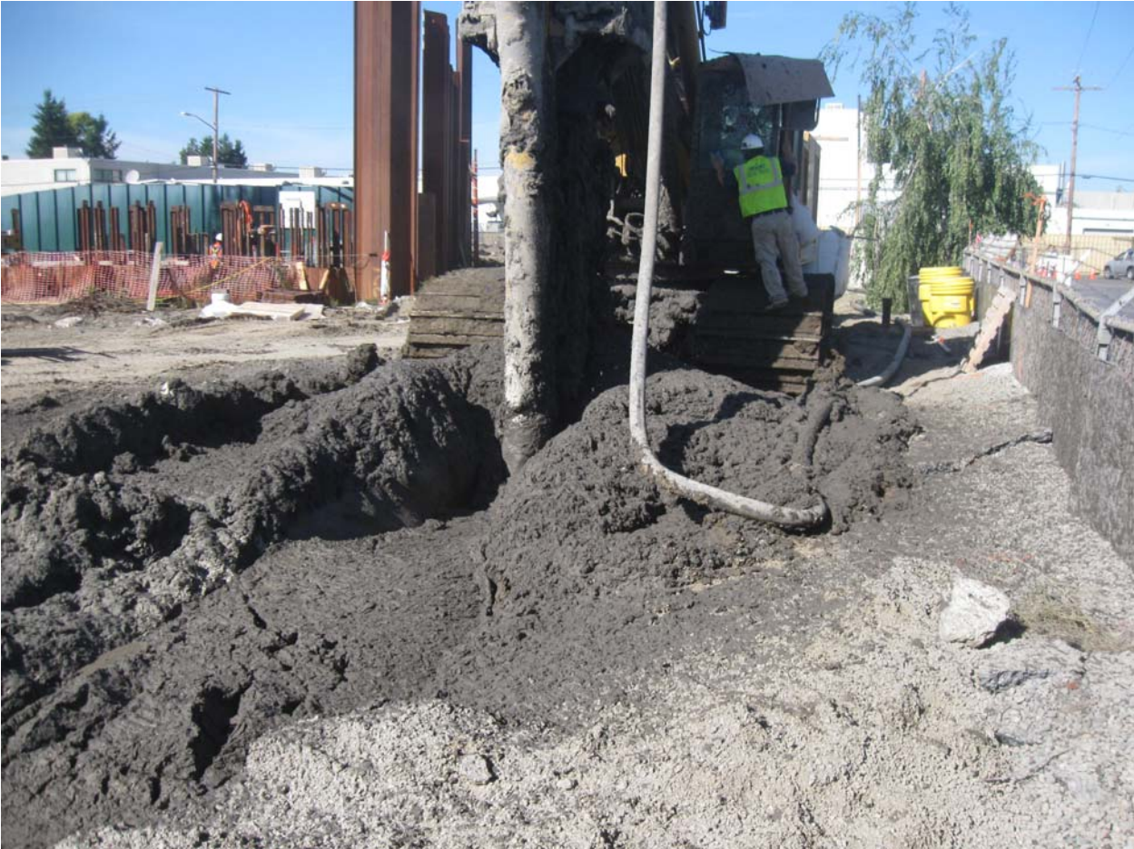
Trenching without trench box.
