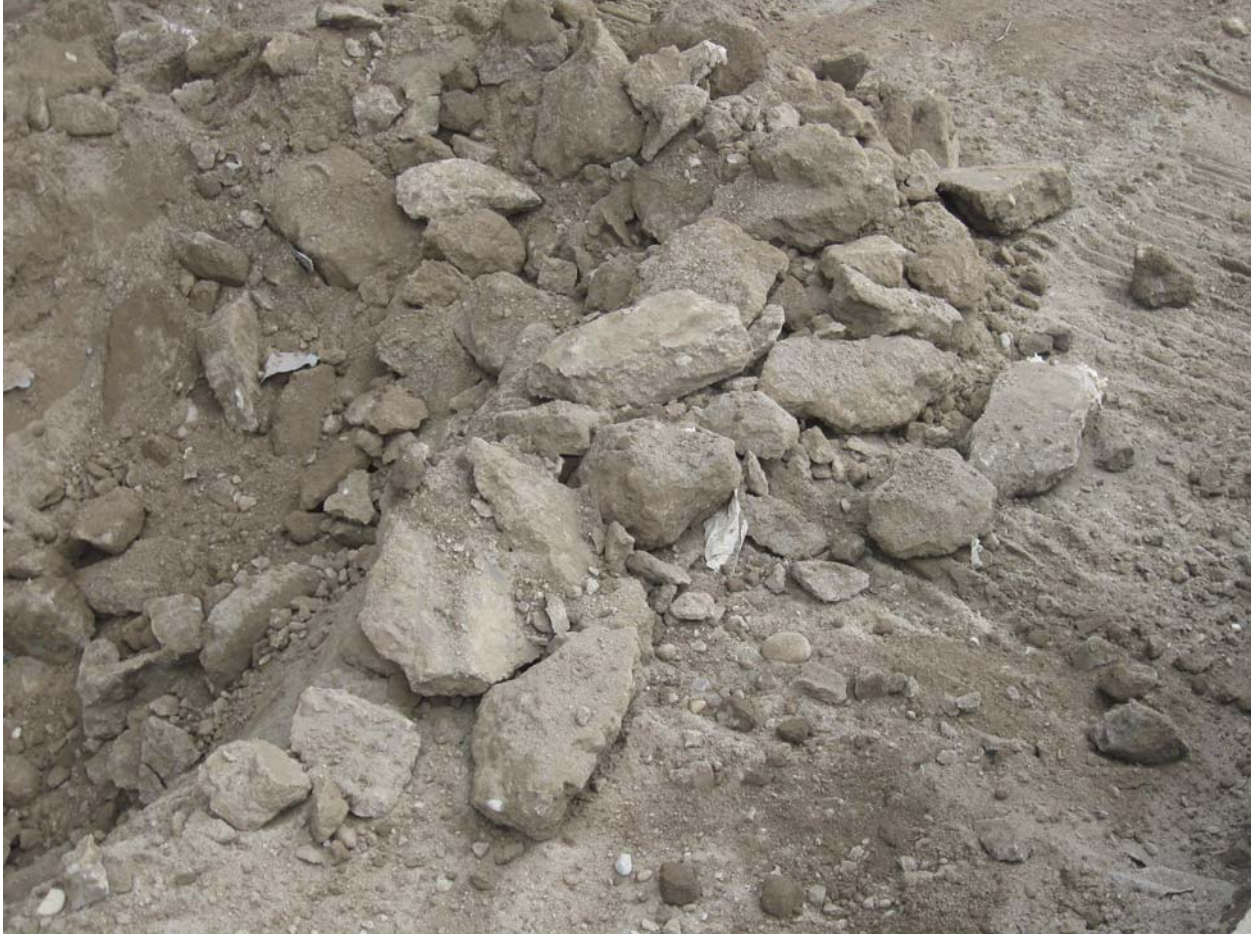
Cement stabilized sludge found under PVC cover from station 0+00 TO 1+50.
