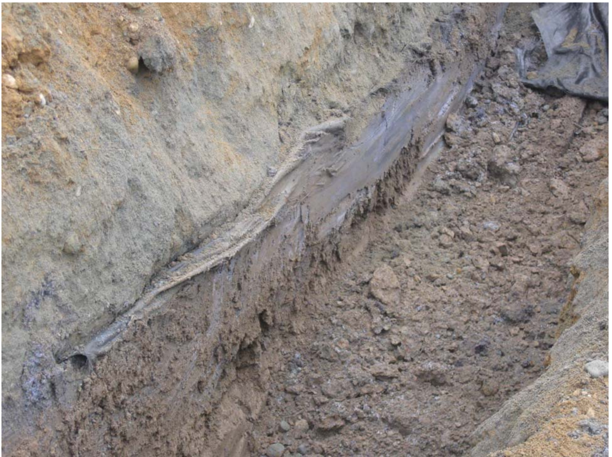
Exploratory trench at approximately 14+50 with sludge under geotextile and original ground exposed on the bottom of the trench.
