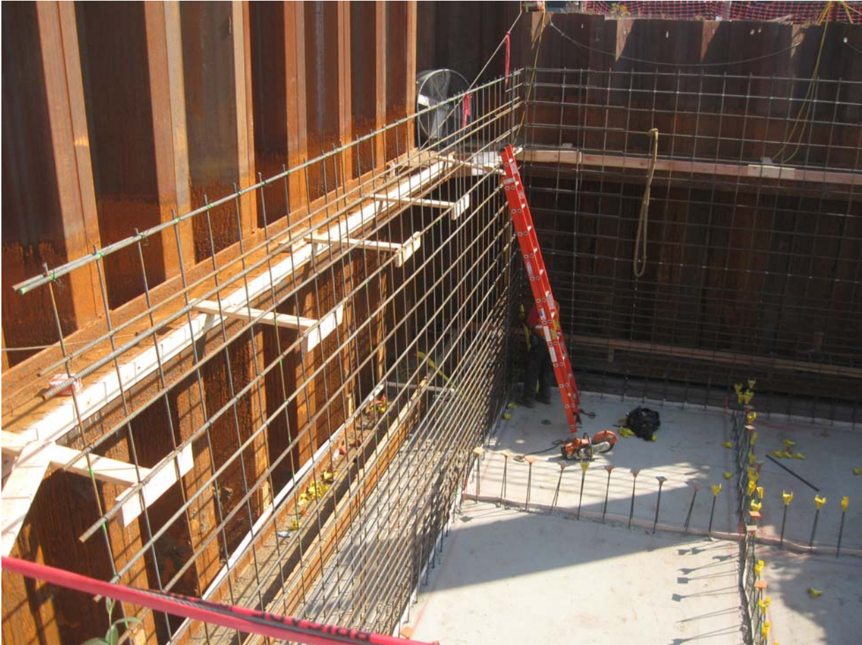
2 x 6 framing used to position east wall rebar in position relative to outside form.
