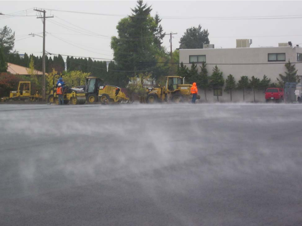
Steam on pavement as light rain begins.
