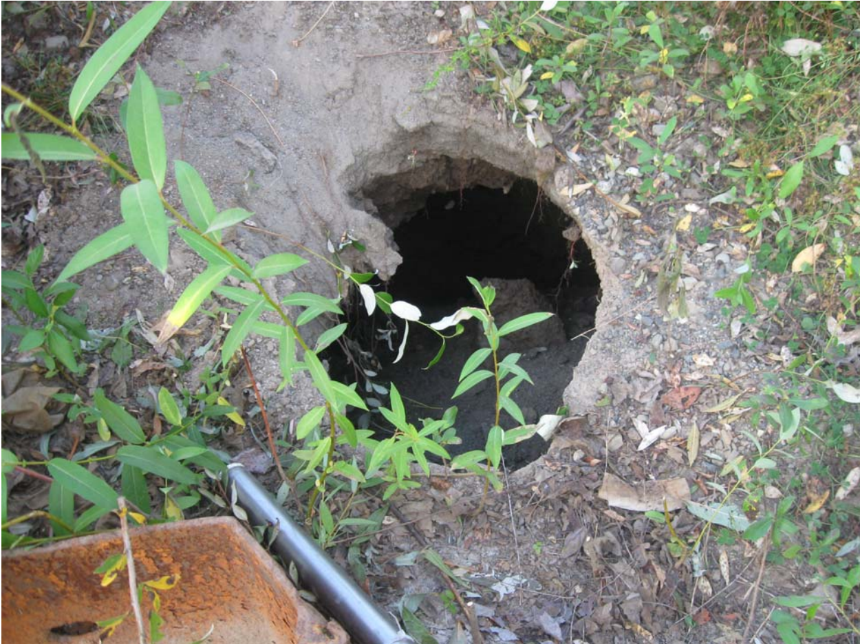
Sink hole at northwest corner of excavation outside of sheet piles.
