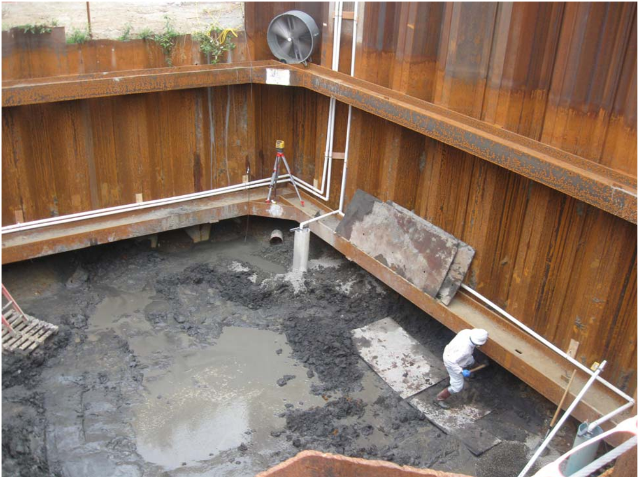
Hard pipe discharge from wells to Baker tanks.
