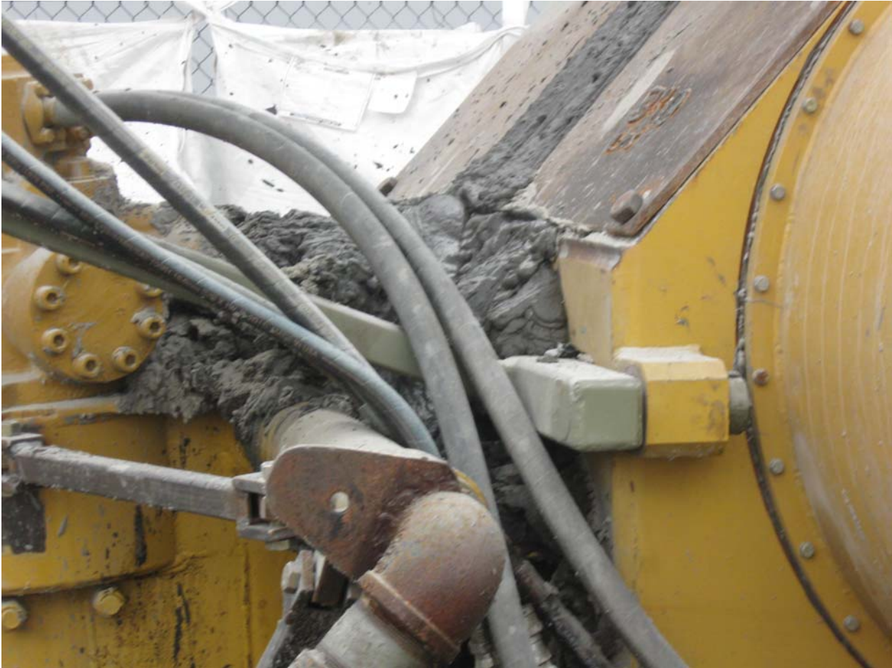
Slurry spilling from top of rotating chain.
