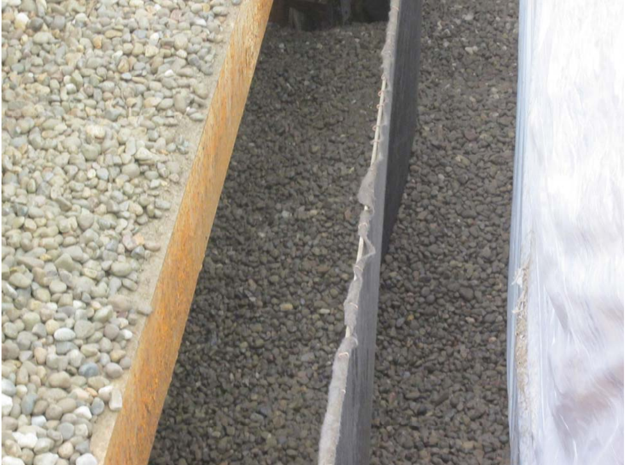
Drain rock placed on both sides of the geotextile west side of vault.
