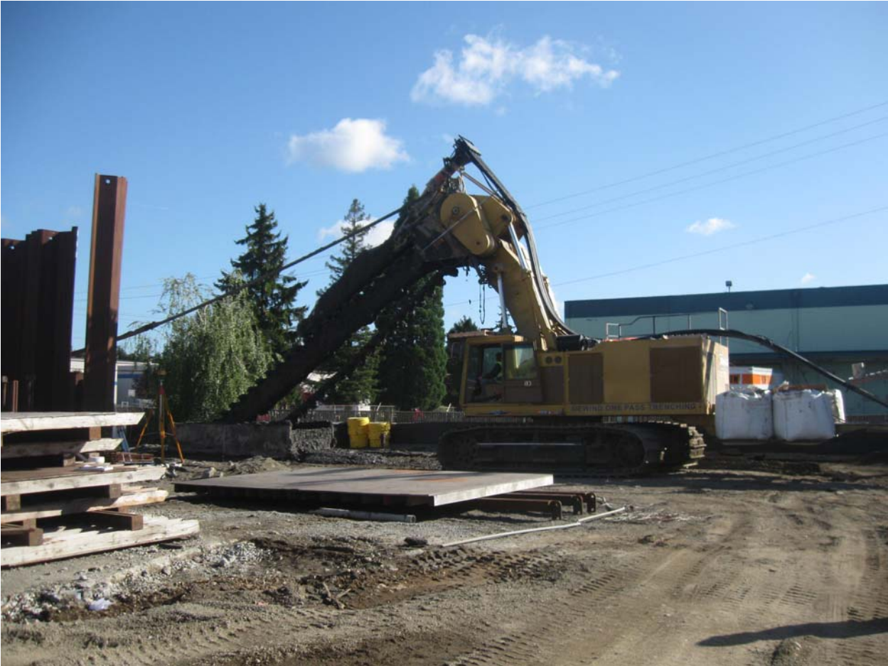
Mixing chain pulled out after machine breakdown.
