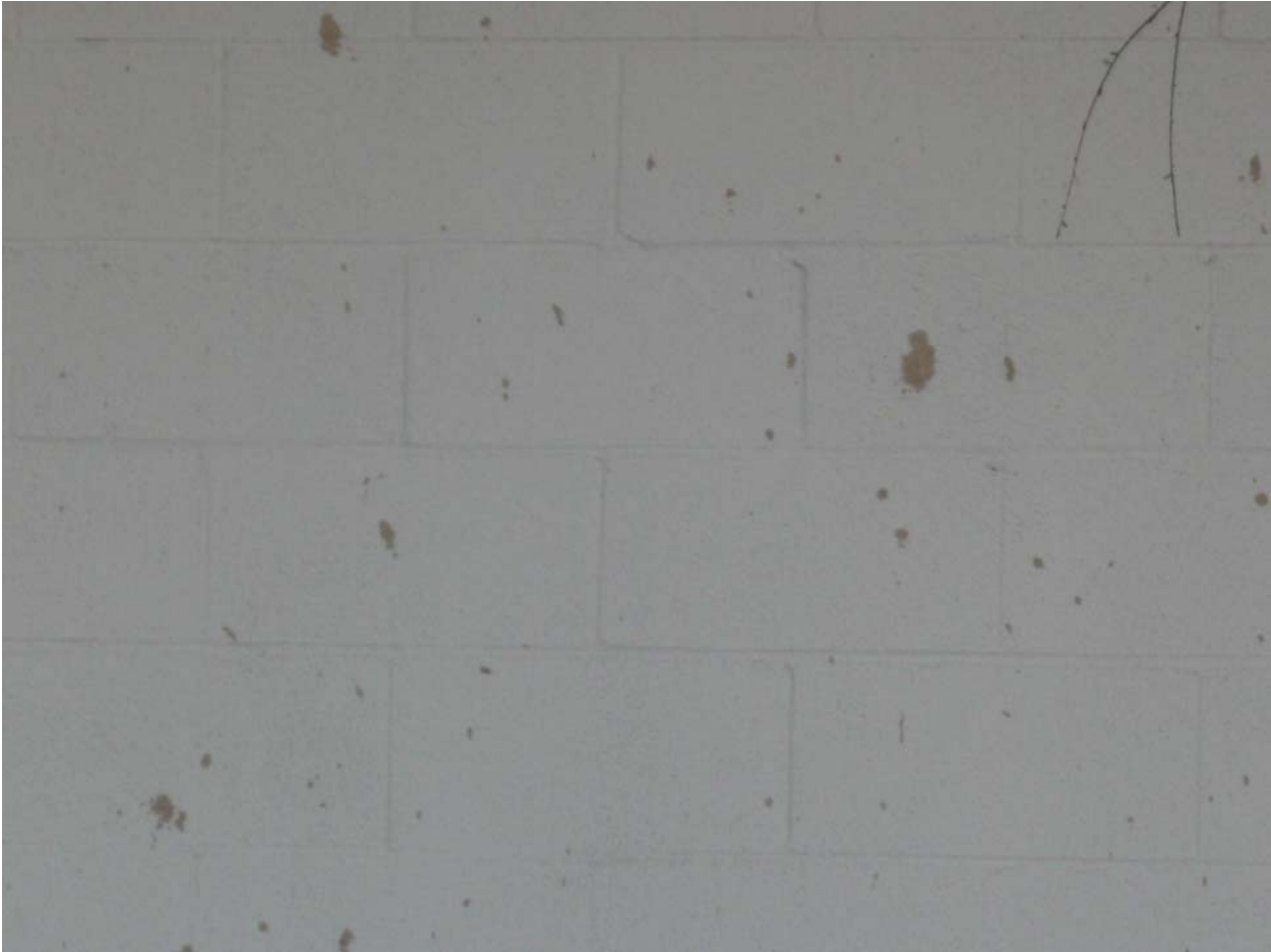
Slurry on building wall south of site.
