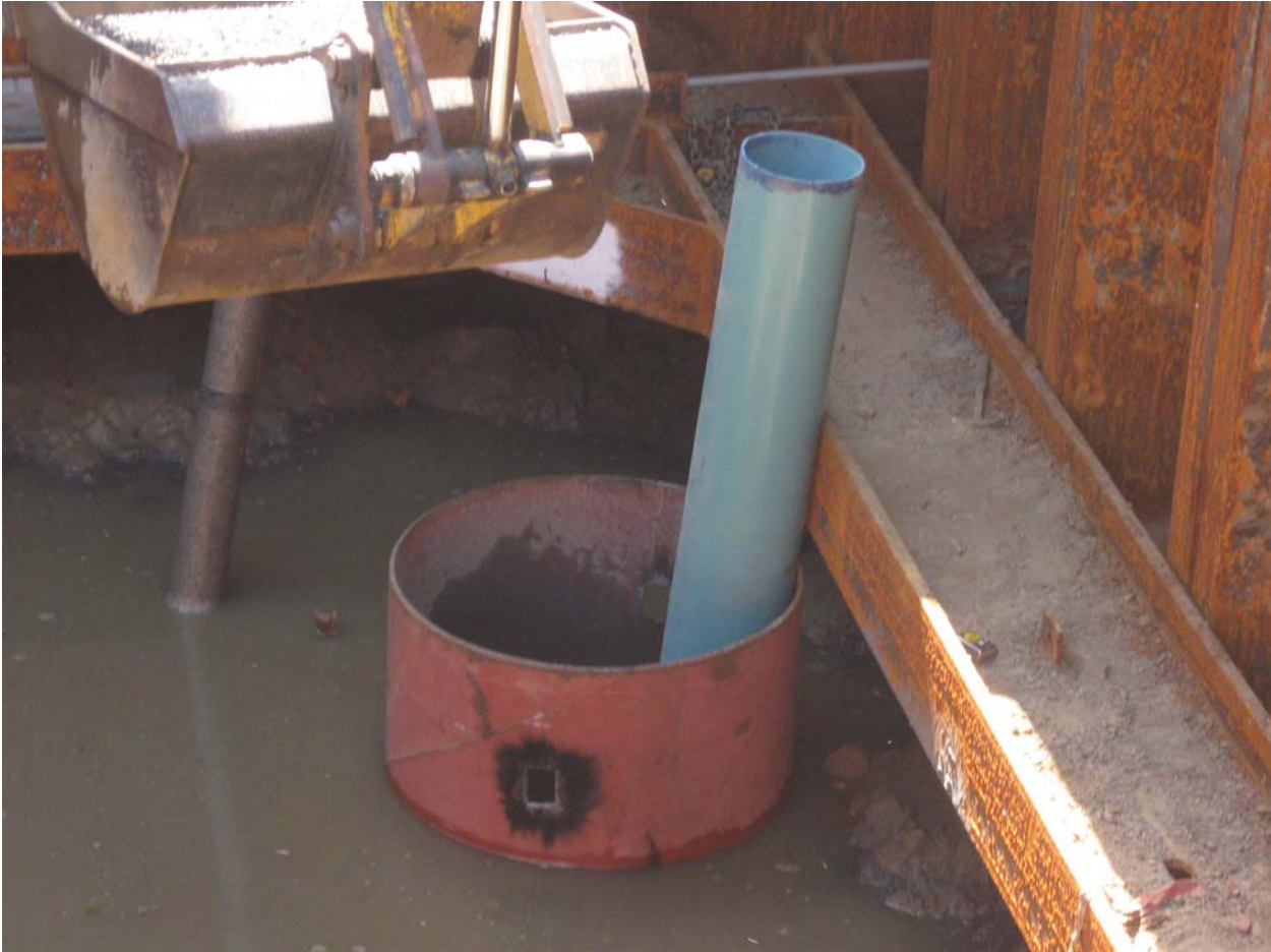
Setting PVC casing in steel casing with bottom of capped PVC casing set at elevation 6.0 feet.
