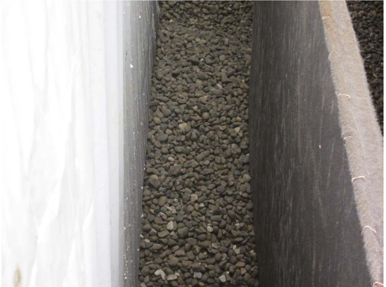
Gravel being placed on the west side of the vertical geotextile along the west wall of the vault. Geotextile hooked to a cable is shown to the left.
