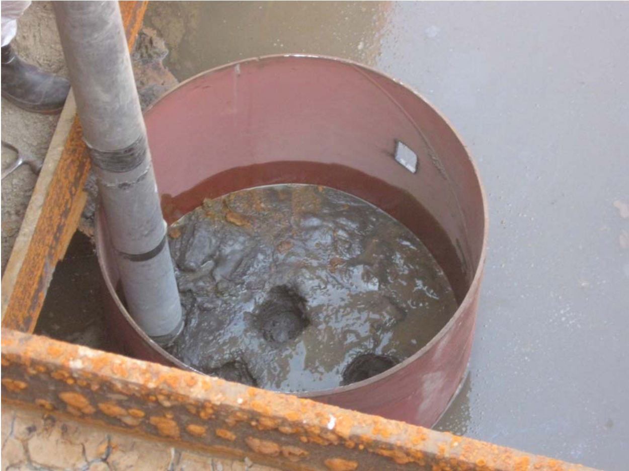
Vactoring soil from inside casing after it was pushed to a base elevation of 6 feet.
