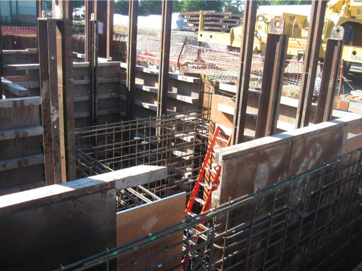
Progress on re-bar installation and form work at north end of vault.
