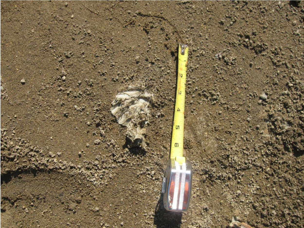
Slimy tan sludge coming up through liner at station 2+25.
