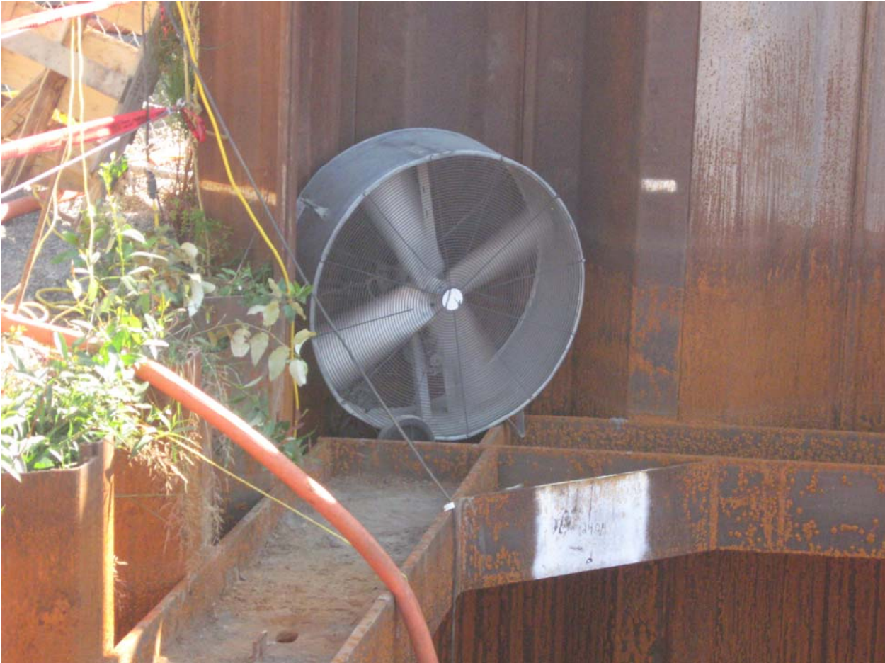
Fans installed to provide fresh air to excavation.
