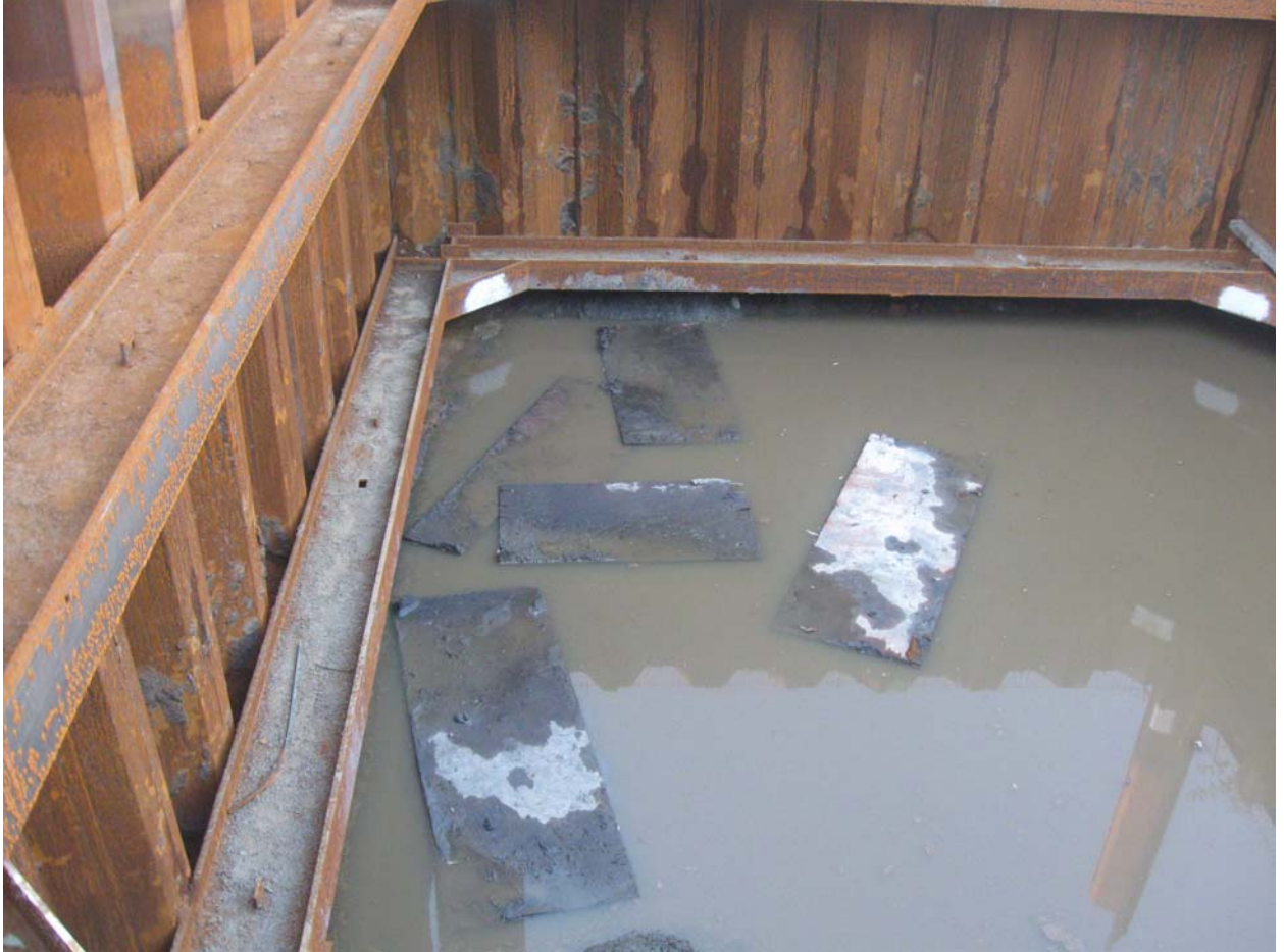
• Groundwater in excavation at elevation 11.4 feet.
