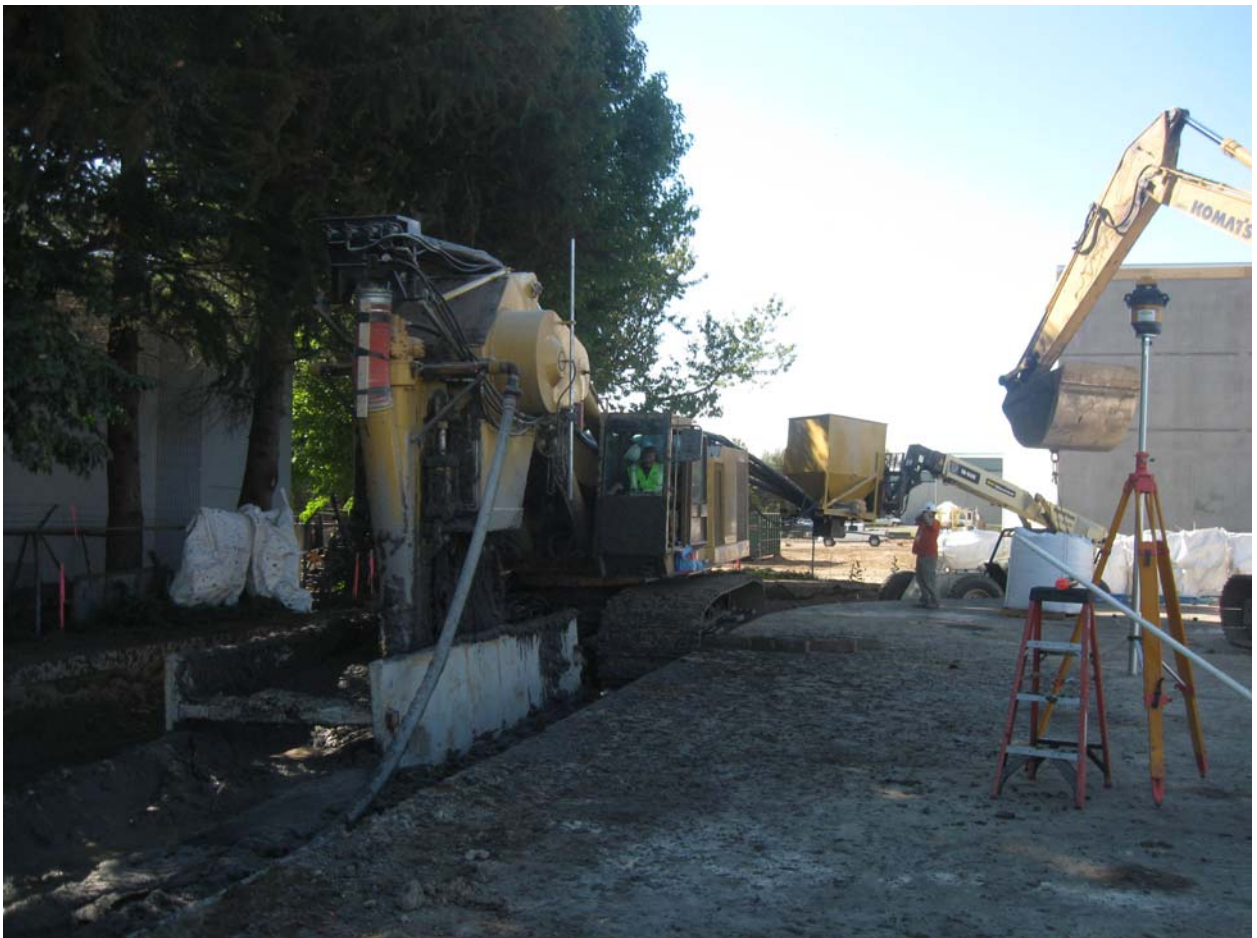
Bentonite feeder suspended on forklift to allow trencher to make the southwest corner.
