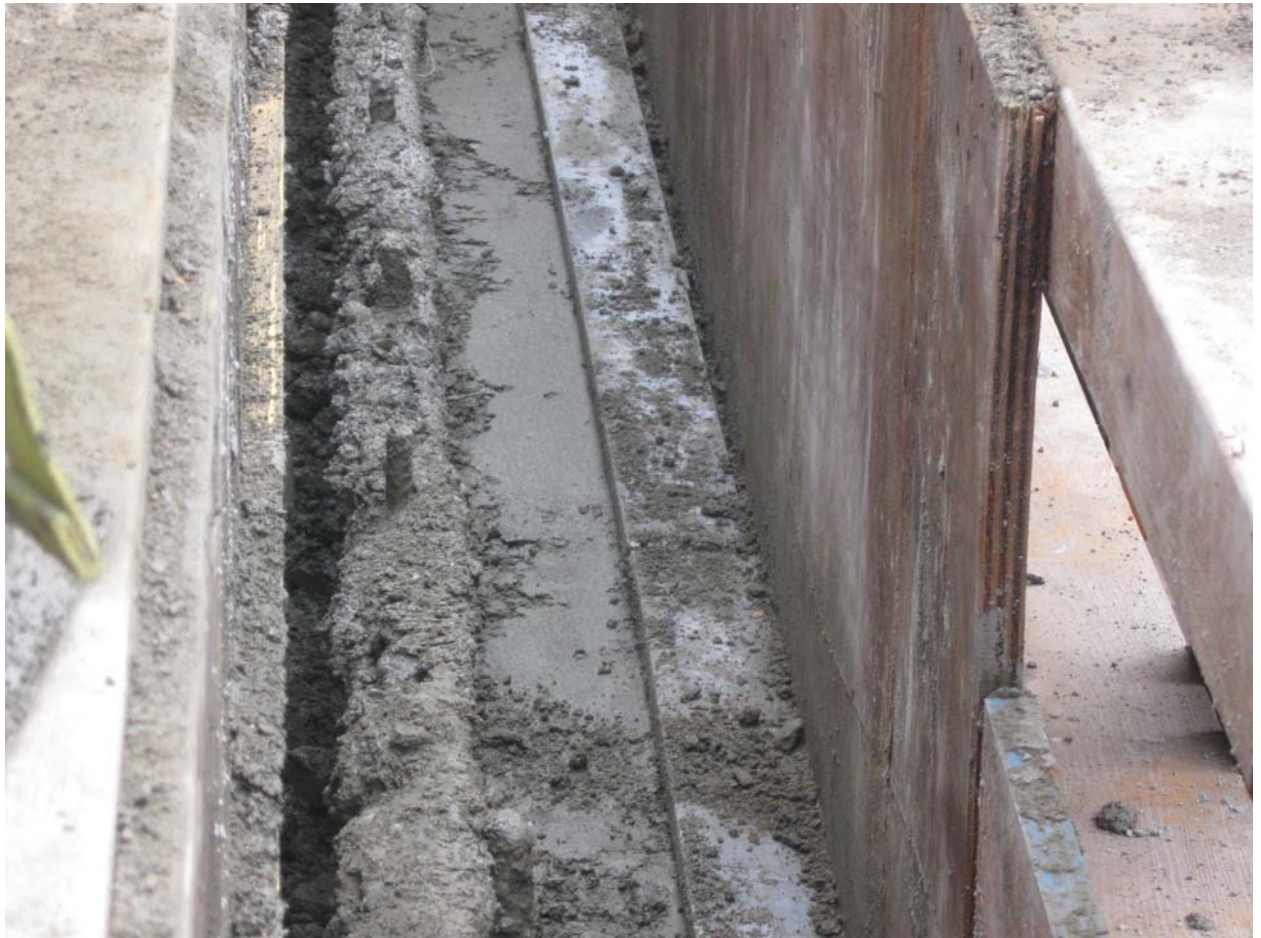
Float finish next to an embedded Nelson Stud on the east wall, prior to removing concrete from re-bar that will be cast inside the 4 ½-inch wall.
