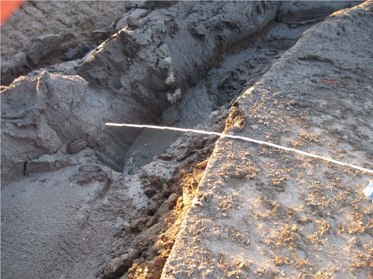
Centerline of trench at mid-point of southwest corner only 4 feet from edge of asphalt cut at station 1+75.
