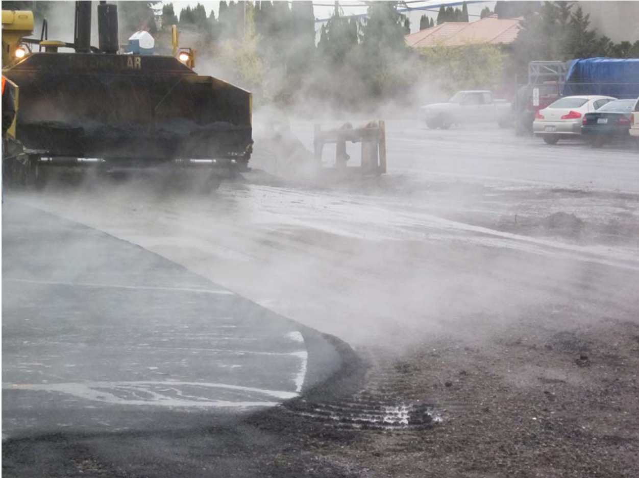
Paving in rain with surface water running across stable aggregate near new site entrance.
