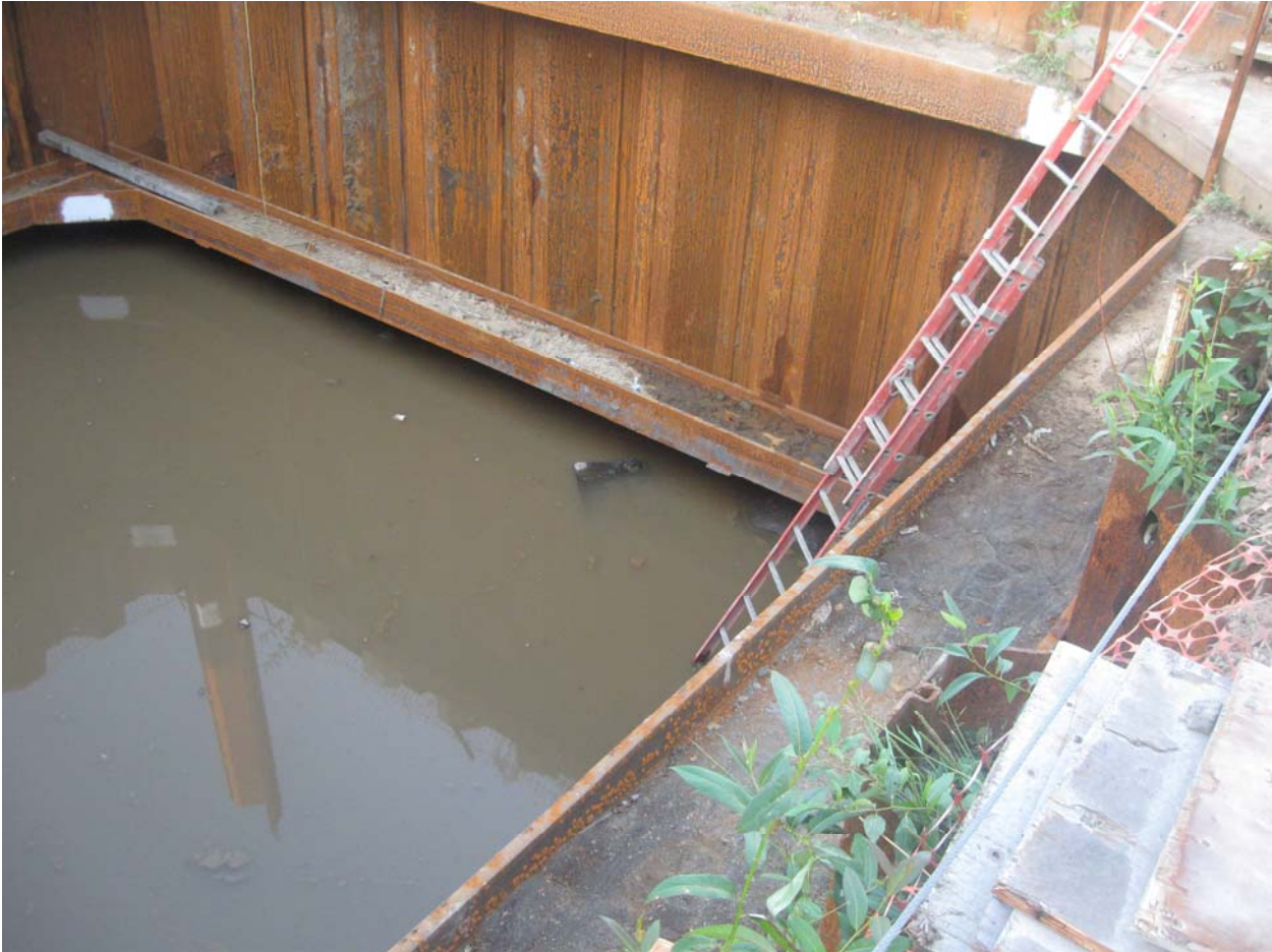
Groundwater in excavation.
