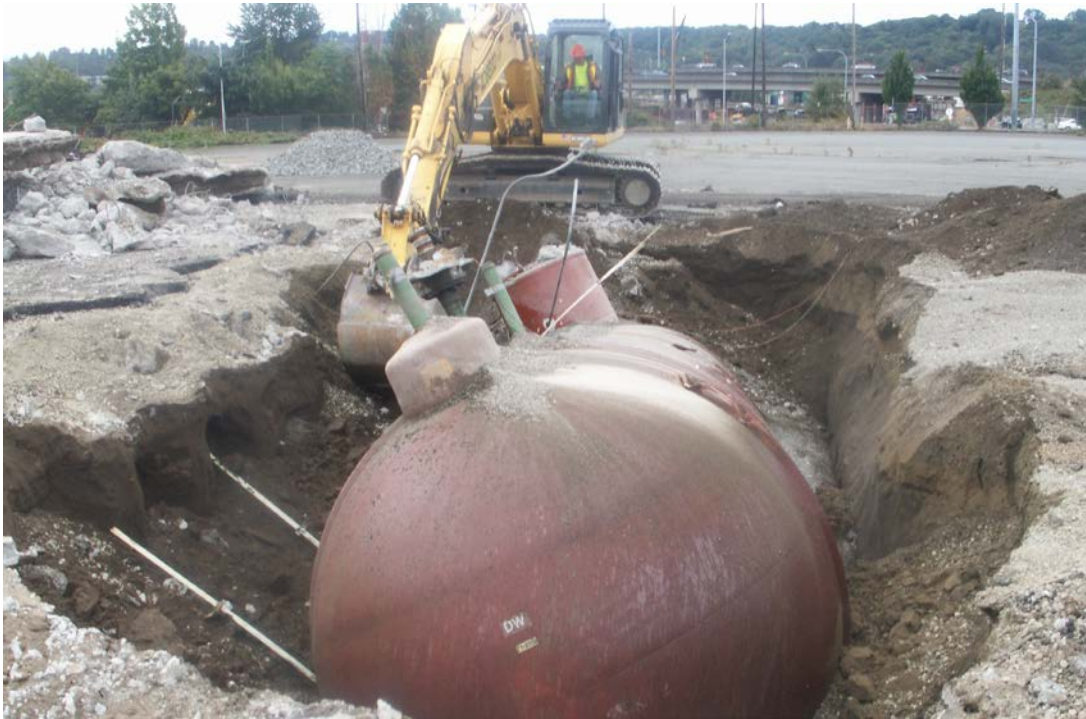
Photograph 3: Uncovered UST floating on groundwater following removal of hold-down straps, looking west.
