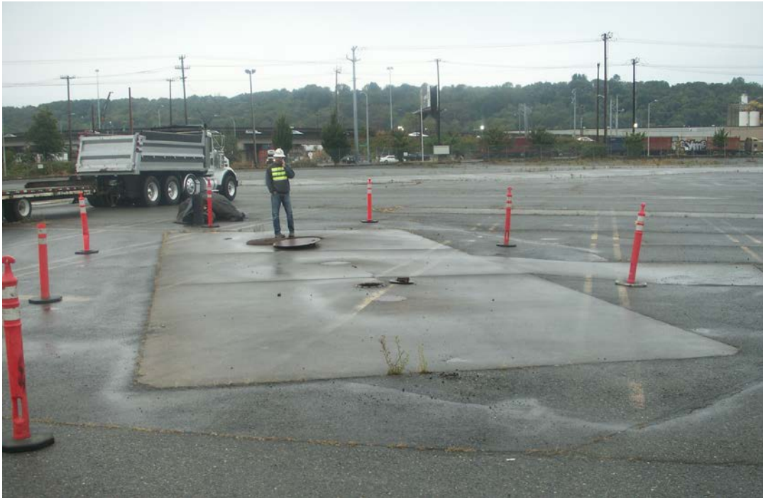
Photograph 1: Concrete pad overlying the underground storage tank (UST) prior to start of excavation, looking west.
