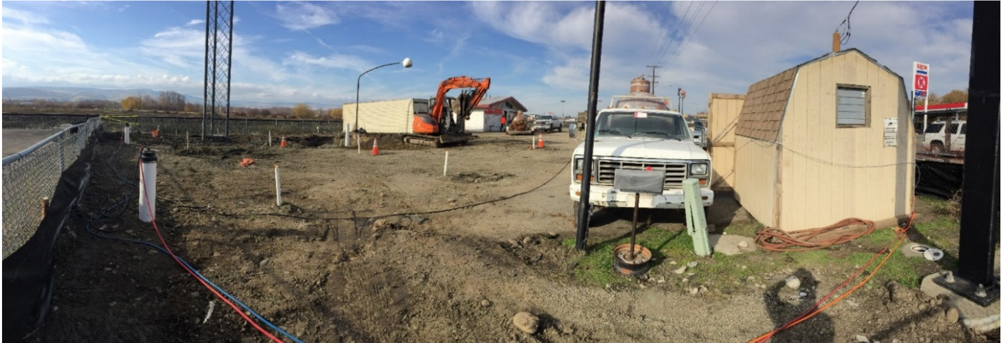
Photograph 11. Trench recovery system, sumps, 1,000-gallon holding tank, and compressor shed.
