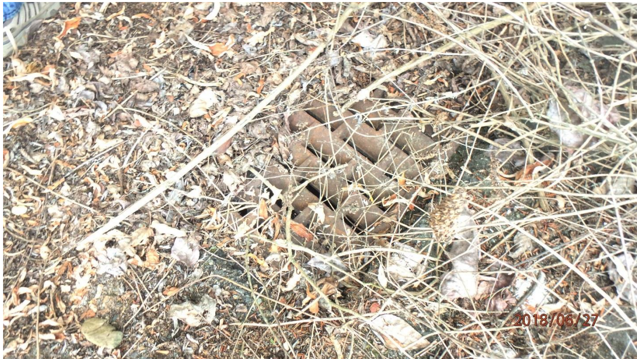
Photo 11. Organic debris obstructing catch basin near southeast corner of consolidated landfill: RA-3
