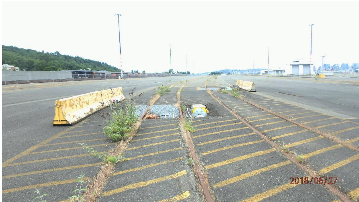
Photo 1. Vegetation growth along rail tracks: RA-2 and RA-3
