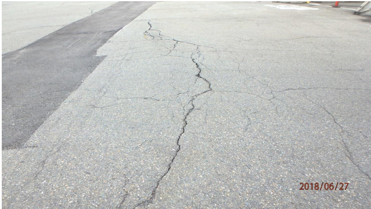
Photo 9. Another view of elongated mound in pavement with cracks: RA-2 (map note 5)
