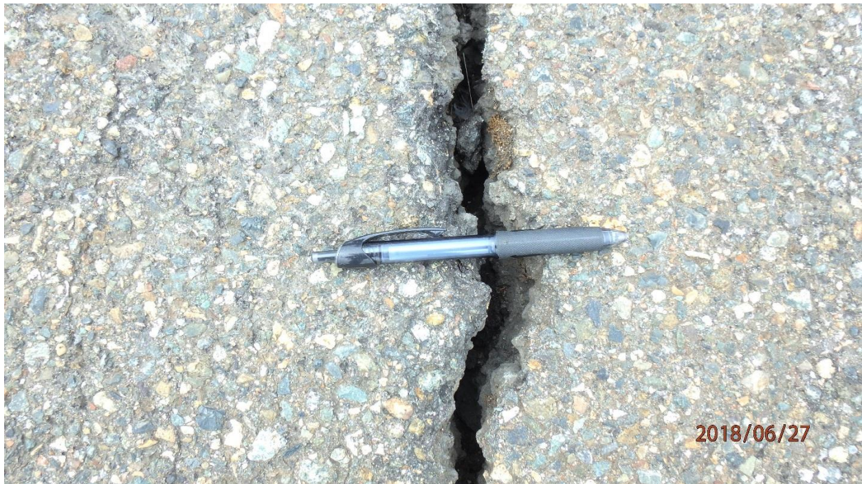
Photo 10. Close up of elongated mound in pavement with cracks as wide as 1 in.: RA-2 (map note 5)
