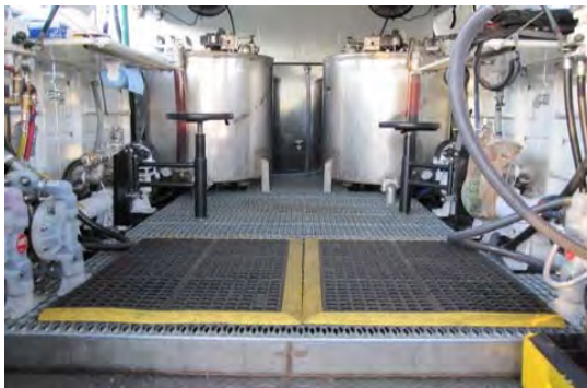
5. Injection Rig Interior
