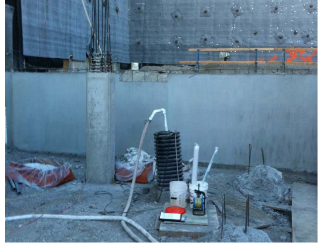
Photograph 20. Taken May 10, 2016, looking northeast. Set up prior to collecting groundwater sample from dewatering well DW05.
