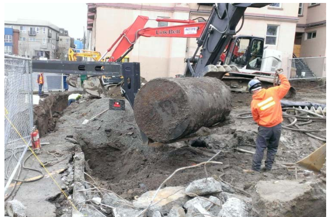
Photograph 6. Taken January 19, 2016, looking north. Removal of UST02 along west side of Property.
