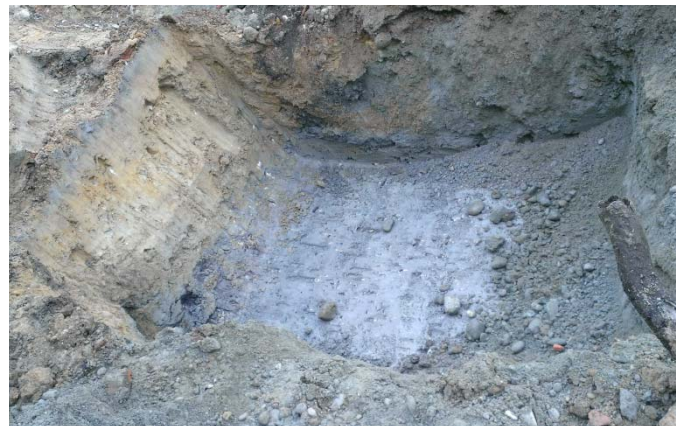
Photograph 4. Taken January 8, 2016, looking south in the vicinity of UST01. Note the boundary between non-impacted soil and stained PCS.
