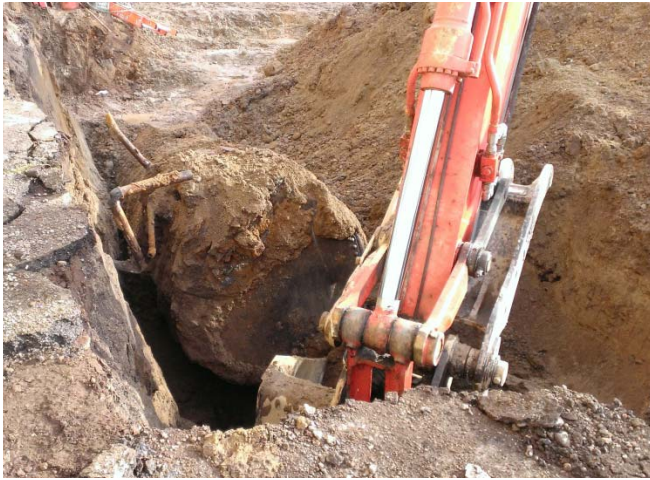
Photograph 7. Taken January 20, 2016, looking east. Removal of UST03. Note product lines connecting UST03 to apartment building to the north.
