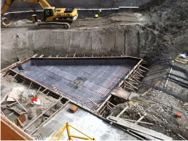
Photograph 19. Taken April 15, 2016, looking southeast. Total depth of excavation has been reached in center of Property. Footing installation in progress.
