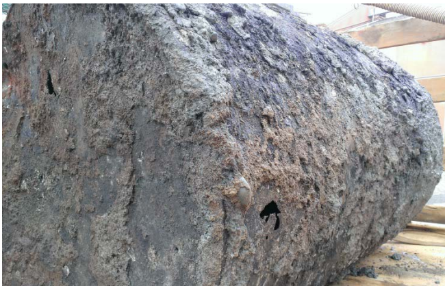
Photograph 3. Taken January 8, 2016. UST01 removed and placed on trailer for disposal off site. Note holes in tank walls.
