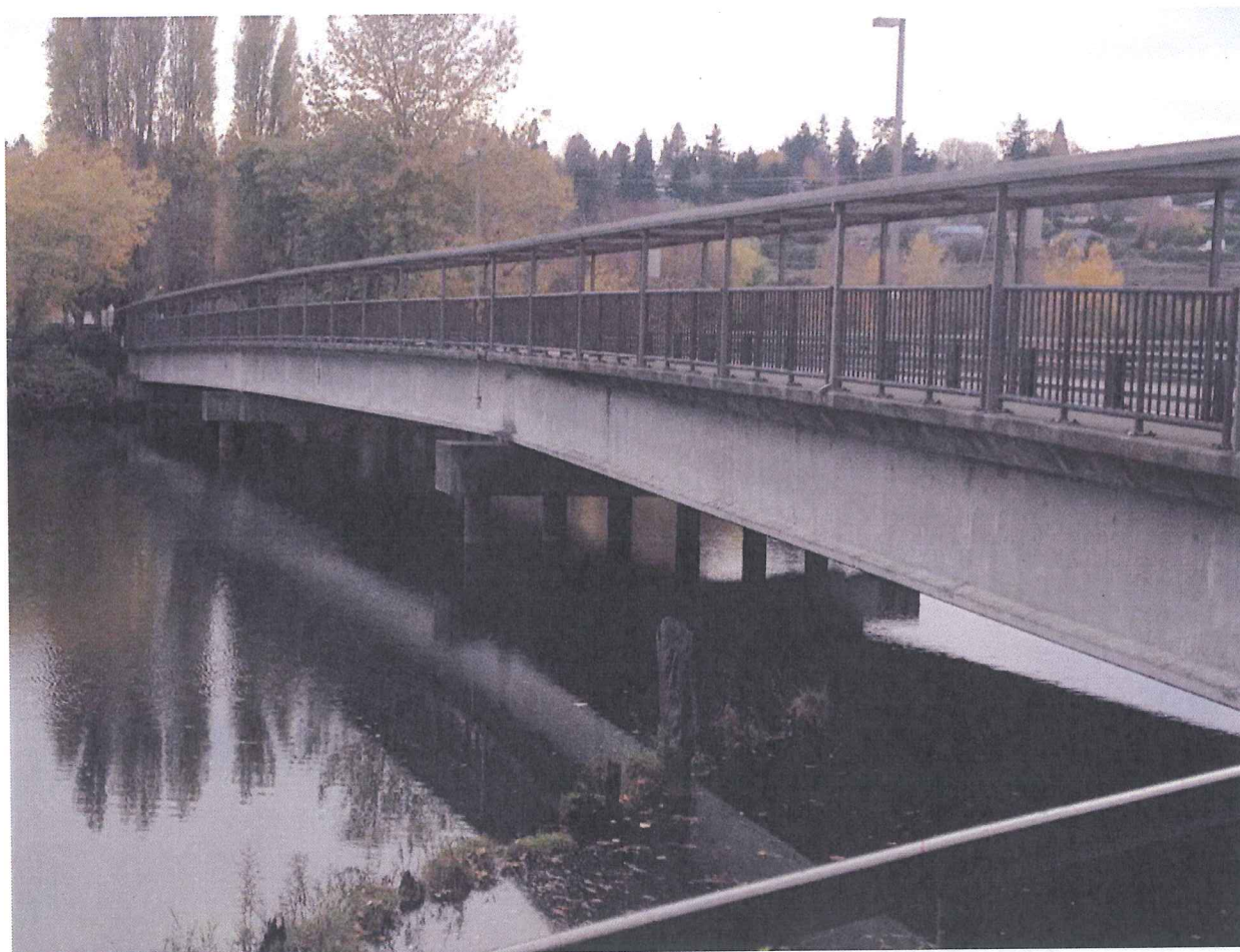
Figure 2. Photo of the downstream station - the pedestrian bridge at the Boeing Development Center- located at River Mile 5.0.
