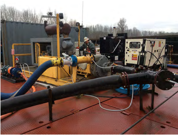
Diesel-powered centrifugal pump.
