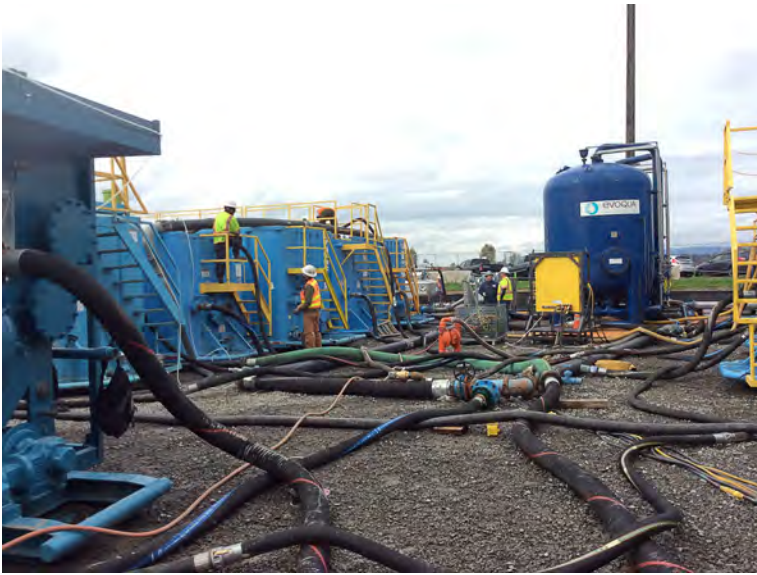
Water treatment setup in MHA.
