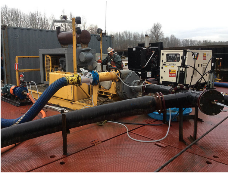
Diesel-powered centrifugal pump.
