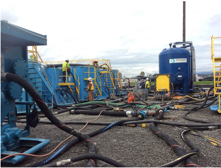
Water treatment setup in MHA.
