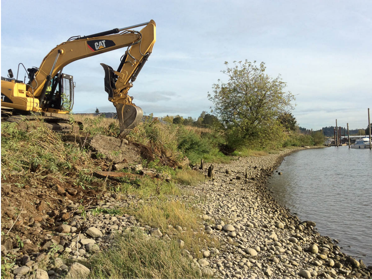
Debris removal along shoreline south of Division Street.
