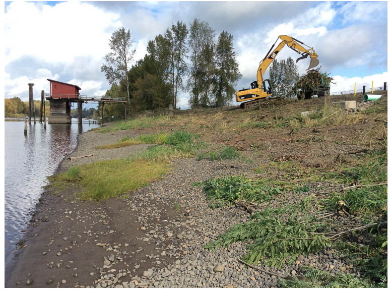
Excavator loading vegetation removed from the shoreline to the track truck, which transfers it to the MHA.
