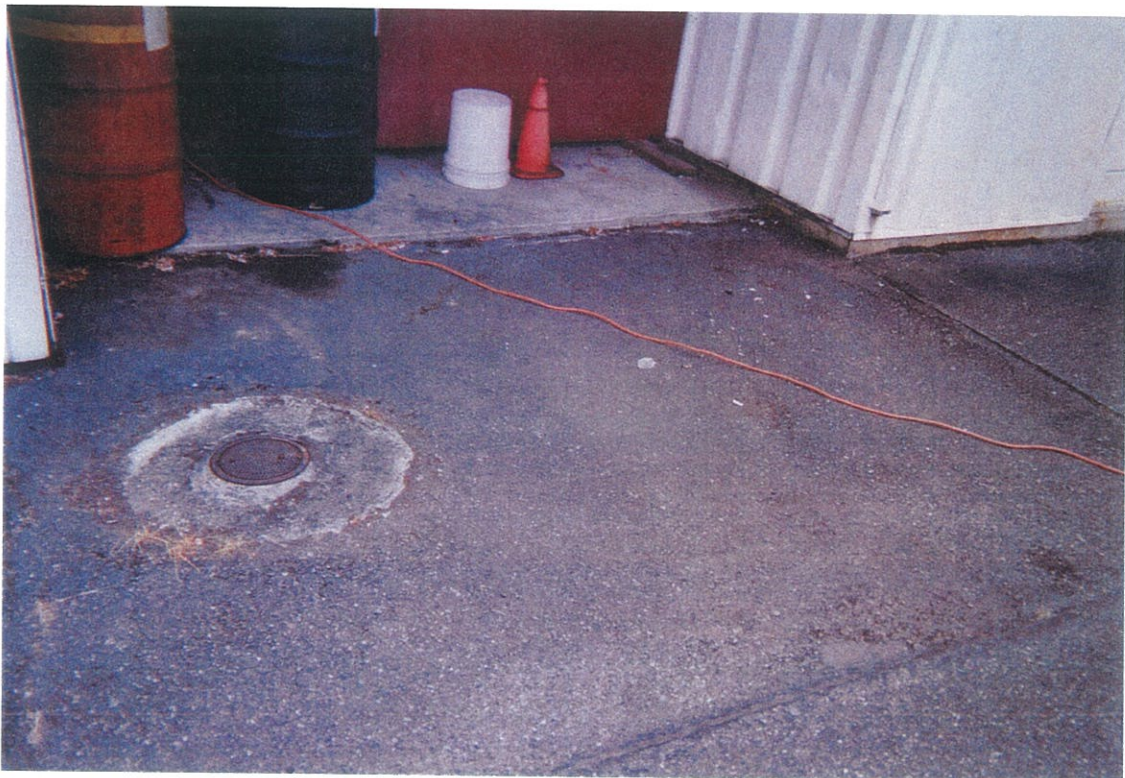
1989 WASTE OIL TANK EXCAVATION AREA AND CURRENT WASTE OIL ABOVEGROUND STORAGE TANK
