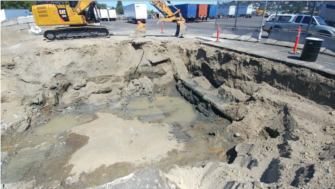
Excavation at conclusion of excavation, with view looking NNE. North-south oriented sewer line is visible on right side of excavation. A steel or iron pipe with a capped end is visible in the NE corner of the excavation; that pipe is of unknown origin and connection. July 16, 2018.
