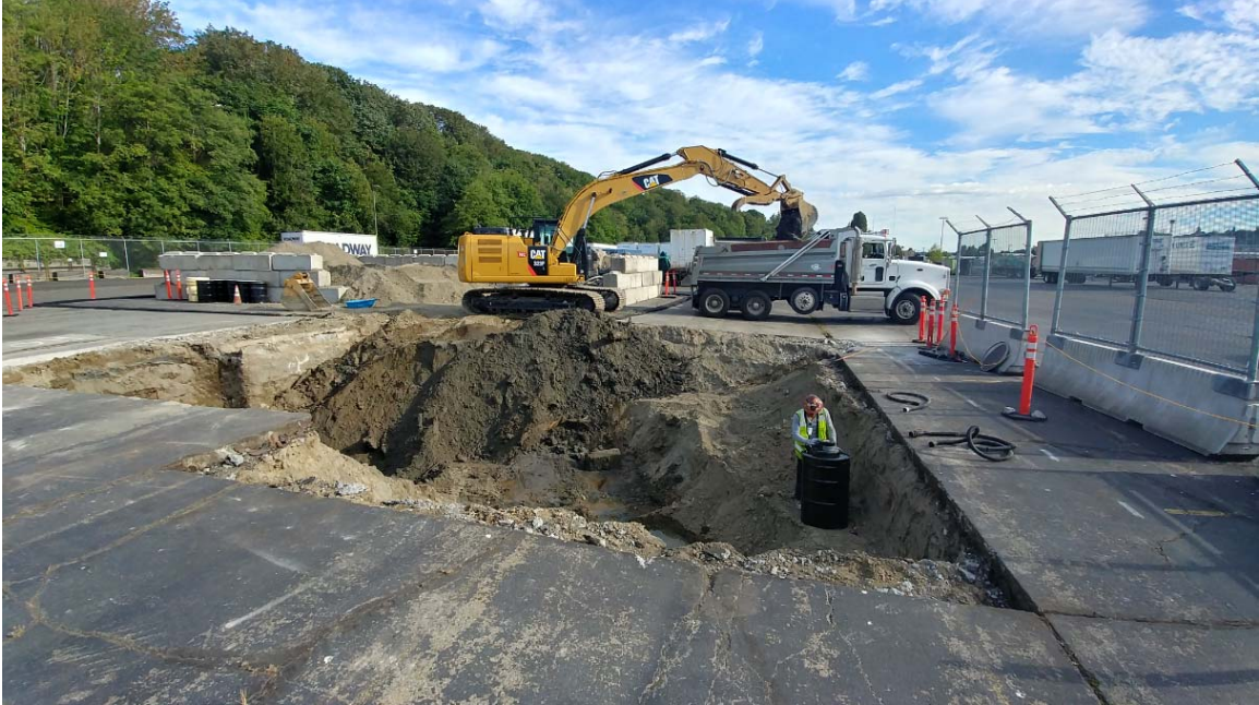
Direct-loading impacted soils into truck for disposal. The western concrete hydraulic lift trough is visible at the left (west) side of the excavation. July 6, 2018.
