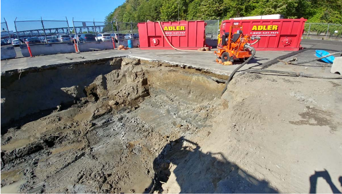
View to the SW showing clean western edge of excavation, dewatering pump, and discharge tanks. July 13, 2018.
