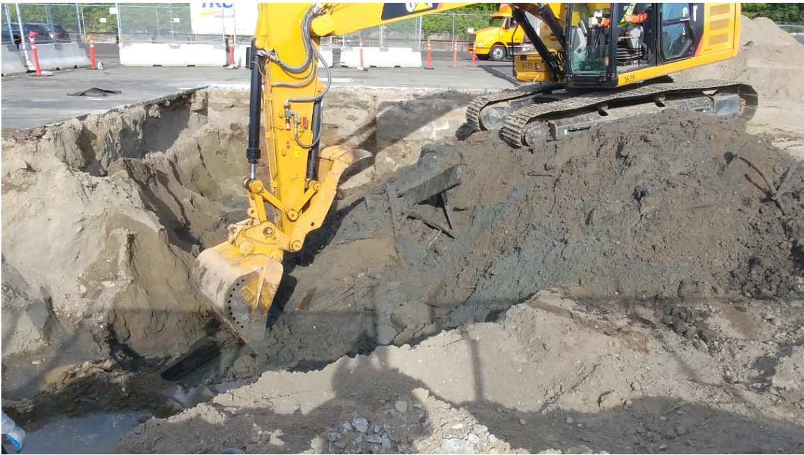
Removing impacted soils. Wooden boards formerly part of the wooden trough are visible just below the excavator bucket. July 6, 2018.
