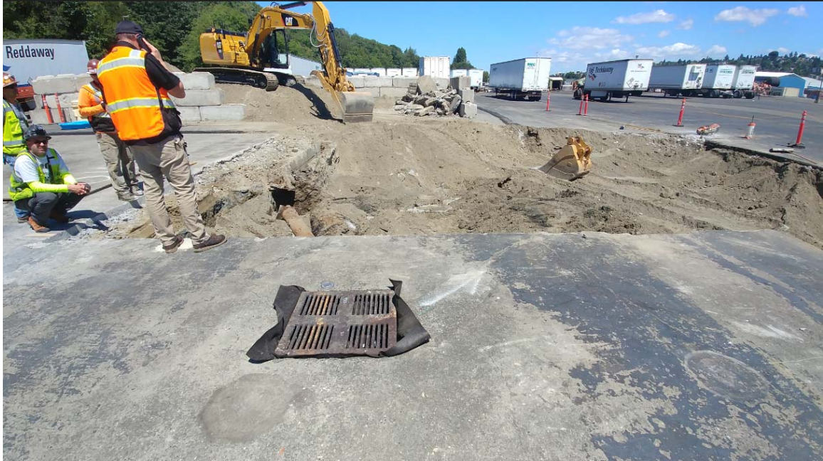
Stockpiling clean overburden to the northwest of the excavation. West hydraulic lift trough is still in place on left side of excavation. The east trough has been broken up and removed. July 3, 2018.
