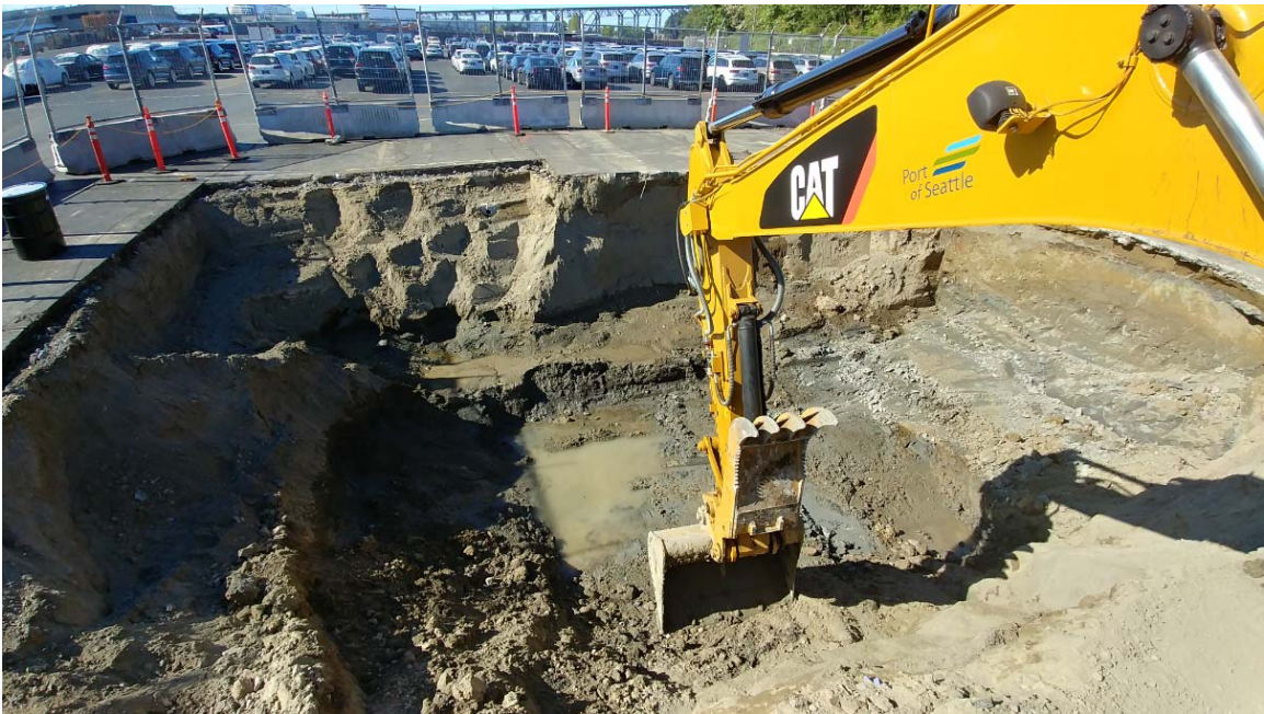
Nearing the completion of excavation with view to south. The capillary zone and slow groundwater seepage into the excavation are visible on the south wall of the excavation. July 13, 2016.
