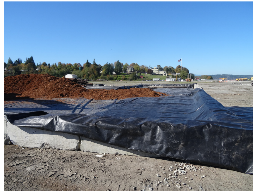
Lined eco-block containment for creosote processing
