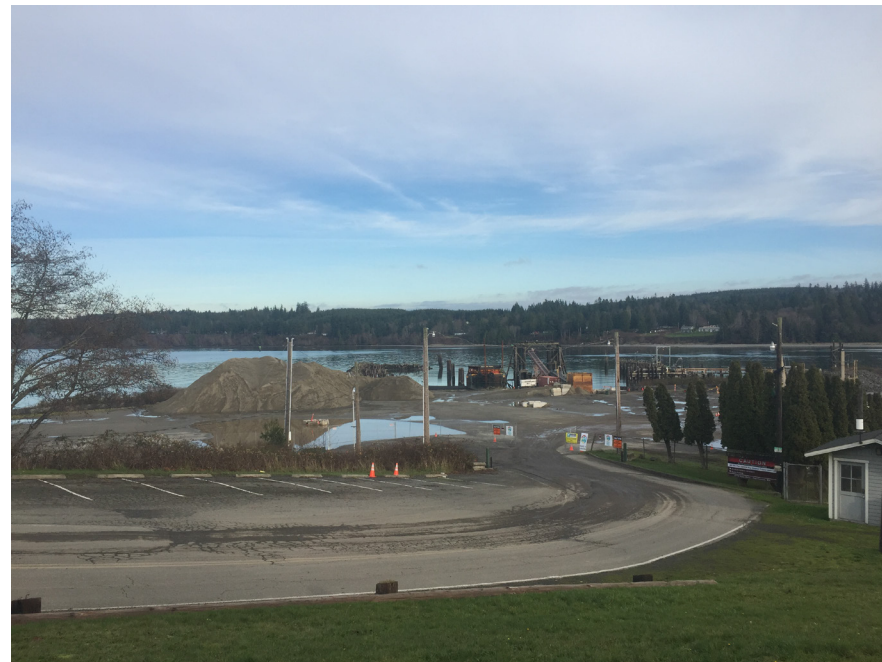
Subtidal cap, EMNR, and RMC sand material stockpile and barge loading conveyor
