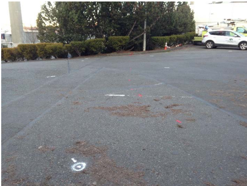
View of utility locate, B-01 location in foreground, looking to the north.
