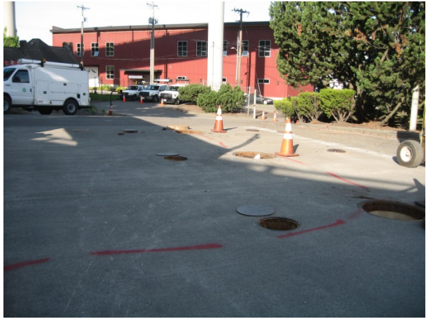
Tank Location and Risers
