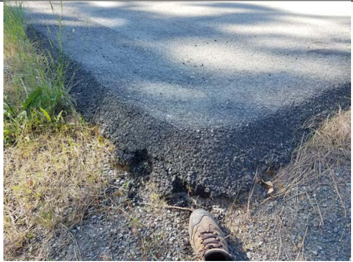
Photo 3: Subbase exposed in northeastern corner of cap (pre-crack fill).
