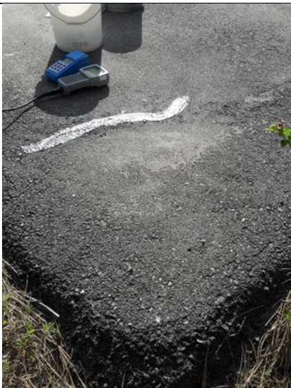
Photo 11: View looking northeast in northeast corner of cap (post-crack fill).
