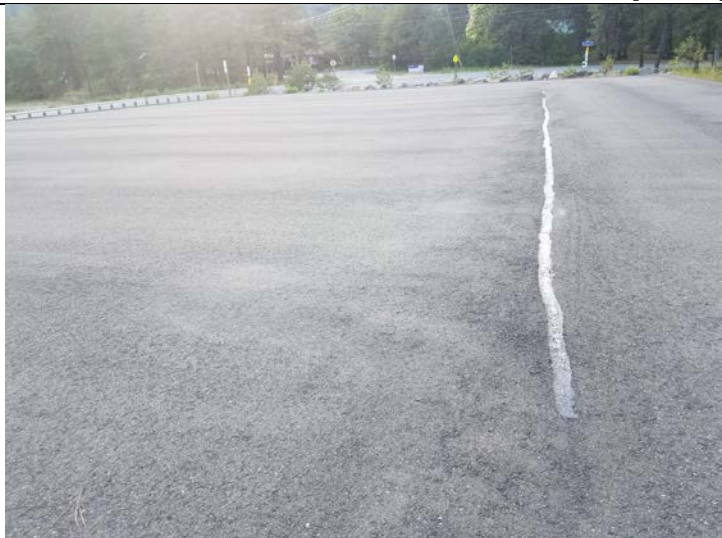
Photo 9: North-South trending crack in cap approximately 85 feet in length (post-crack fill).
