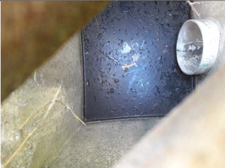
Photo 6: View inside catch basin located on asphalt cap, water not observed to be flowing into the grit chamber.
