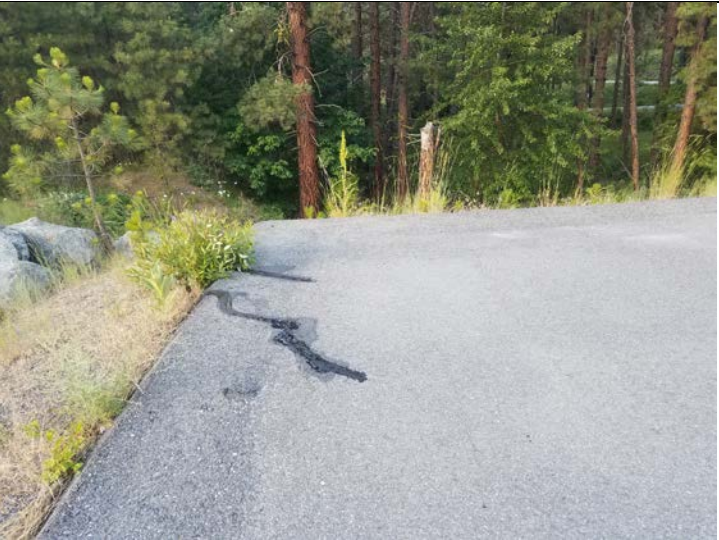
Photo 4: View looking east toward northeastern corner of cap. Cracks developing and elongating as a result of root expansion (post-crack fill).
