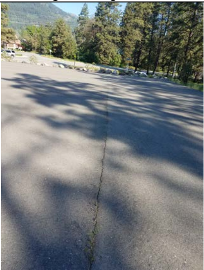
Photo 8: North-South trending crack in cap approximately 85 feet in length (pre-crack fill).
