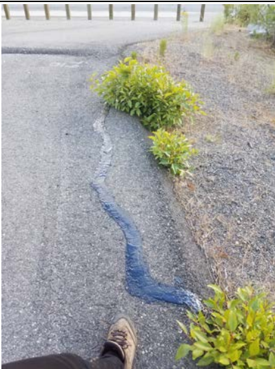
Photo 5: View looking west of crack ~9 feet long along northern edge of cap (post-crack fill).
