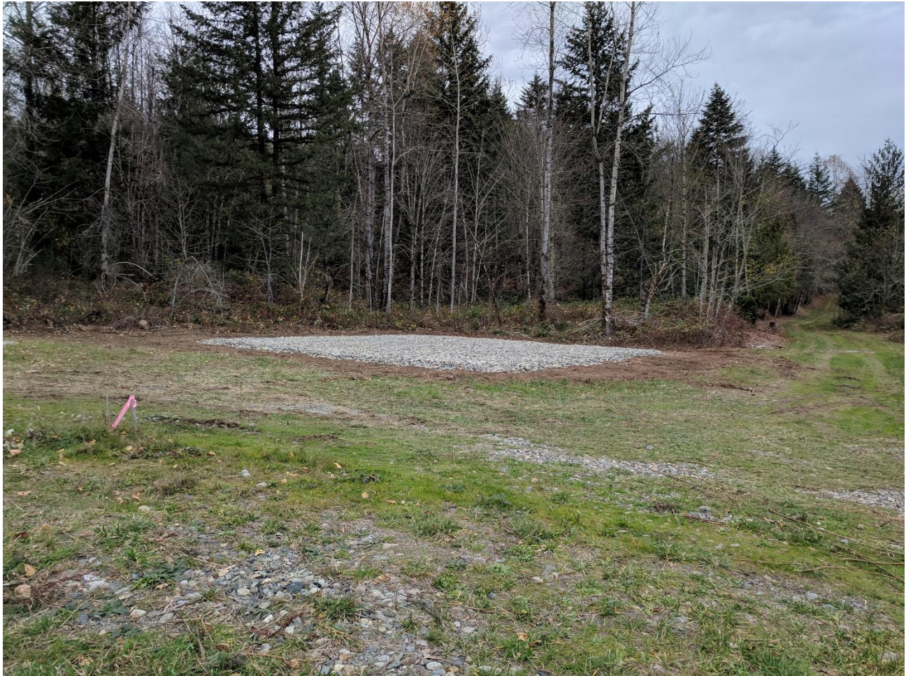
Photo 6 – View of south contingency treatment area that was cleared and rock pad placed.
