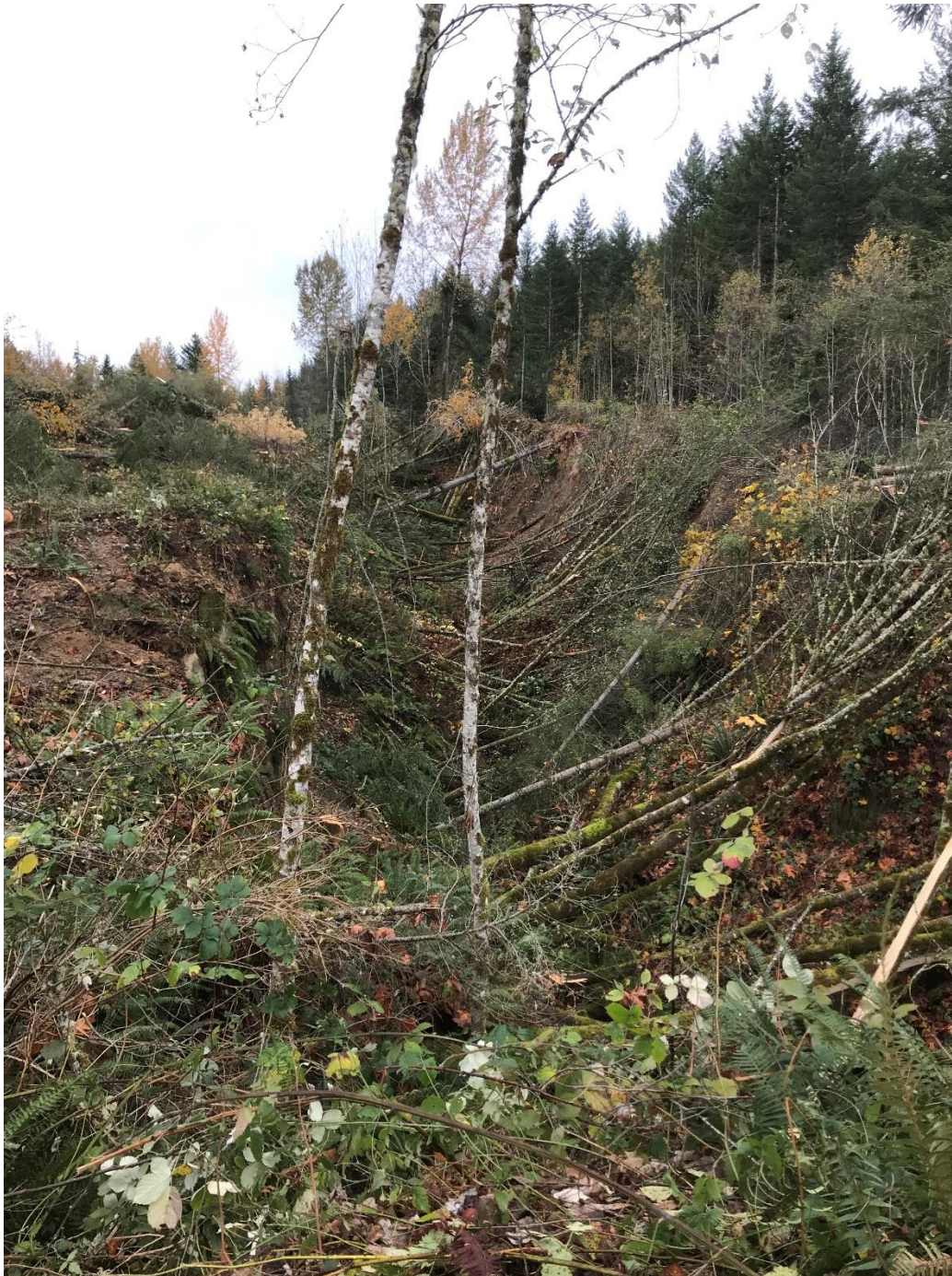
Photo 2 – Cut trees within trench, felled to lie against trench side-walls to allow removal with tree picker.
