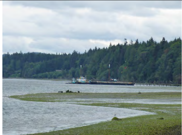
Comment: Removing piles with vibratory hammer in SMA-5, viewed from shoreline of project site.
