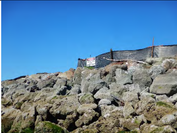
Comment: "Danger Keep Out" sign installed on silt fence at the Eastern Wharf area
