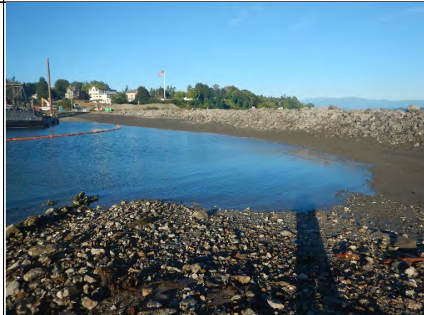
Comment: SMA-1 jetty after concrete and piling removal and rip rap replacement
