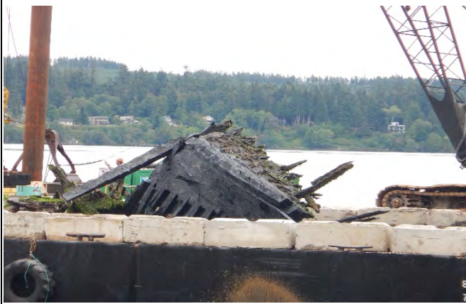
Comment: Large portion of the derelict vessel removed from FLTF and placed on material barge
