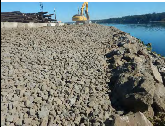
Comment: Placement of Type 1 armor on upper portion of Eastern Wharf bank
