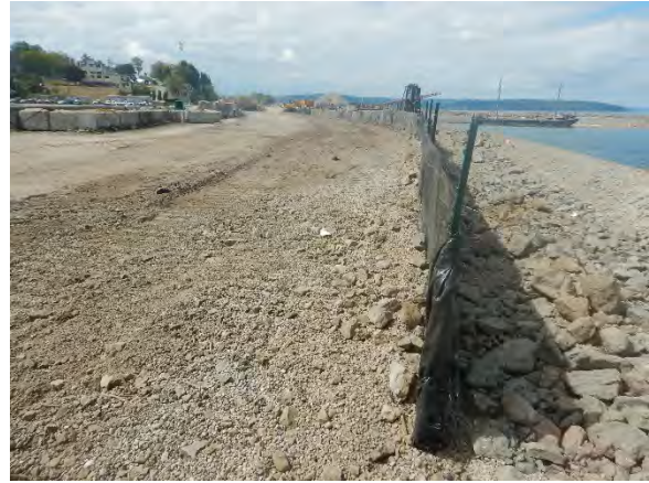
Comment: Silt fence installed at the south end of SMA-1 along top of bank
