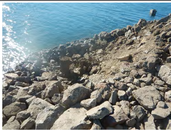
Comment: Piles in upper portion of Eastern Wharf (south end) exposed for extraction
