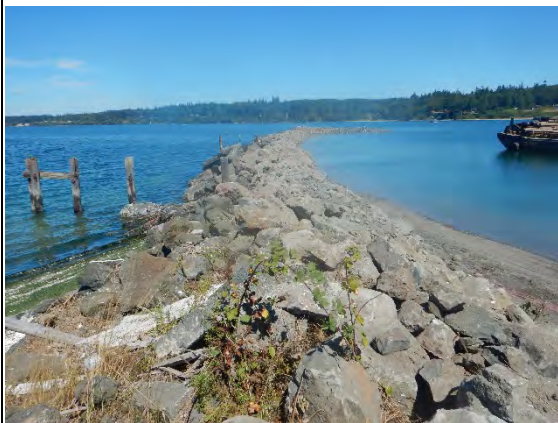
Comment: SMA-1 jetty after completion of piling removal, concrete removal, and rip rap placement
