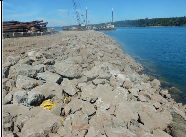
Comment: Placement of rip rap over Type 1 armor on upper portion of Eastern Wharf bank
