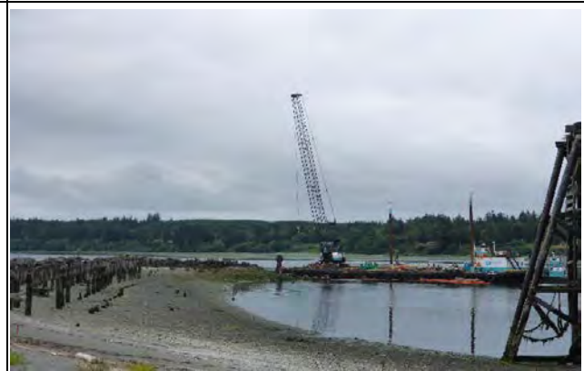
Comment: Removing piles during low tide with vibratory hammer at Station 34+00 (SMA-1 Jetty area)
