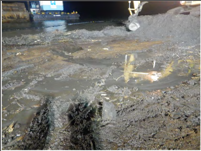
Comment: Upland excavation in SMA-2 bank, adjacent to former Pier 4 area at approximately 0 MLLW
