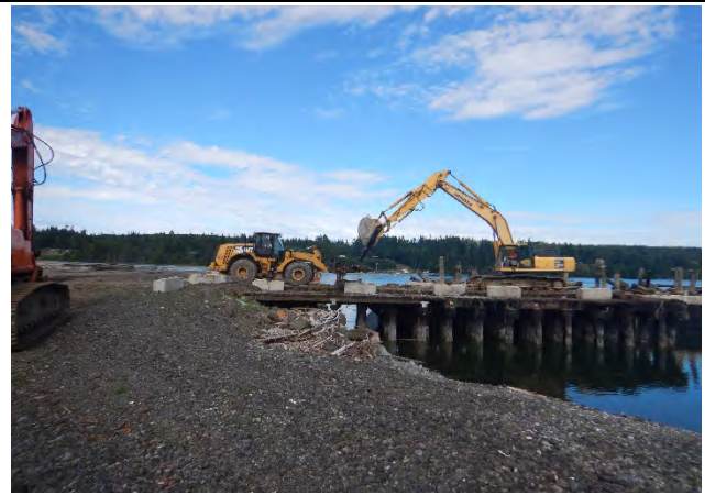
Comment: Transferring pilings from material barge to upland containment and processing area
