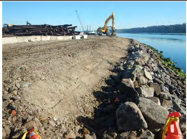
Comment: Removal of asphalt and concrete from upper portion of Eastern Wharf bank
