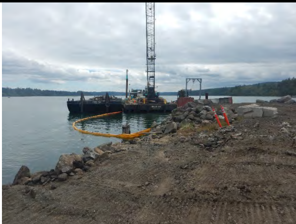
Comment: Pulling pilings from south end of Eastern Wharf with diver assistance
