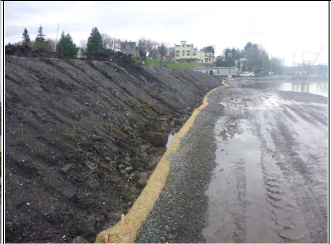
Comment: Wattle and filter material installed along northern edge of containment berm
